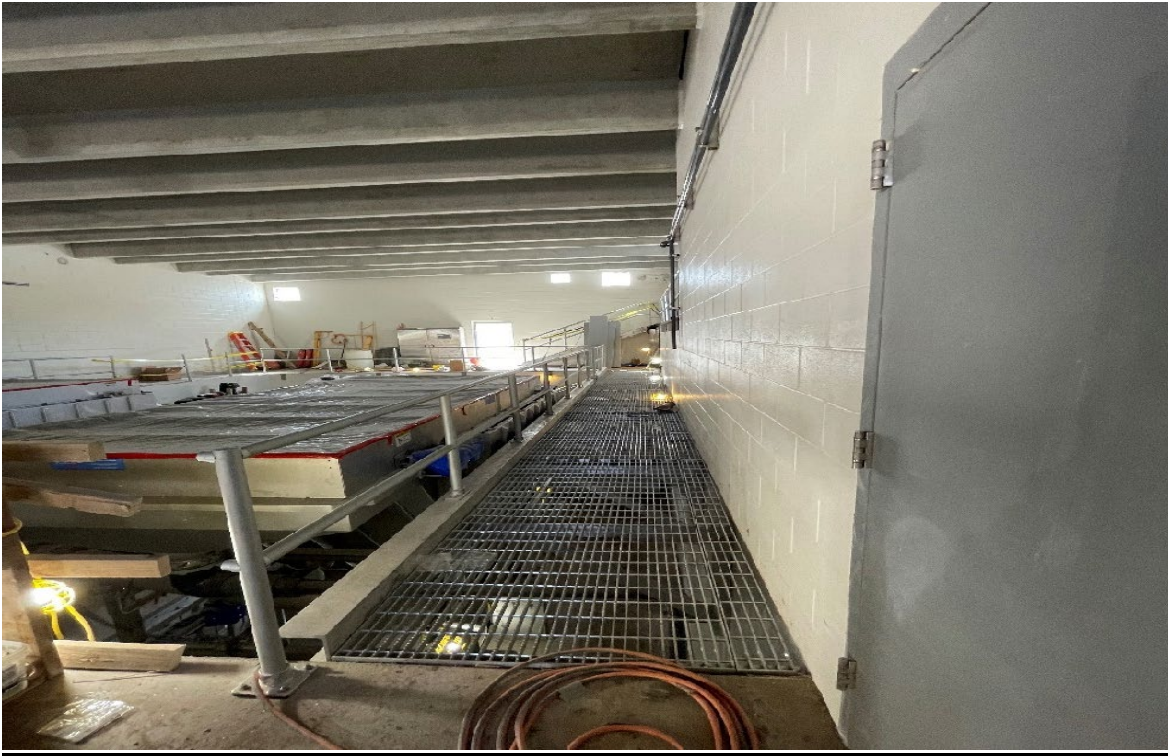
Grating catwalk with handrail installed adjacent to DAF tank.
