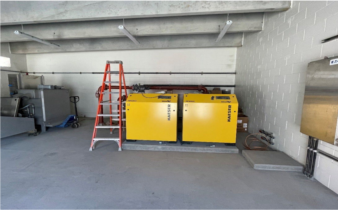
Digester blowers installed with associated piping and valves.
