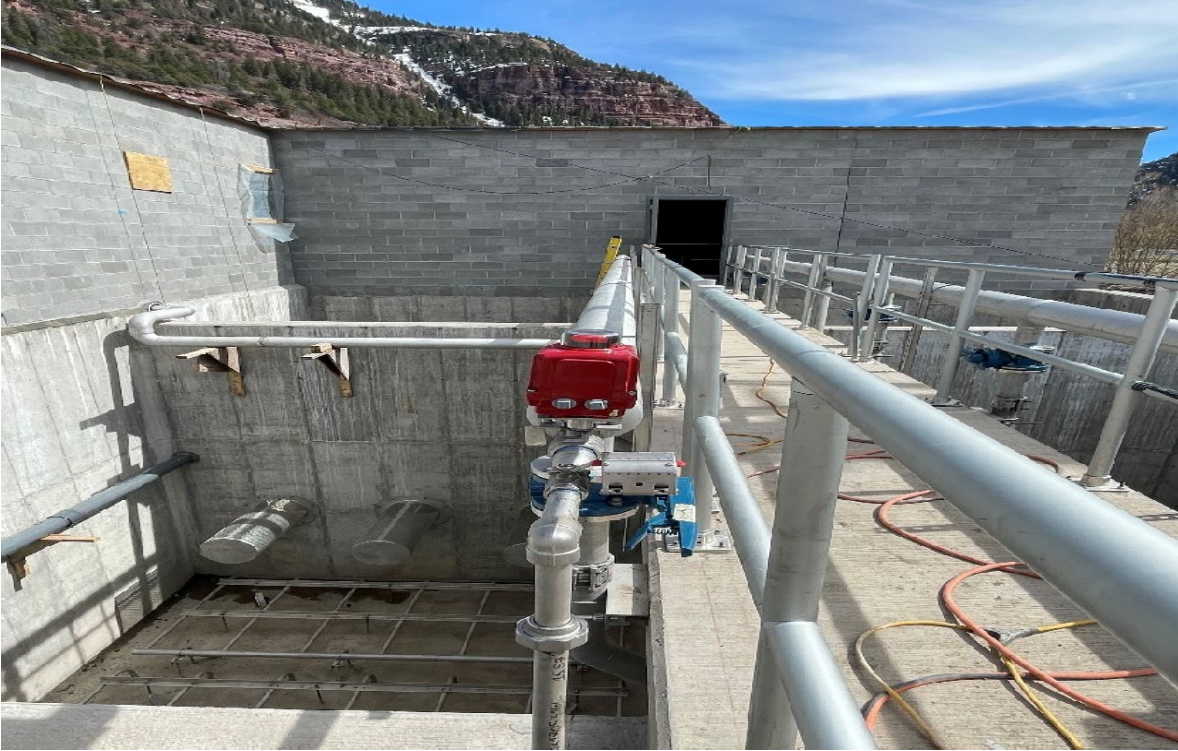
MBBR train #2 from above the pre- anoxic zone
