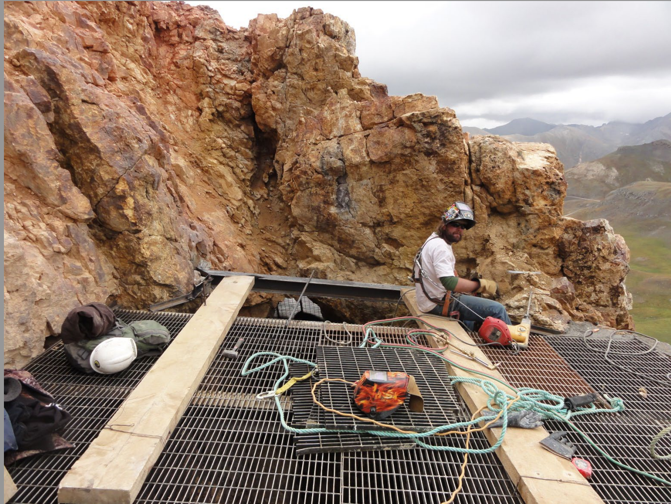
Contractors working with rope/harness installing a grated shaft closure. The work is very physical and dangerous in remote, sometimes high elevation areas
