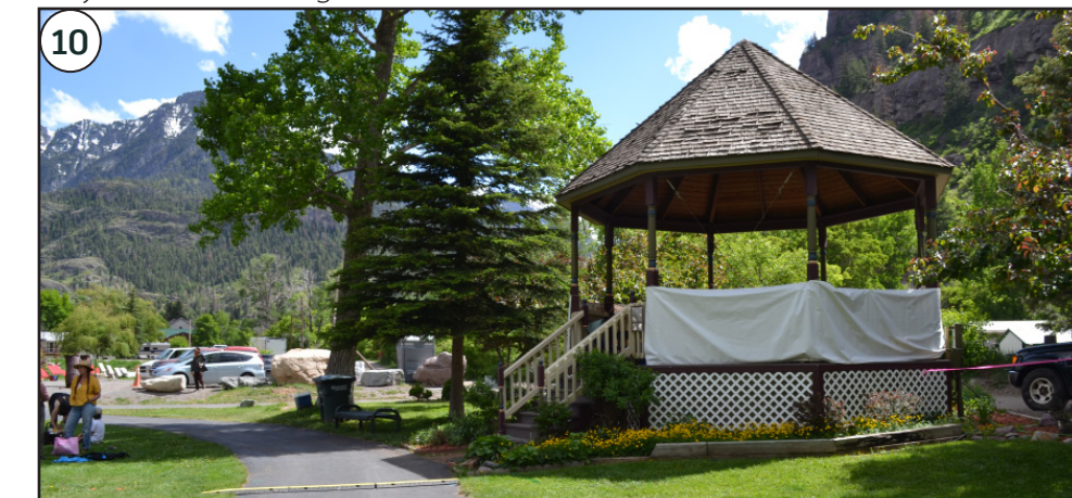
10 Existing Gazebo Analysis: Stringers beneath structure are deteriorating and in poor condition, creating safety concerns.
