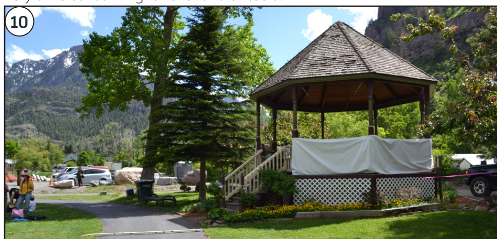
10 Existing Gazebo Analysis: Stringers beneath structure are deteriorating and in poor condition, creating safety concerns.
