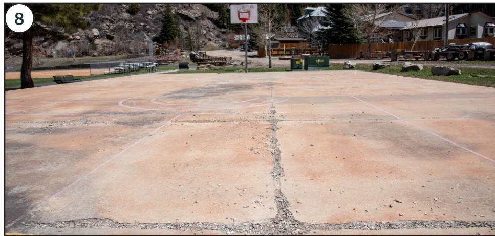
8 Basketball Court Analysis: Surface of concrete is spalling and needs improvement.
