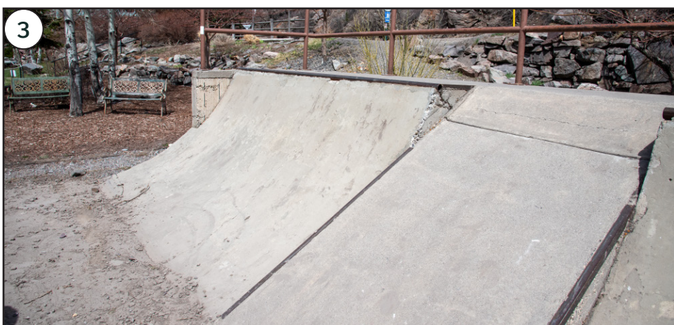
3 Skate Park Analysis: Deteriorating concrete needs improvement and or replacement.
