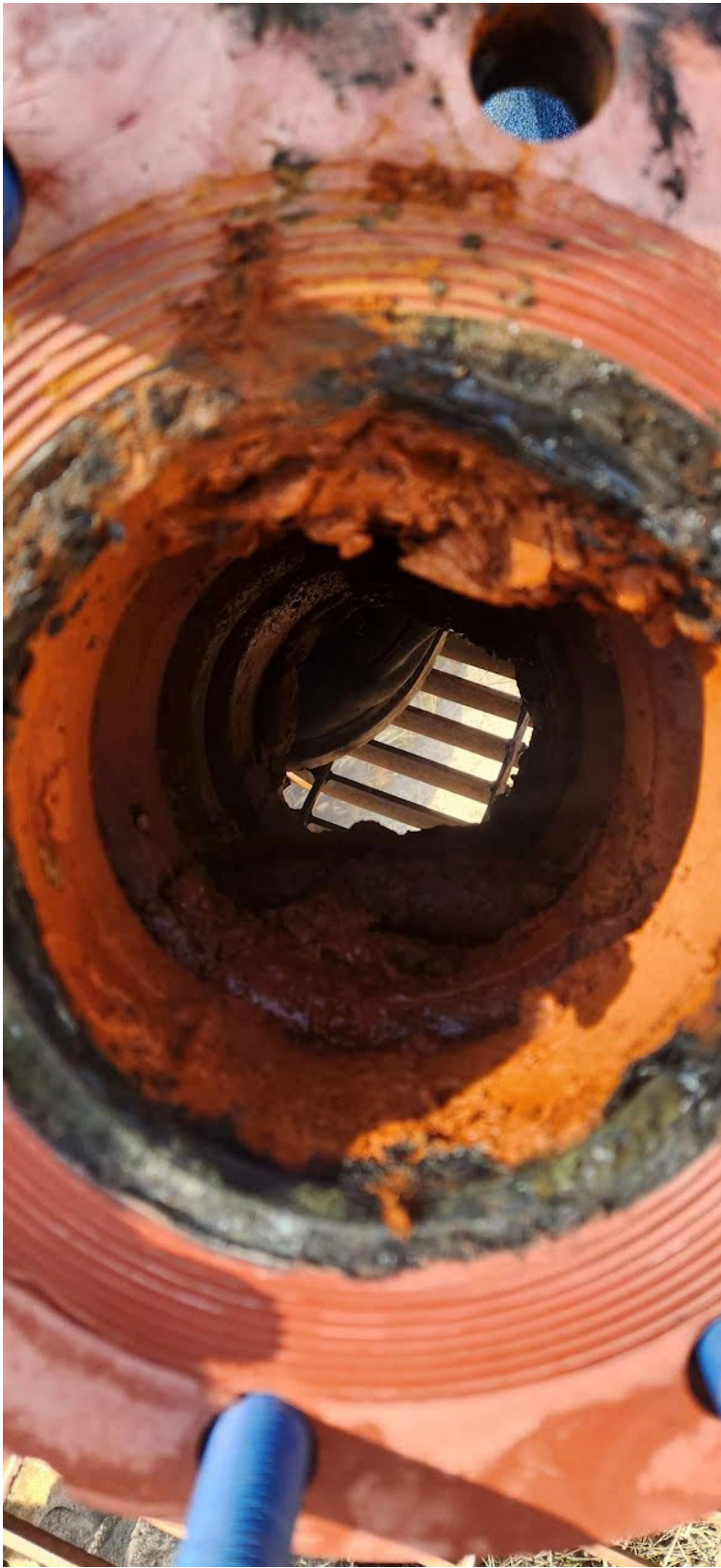
Mineral Buildup within Geothermal Pipe
