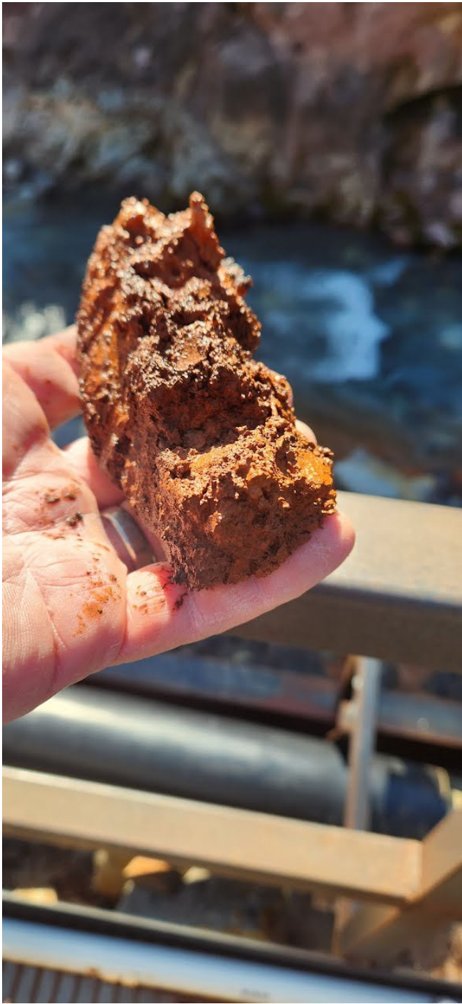
Mineral Buildup Removed from Geothermal Line
