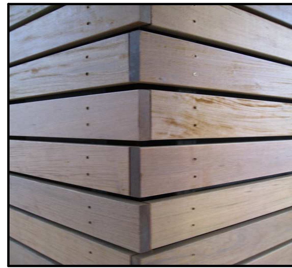
WOOD SIDING: THERMORY KODIAK SPRUCE 5/4x8 W/ EXPOSED FASTENERS OVER METAL AT REVEAL
