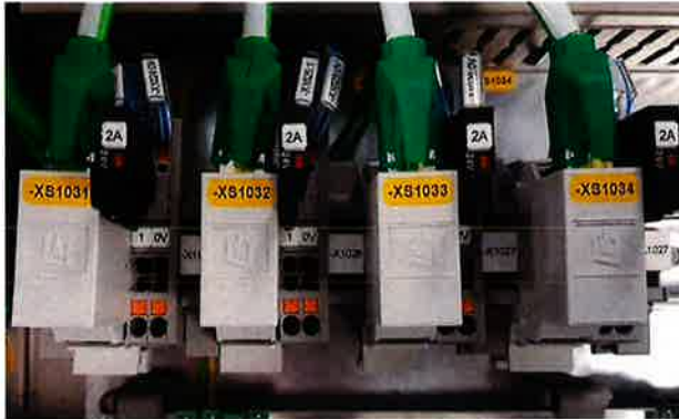
Figure 33 - READY Collector Base 24 VDC connection
