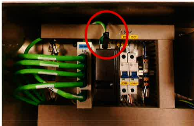
Figure 38 - LAN and power connection, SIERRA Wireless RV50x
