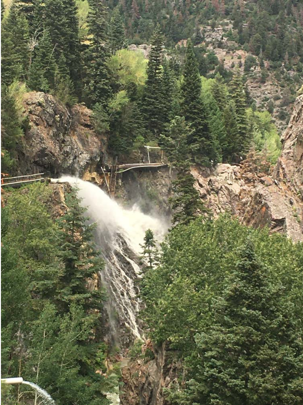
Photo: Penstock break. Witnesses said that the water from the initial break hit the bottom of the Sky Ladder.
