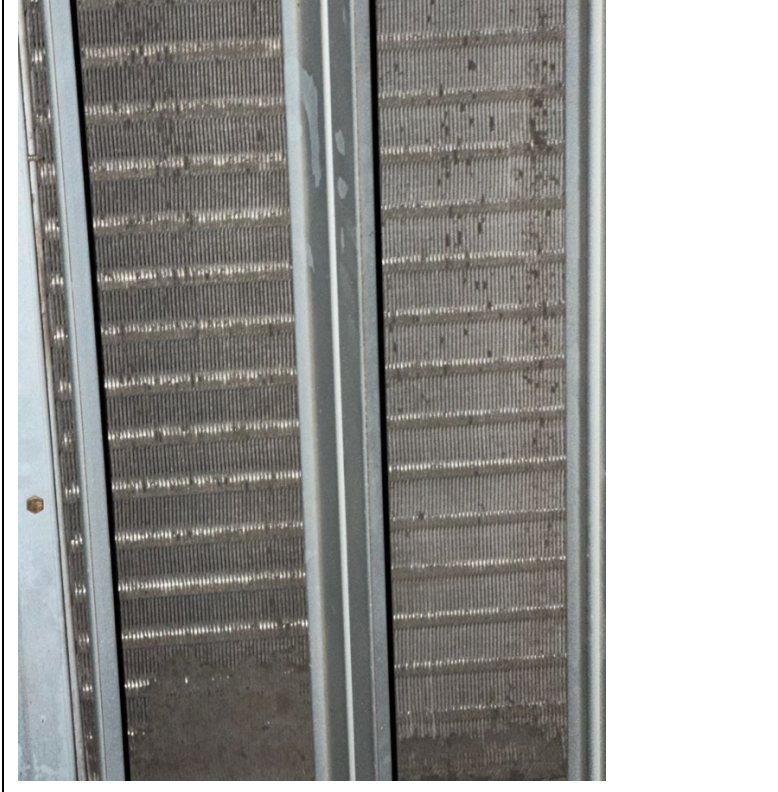
Dirty coil face inlet
