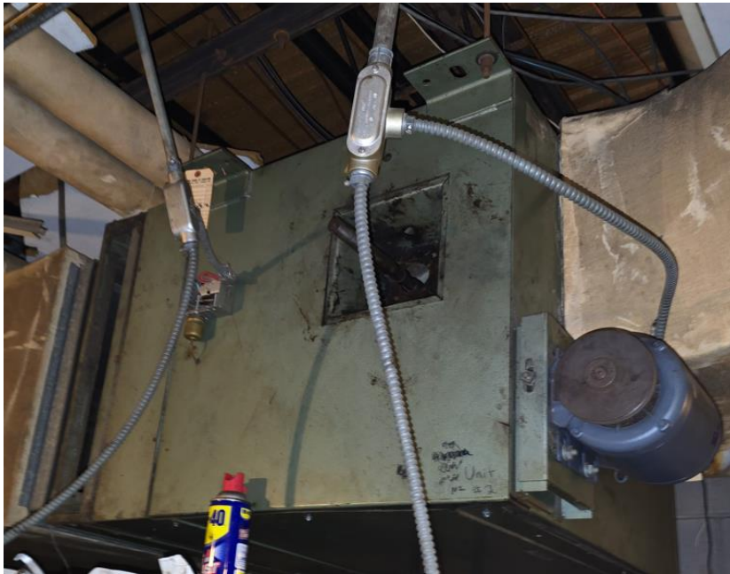
Figure 5. Non-classroom HV unit missing fan sheave
