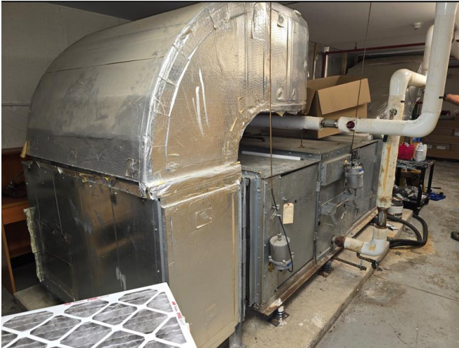
Figure 8. Classroom Addition HV unit
