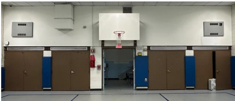
Figure 3. Gym cabinet heaters
