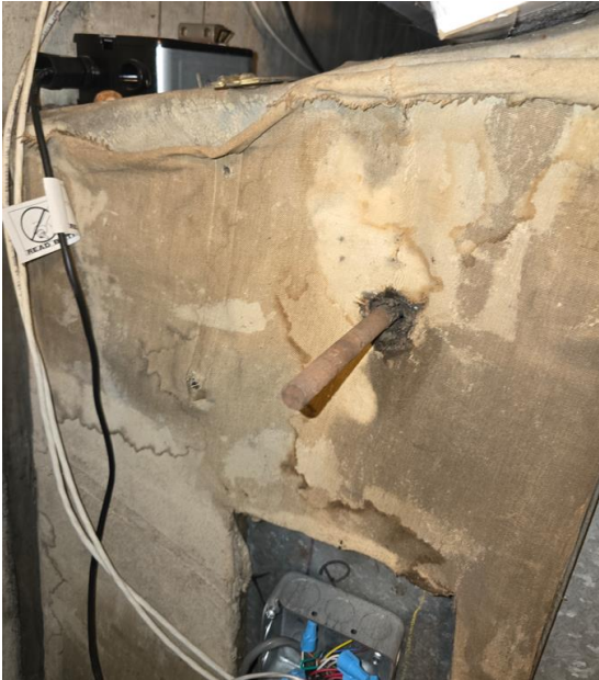
Figure 7. Damper shaft not connected
