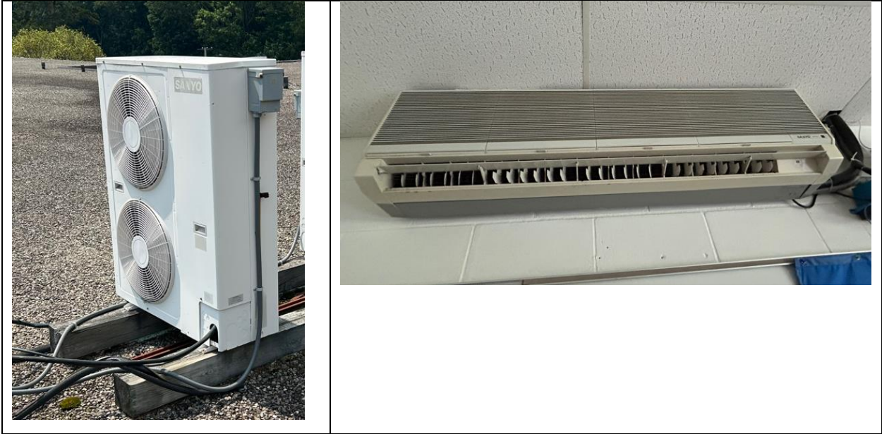
Figure 10. Ductless Split System
