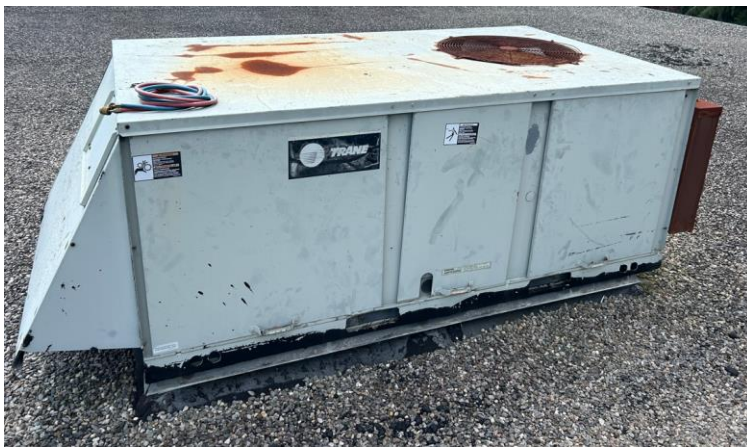
Figure 9. Roof Top Unit
