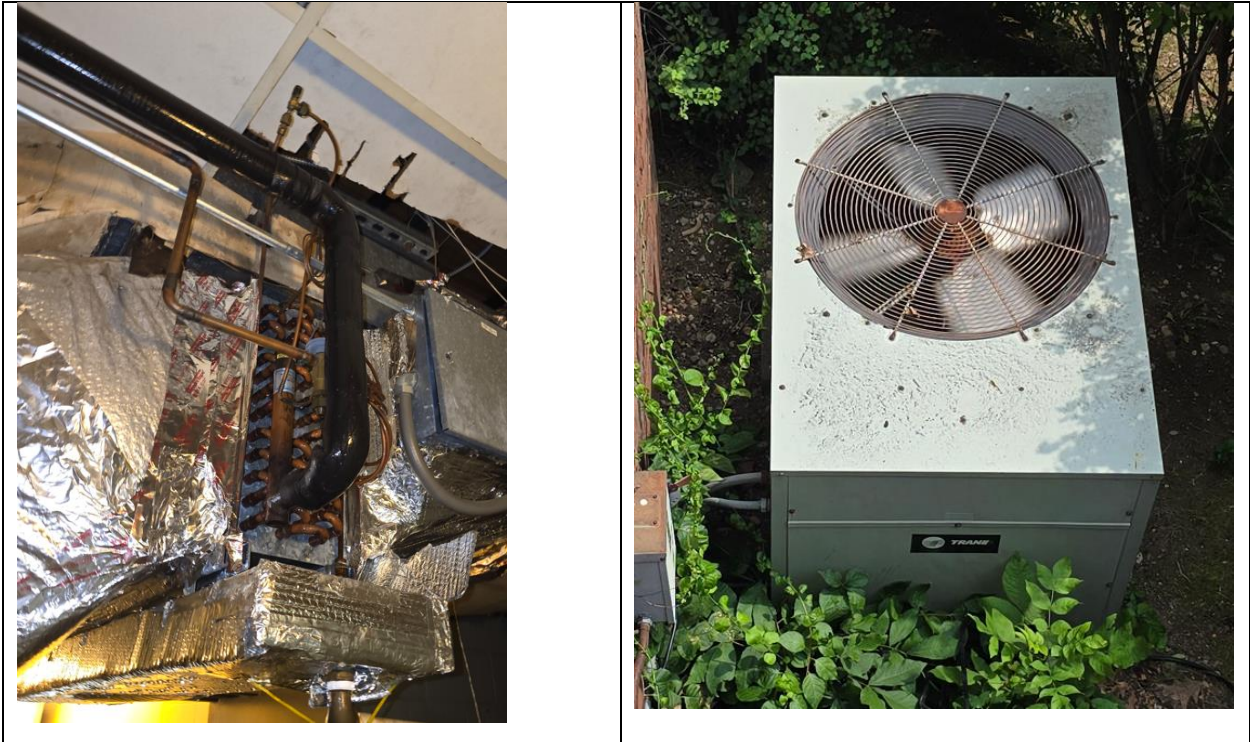
Figure 11. Gym A/C Coil and Condensing Unit
