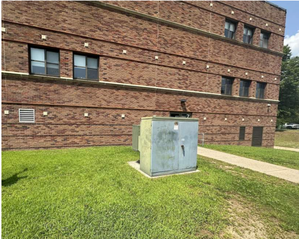
Exhibit 6: Photos of the existing utility transformer
