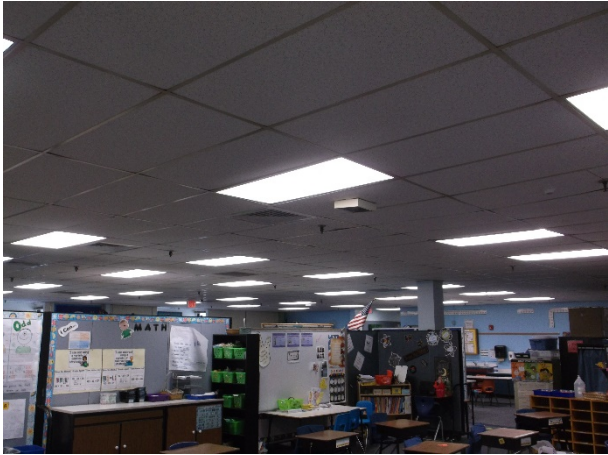
Existing 2x4 light fixtures
