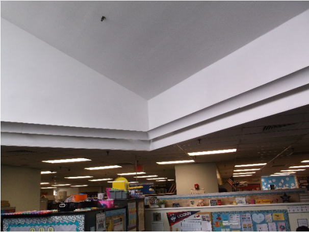
Existing "Curved" Valance light fixtures
