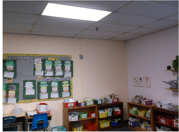
Surface mounted receptacle
