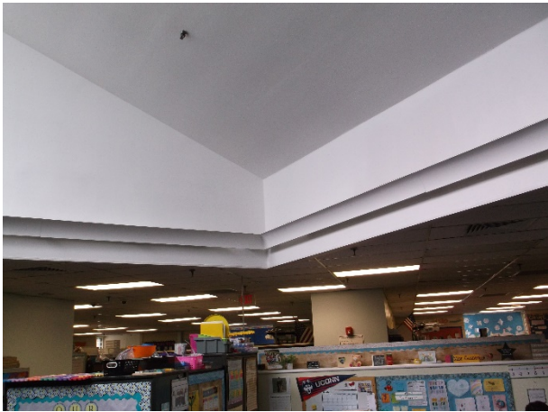
Existing "Curved" Valance light fixtures
