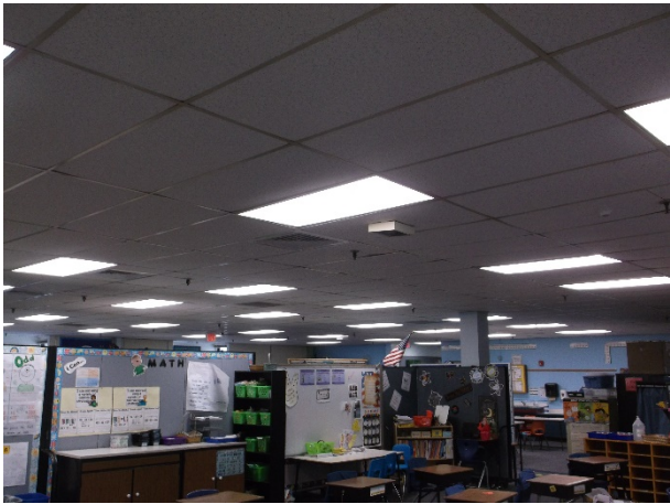
Existing 2x4 light fixtures
