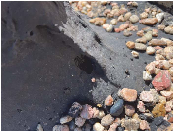
Hole around a Curb allowing water to enter the building
