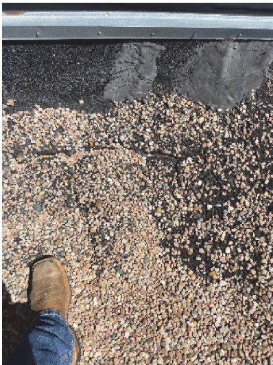
Roof System Failing
