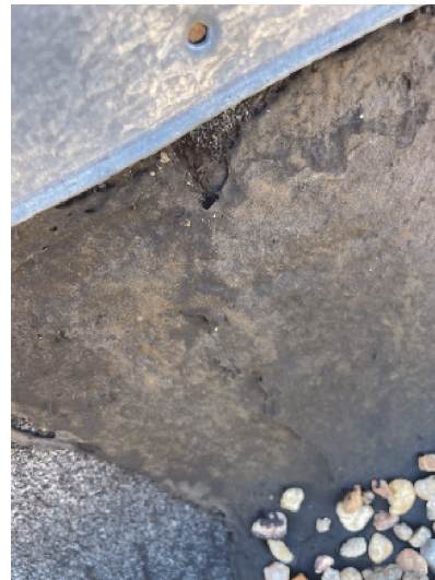
Hole around a Curb allowing water to enter the building
