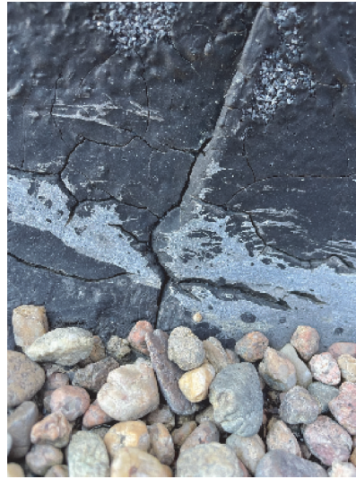
Built up tar starting to age and crack
