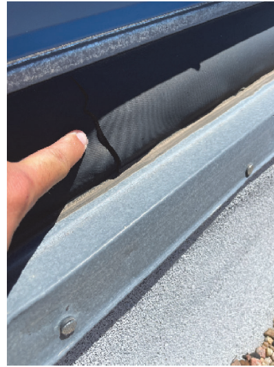
Expansion Joint Cracking
