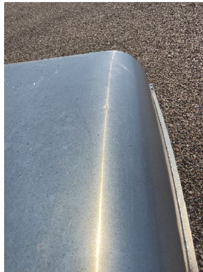
Hail damage to soft metal vent caps
