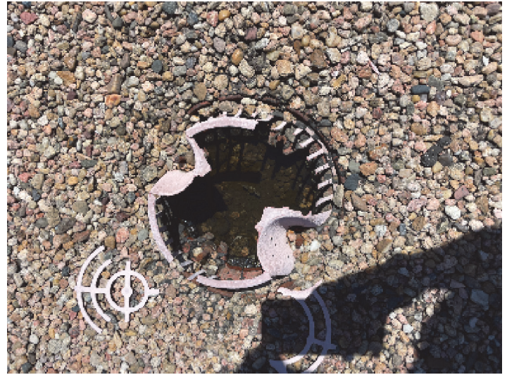
UV rays and hail damaged roof drain
