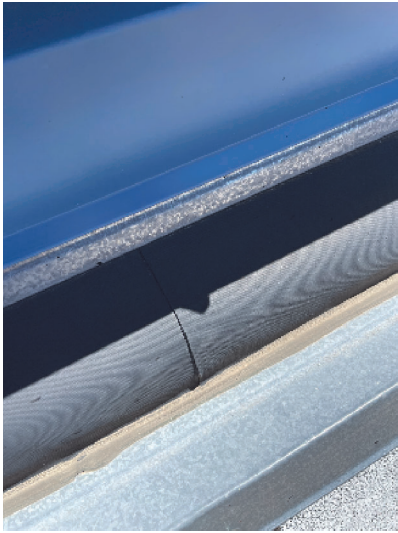
Expansion Joint Cracking
