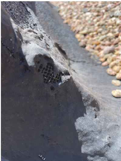
Failing sealant around a roof top curb
