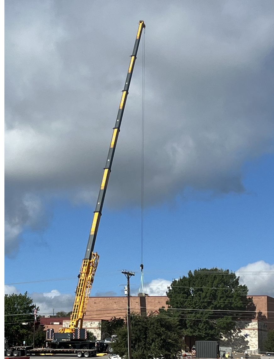
Photo: WHS Gym HVAC Units
