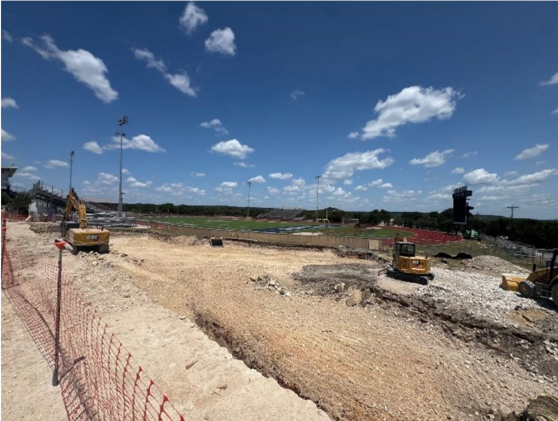
Photo: Underground Detention Pond
