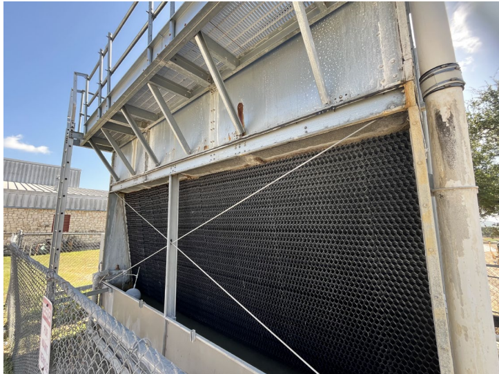
Photo: Cooling Tower Updated
