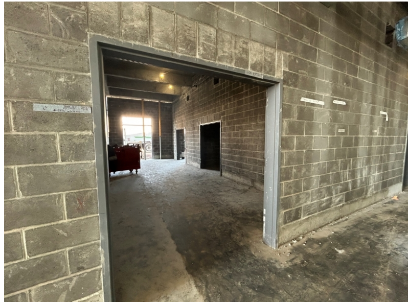
CMU walls complete on 1 st floor 1 st floor– Area A, B, C, D
