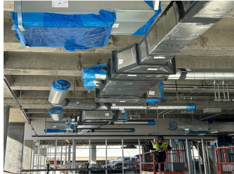
Overhead mechanical, electrical and plumbing 1 st floor
