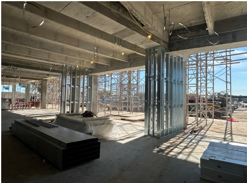
Cold form framing in progress 1 st floor– Area A, B, C, D
