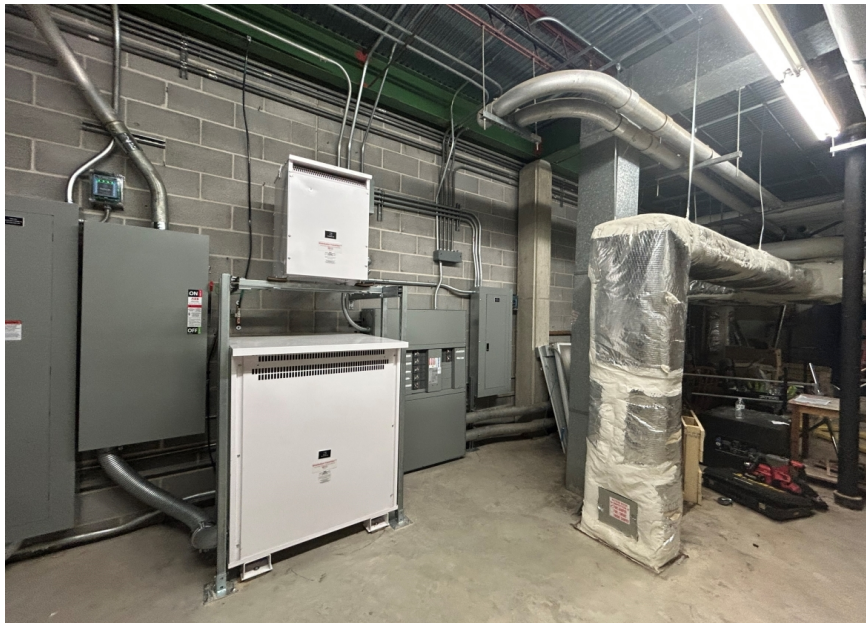
New transformers and panels
