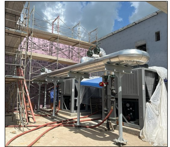
Chillers installed at the central plant
