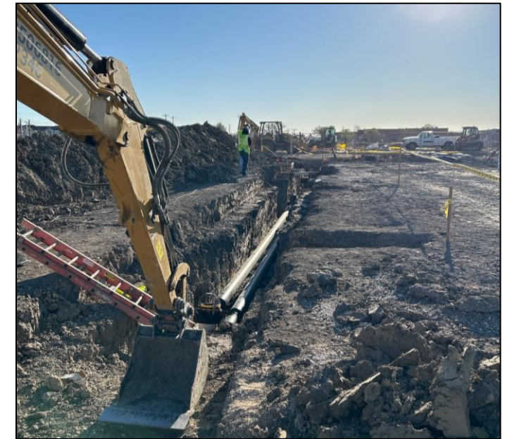
Underground hydronic piping
