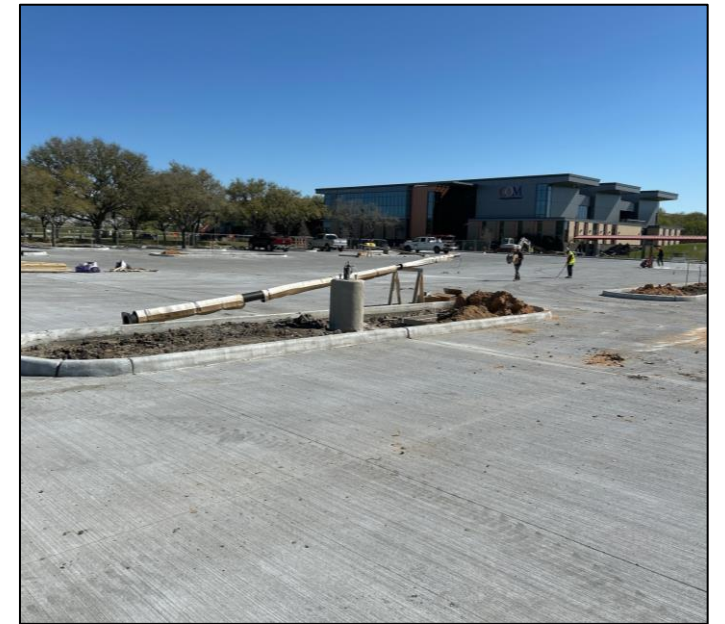
Lighting - Parking Lot B
