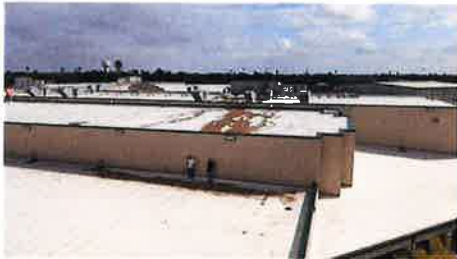
28. NOTE; After ARGIO cleaned roof membrane, the HVAC equipment was serviced & stained roof.
