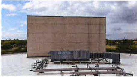
27. Performing Art's new metal allows stains from original roof to be exposed.
