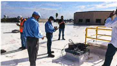
13. Typical, obsolete curbs need proper sized caps.
