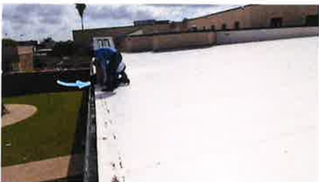
4. Typical, need metal end closures.
