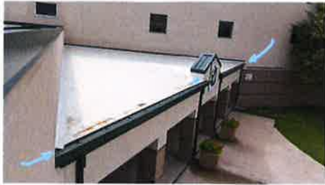
3. Typical, need metal end closures.
