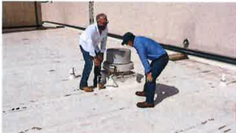
20. Typical, ensure electrical lines are as per code.
