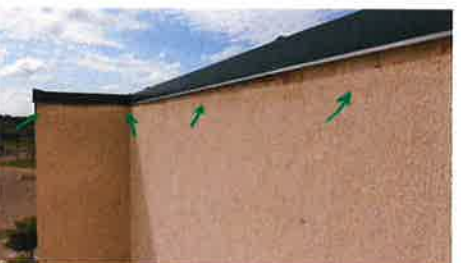
26. Typical, increased height of wood nailers on walls allowed stains from original roof to be exposed. Uncertain if Owner wants them removed.
