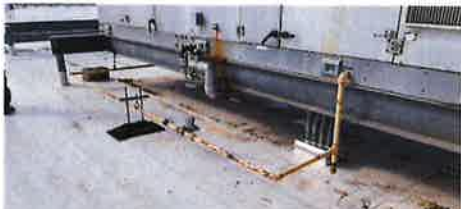
Typical: Supports required within 2' of ELLs or TEEs and 10' max. on straight lines. Normally, Yellow paint required on gas lines
