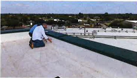
29. NOTE; Performing Arts has flashing that billows. Need to make an effort to re-adhere the flashing. Perhaps, the repairs might include additional securement with T-Bar to prevent it coming loose in the future.
