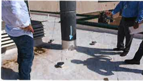
11. Typical, install termination clamps & sealant. If possible, improve guy wire attachments.
