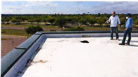
8. Typical, remove excessive wrinkles @ drains.
