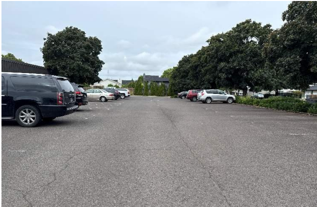
1. Parking areas need to be restriped.
