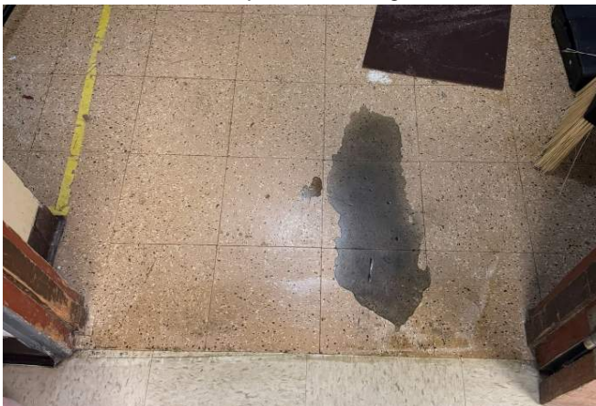
5. Heavy damage to presumed asbestos tile.
