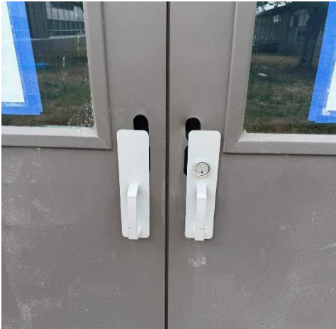
7. Hardware fix on doors, replacement of doors needed.
