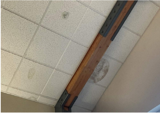
1. Roof leaks at main entry.
