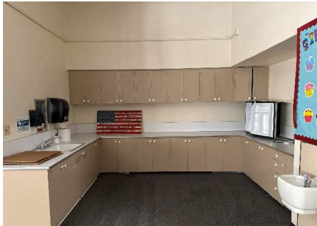
3. Typical original classroom casework and non-compliant drinking fountain.
