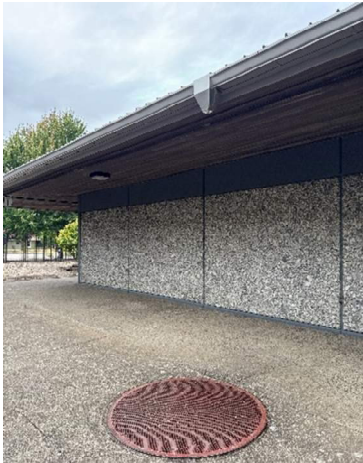
3. Storm drains splash on ground and make passing time very wet during inclement weather.
