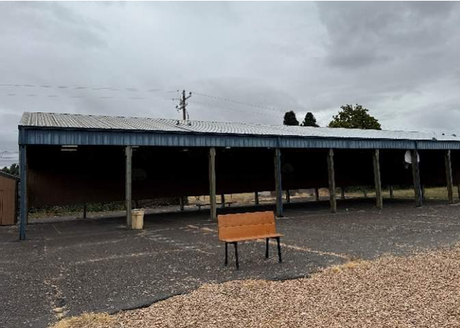
3. Asphalt paving at play areas showing significant cracks and wear.
