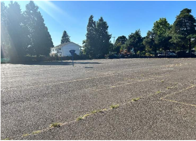
1. Significant cracks at asphalt play area, has drainage issues in winter.
