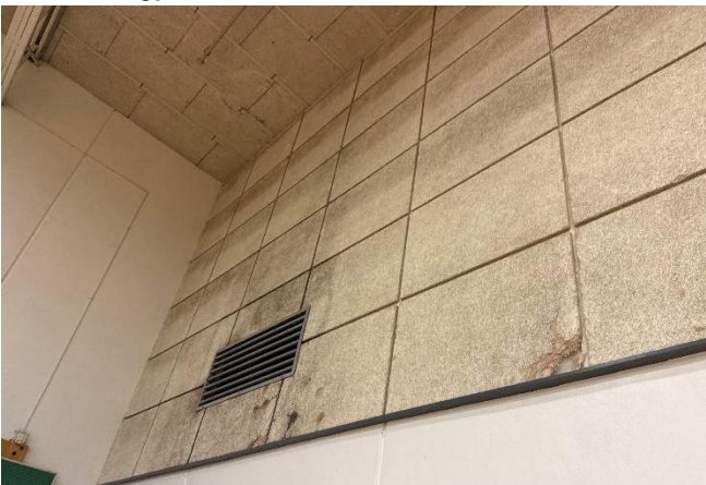
5. Damaged acoustic panels with dirt/dust accumulation in the main gym.
