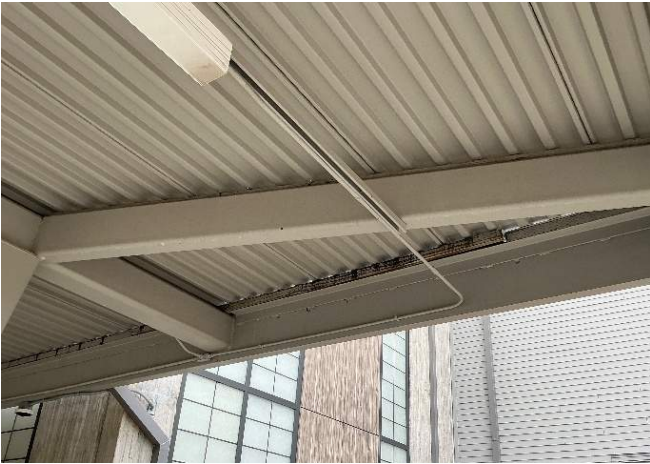
1. Entry canopy leaking at gaps in decking.
