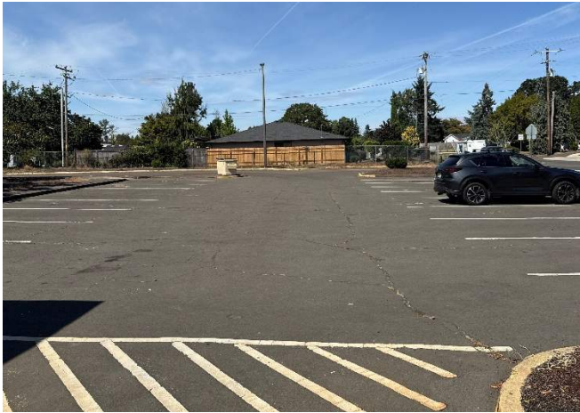
1. Asphalt cracking at north parking area.
