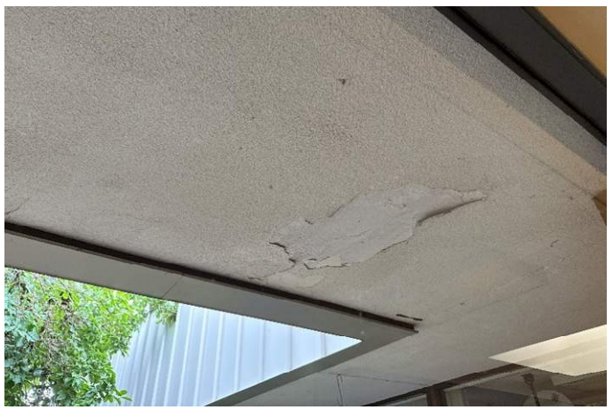
4. Paint finish at exterior soffit peeling.
