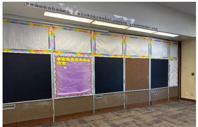
6. Operable partitions in classrooms causes sound issues.
