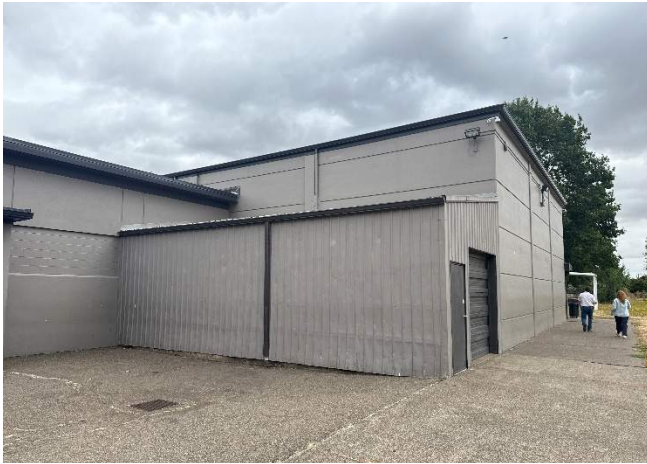
1. Equipment storage shed with pest and water intrusion issues.
