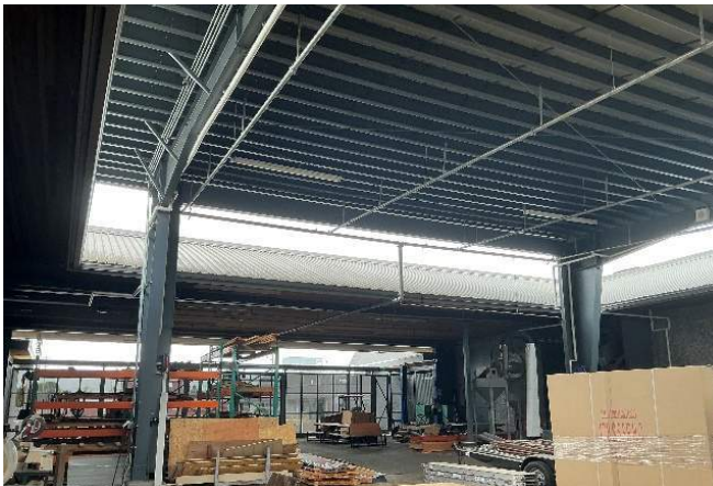
5. Corner of existing roof pours rain down into covered shop space. Need to address storm/gutter system.
