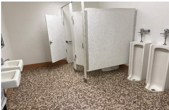
5. Dated student restroom, sinks, toilet stalls and urinals not ADA compliant.
