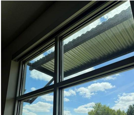
3. Gap at southern facing window screens may be causing glare issues.
