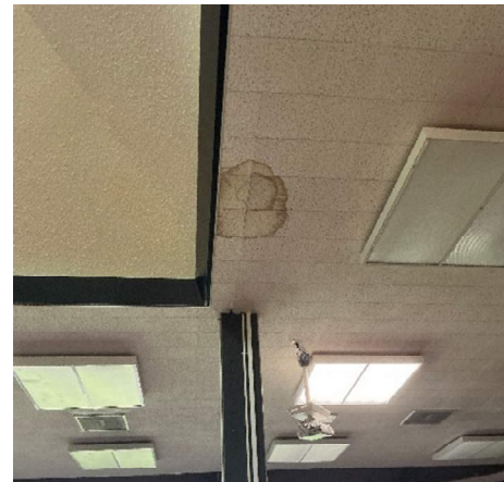
6. Ceiling and lighting in Library needs to be replaced.
