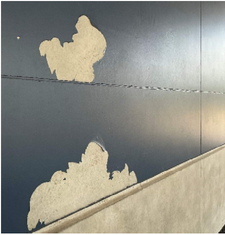
1. Peeling paint on the exterior tilt concrete walls.
