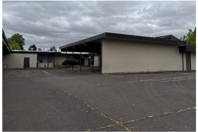
2. Significant cracks at asphalt play area, deteriorating siding at covered play.
