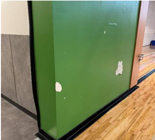
3. Paint failure at interior walls.
