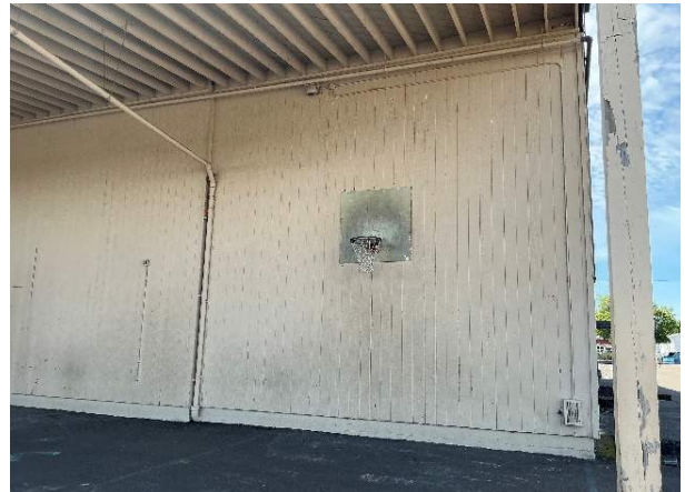
6. Equipment in need of replacement, siding and wood columns in need of repair.
