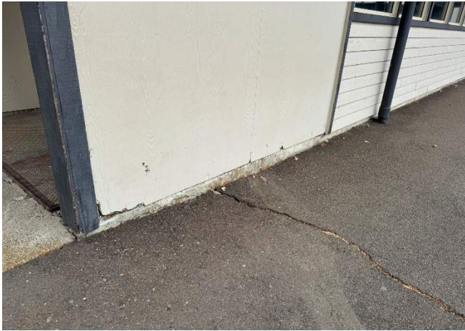
1. Significant deterioration of façade siding, cracking at play area asphalt.
