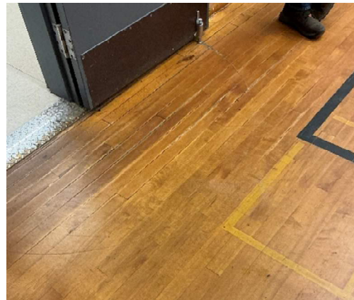
4. Gym flooring to get replaced or refinished.
