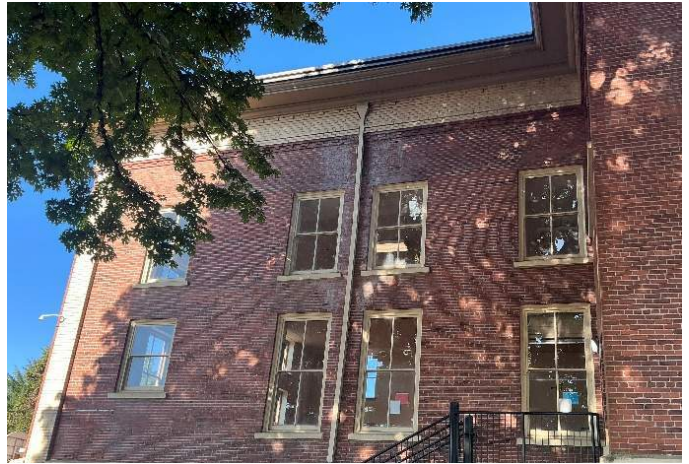
2. Water intrusion visible at brick adjacent to downspout.
