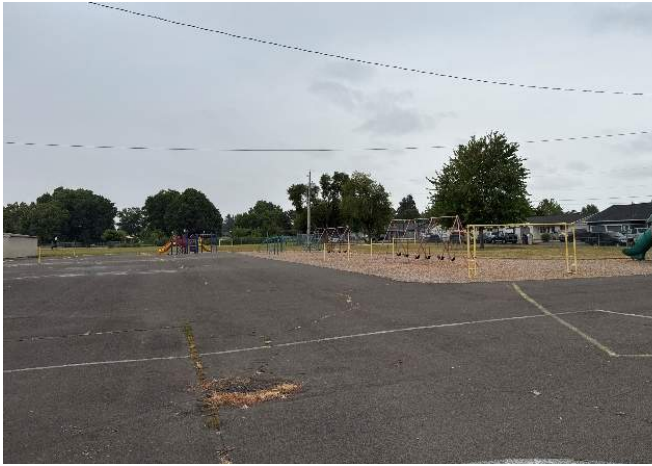
3. Visible cracks and damage to asphalt paving at play area.
