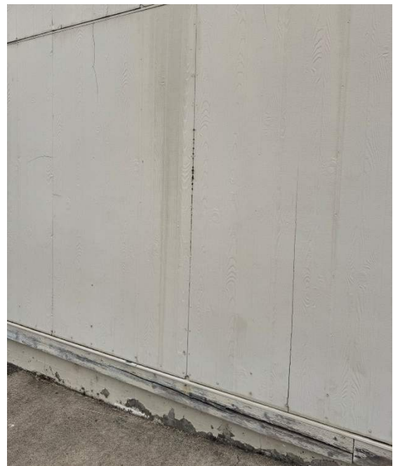
2. Visible water damage exterior siding.
