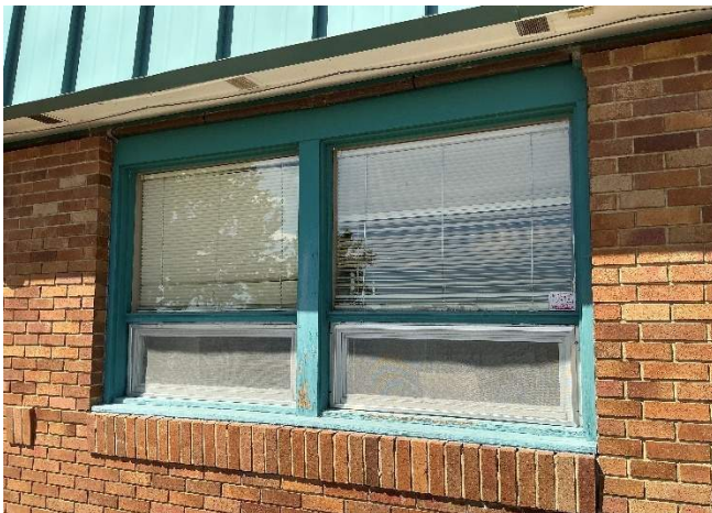
3. Original single pane windows and deterioration of wood trim.
