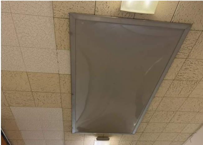
3. Skylights covered in recent roof repair, ceiling tiles need to be replaced throughout.
