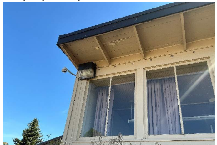
8. Damaged soffit and single pane windows.
