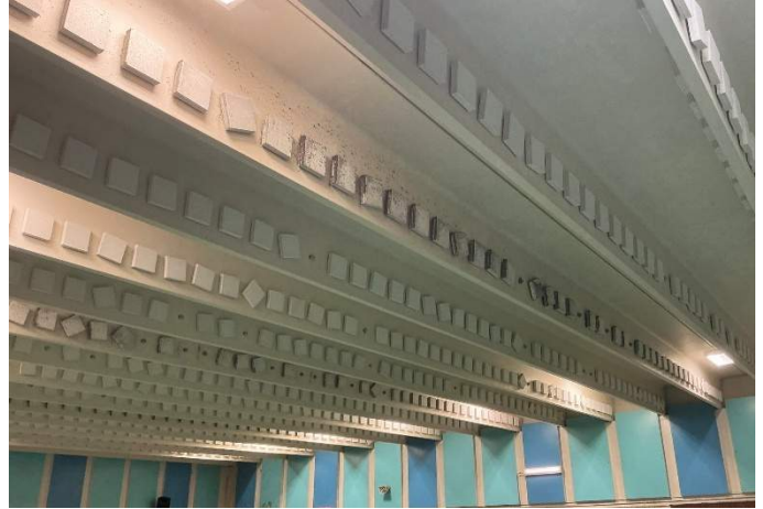
4. Dirt and dust accumulation on ceiling acoustic panels as well as many missing or crooked panels.
