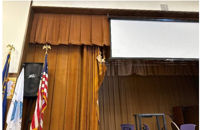
6. Stage curtain damaged, in need of replacement.
