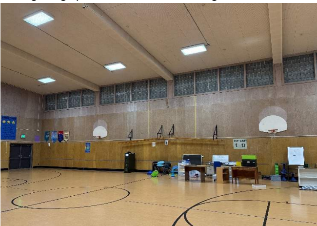
7. Aged wall panels and glass block in gym.
