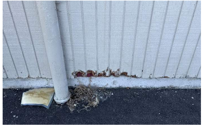
4. Siding damage at exterior.
