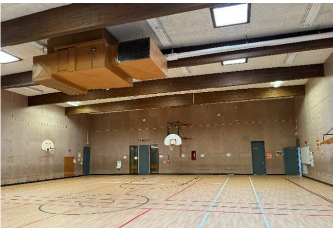
5. Large and noisy ventilation unit in gym.
