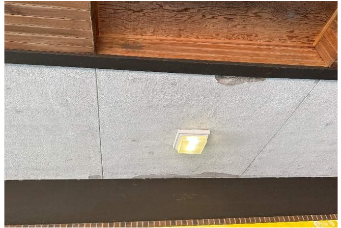
2. Exterior soffit finish spalling at main entry.
