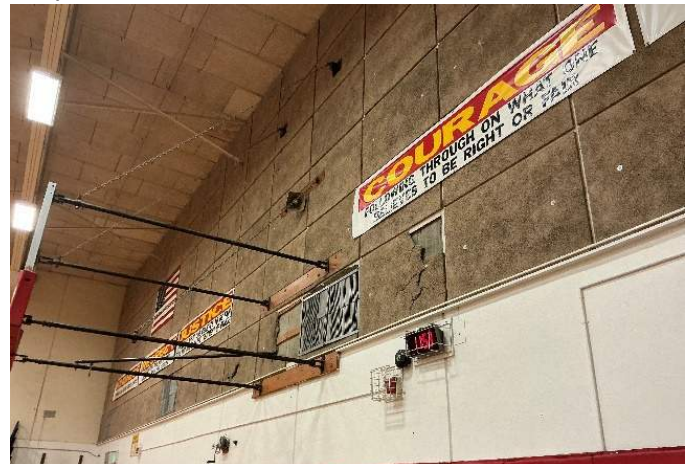
4. Acoustic wall panels at gyms to be replaced.
