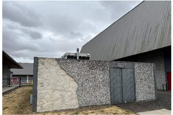
2. Wall at chiller with finish coming off.
