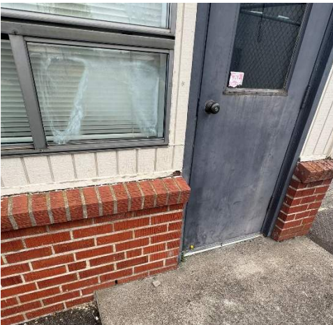
5. Failing window, heavy damage to exterior door and deteriorated siding and trim.
