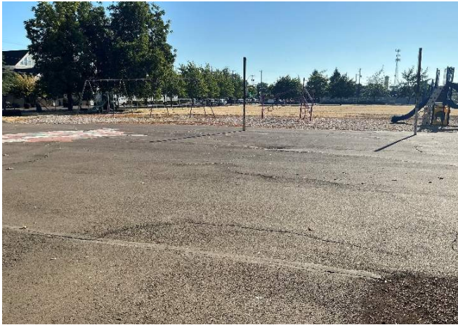
1. Uneven and cracked asphalt surface at playground.
