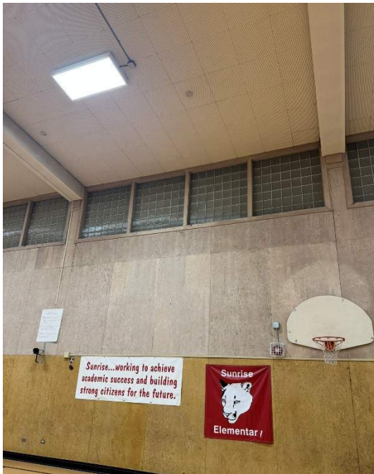
1. Aged wall panels and equipment in main gym.
