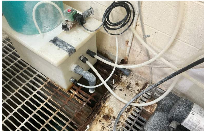
6. Long term corrosion on metal grating in equipment room.
