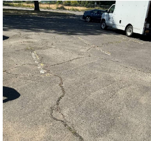
8. Site paving and striping to be redone.
