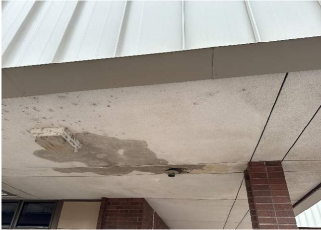
1. Significant water damage to exterior soffit panels.
