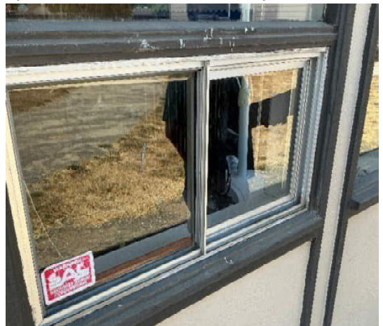
4. Single pane wood framed windows, showing heavy damage to frame trim.
