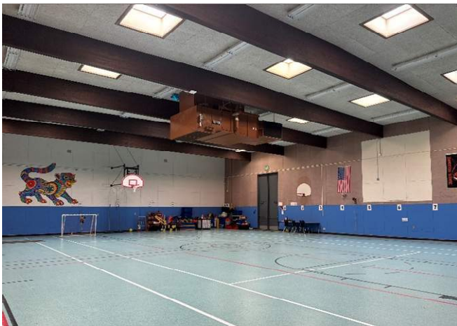
3. Low hanging and loud H&V unit in gym.
