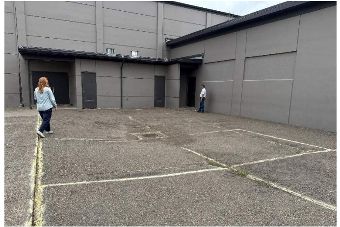
2. Significant cracks around the area drains at the exterior of the gyms.
