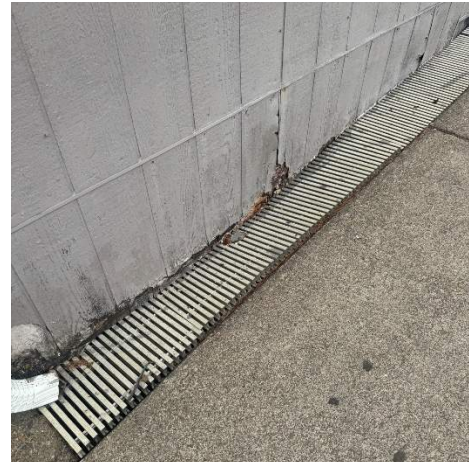
4. Deterioration of the siding at the modular.
