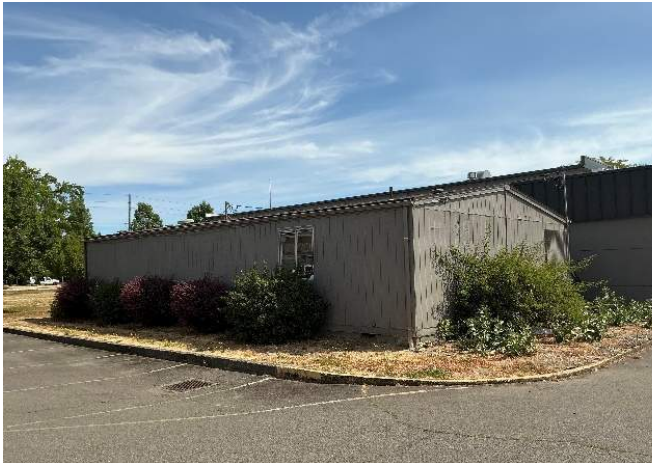
1. Unusable Modular to be removed.
