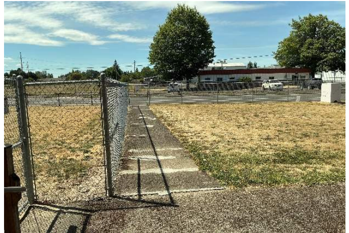
4. Site sidewalks showing damage and failing repairs.
