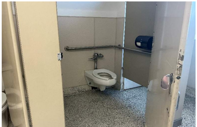
6. Un-updated group restroom, non-compliant stall.
