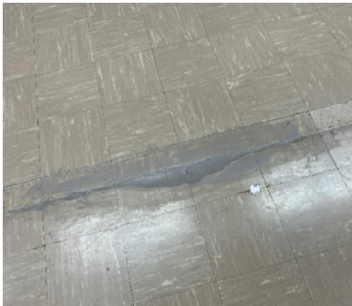
5. Suspected ACM tile in cafeteria, showing damage and temporary repair.
