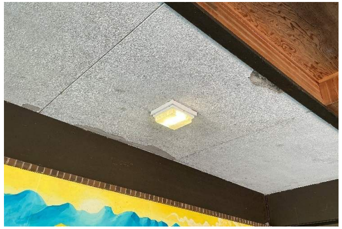
2. Spalling of the exterior soffit panel finish.
