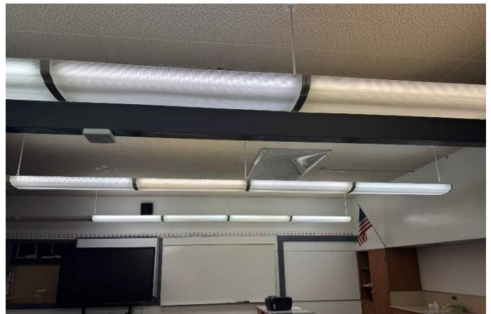
6. Fluorescent and inconsistent lighting in classroom.
