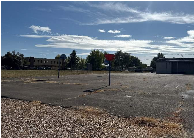
1. Poor asphalt conditions at play area.
