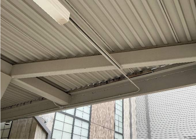
1. Entry canopy leaking at gaps in decking.
