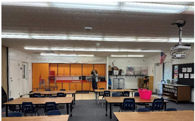
6. Fluorescent lighting in typical classroom.
