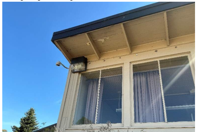
8. Damaged soffit and single pane windows.
