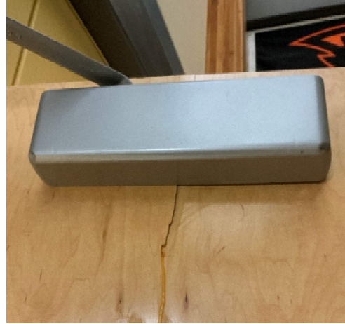
2. Significant damage to doors at gym.
