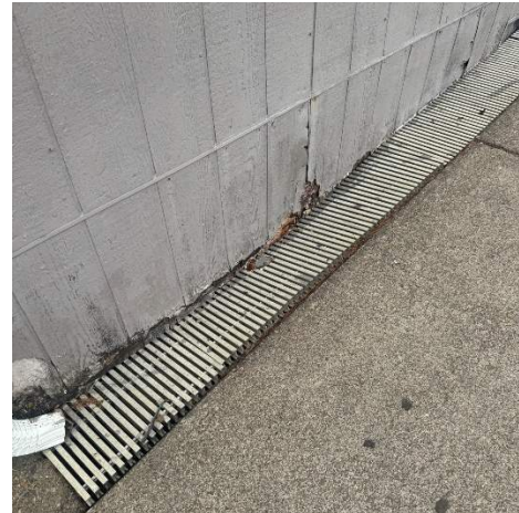
4. Deterioration of the siding at the modular.
