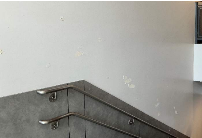
5. Paint failure at interior walls.
