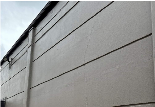
3. Visible repaired cracks in the tilt concrete walls of the gyms.
