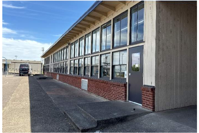
2. Single pane windows on the north facade and inaccessible classroom exits.
