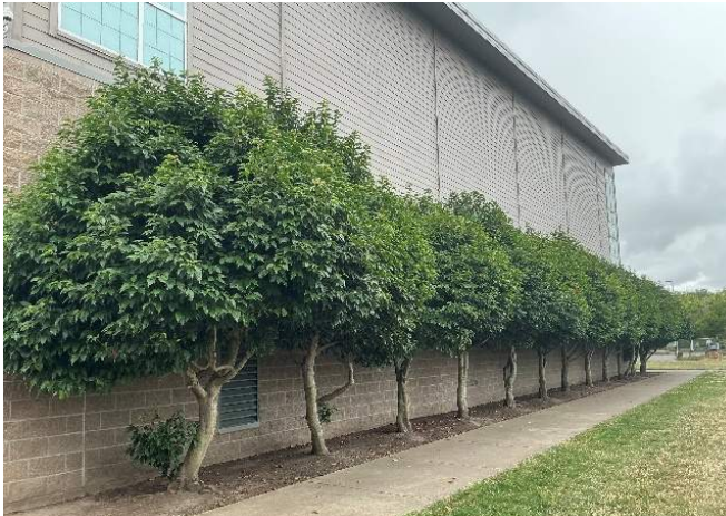
3. Trees planted too close to building.
