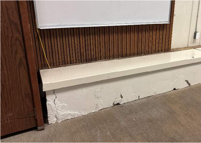
3. Visible water damage to wood paneling and damage to concrete bench.
