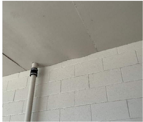
2. Visible water damage to exterior soffit boards, suspected un-reinforced masonry walls.
