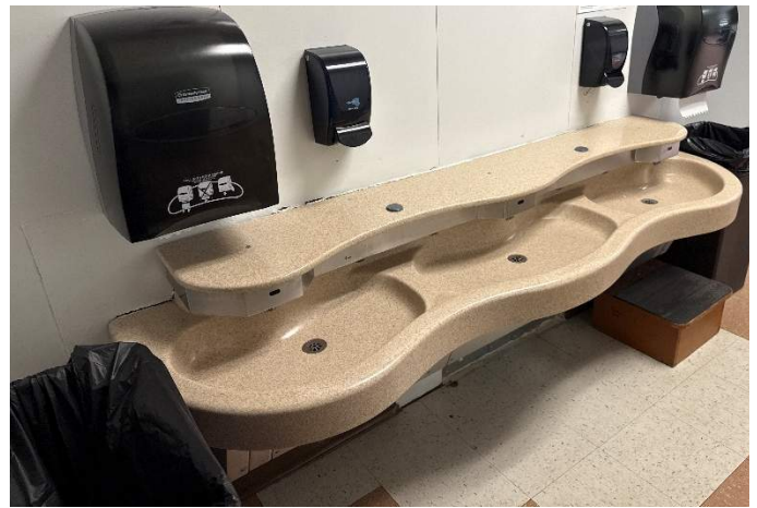
4. Sink pulling away from wall at restroom.
