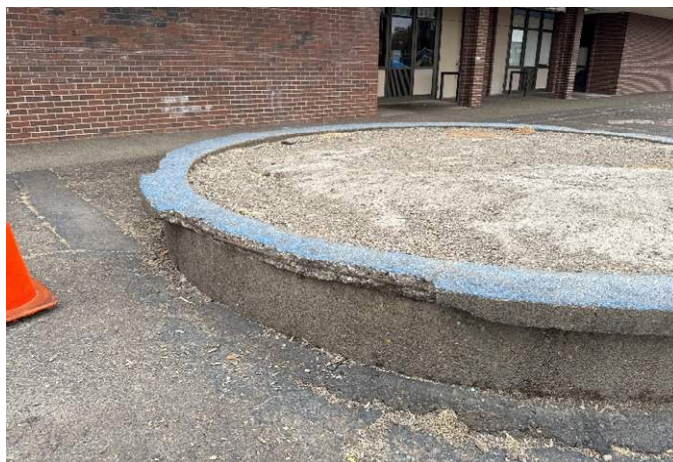
2. Exposed rebar and damaged concrete at former tree planters in the play area.
