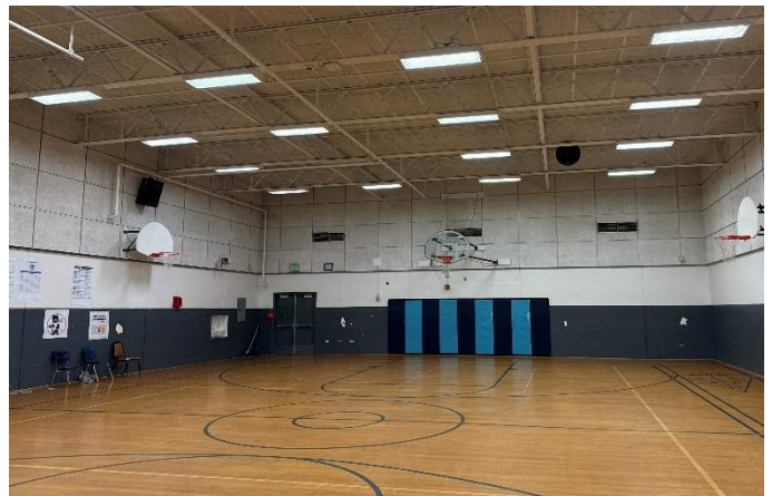
6. Damage to the wall pads and paint in the Aux Gym.
