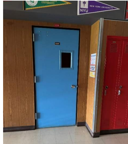
8. Typical classroom doors do not meet code for ADA Accessibility with hardware and clearances.
