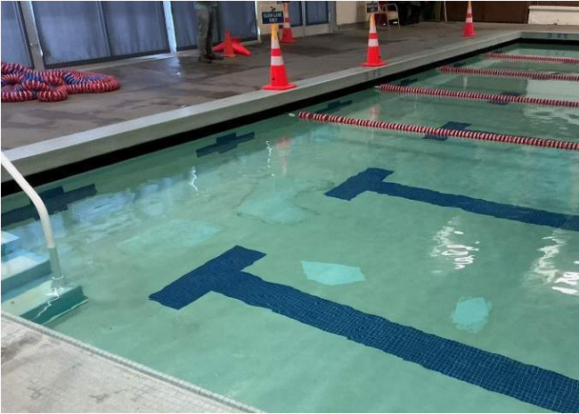
1. Multiple patches visible in the pool surface.
