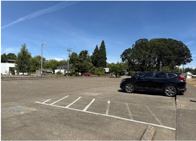
1. Parking area needs to be restriped.
