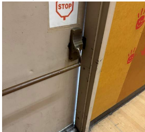
8. Visible gap in exterior door at Aux Gym.
