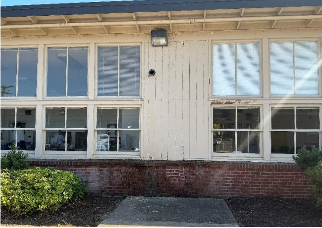
3. Significant deterioration of the siding, brick and trim at the exterior.
