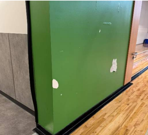
3. Paint failure at interior walls.
