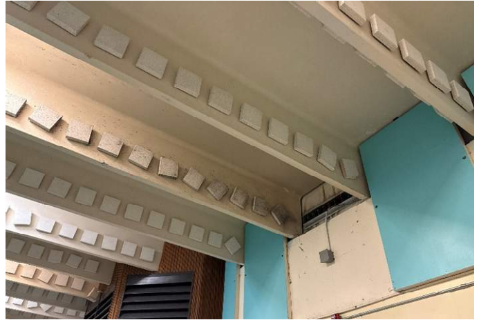
2. Dirt and dust accumulation on ceiling acoustic panels.
