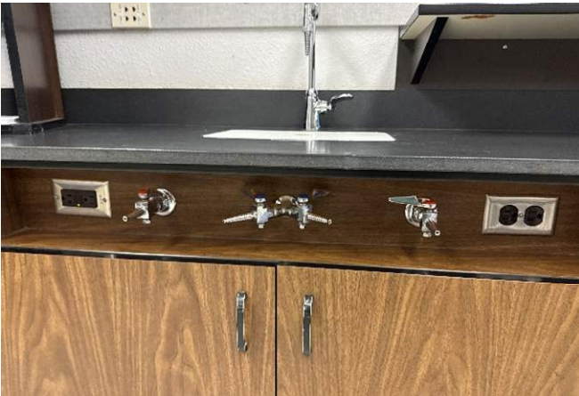
9. Science classroom equipment is outdated and needs to be replaced.
