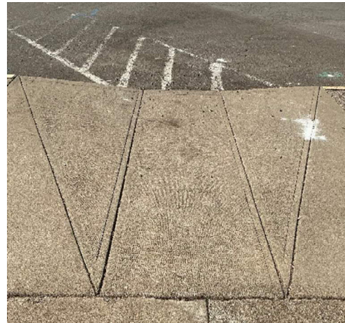
10. Curb cuts need to be modified to meet proper cross slopes
