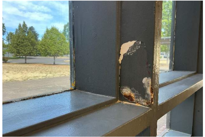
2. Storefront condition rusting through and single pane windows.
