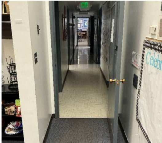
3. Hallway in main building, non-compliant clearance width in hallway and at door.
