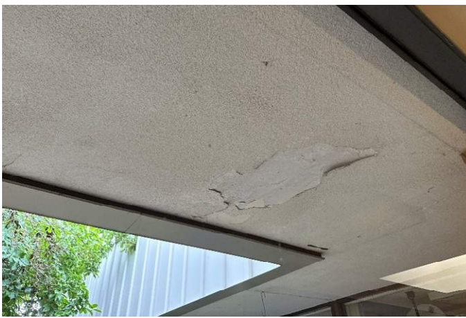
4. Paint finish at exterior soffit peeling.
