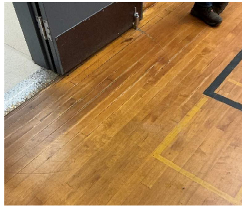
4. Gym flooring to get replaced or refinished.
