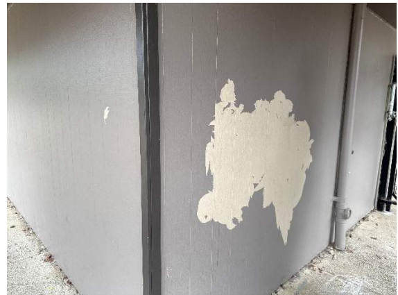
4. New exterior paint peeling at façade.
