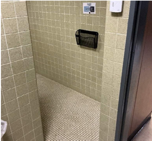
3. Non-compliant restroom clearances.
