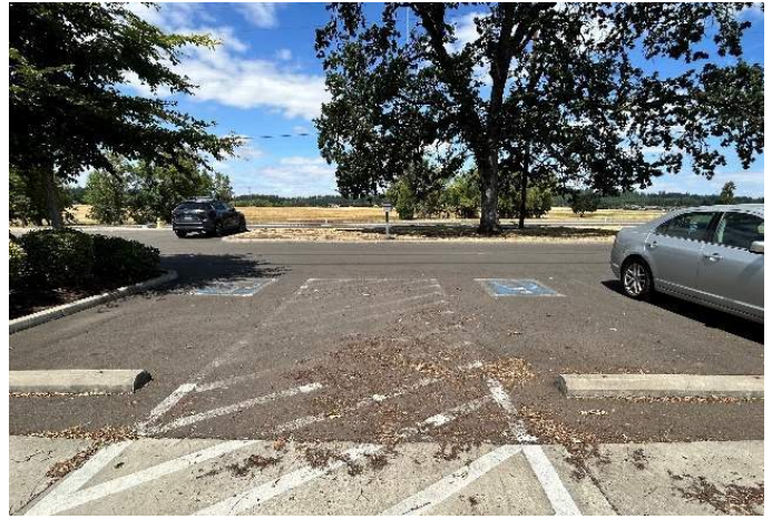
2. Heavily faded markings at accessible parking stalls.
