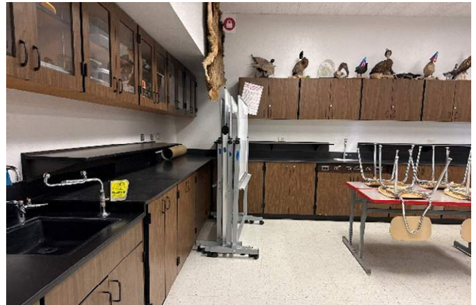
10. Science classroom casework does not have ADA Accessible stations. Classroom is too small for current enrollment.
