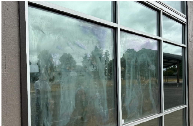
3. Storefront glazing failure at the Cafeteria exterior.
