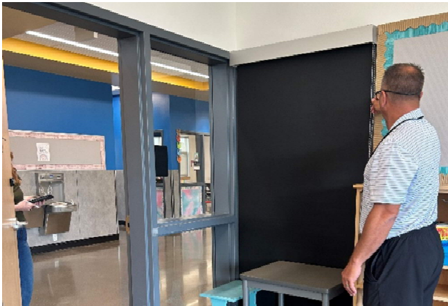
5. No window shades on interior windows to classrooms.
