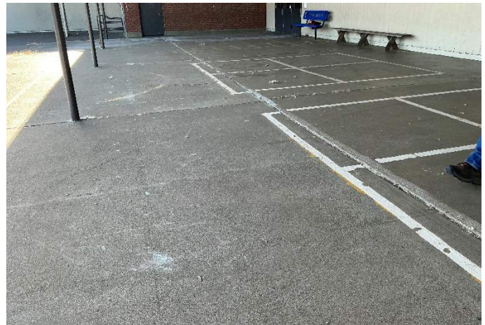
2. Significant cracks and gaps at concrete play area and at building exits.
