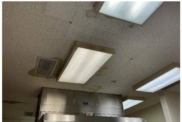
4. Heavy staining on ceiling tiles in the kitchen, fluorescent light fixtures.
