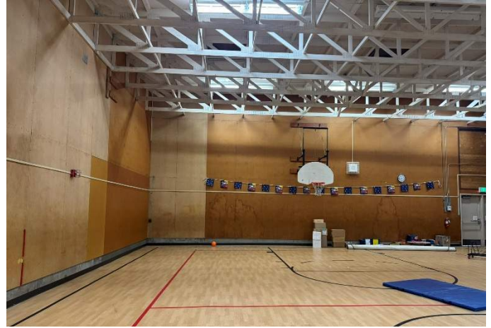
4. Visible water damage on patchwork wall panels in Aux Gym.
