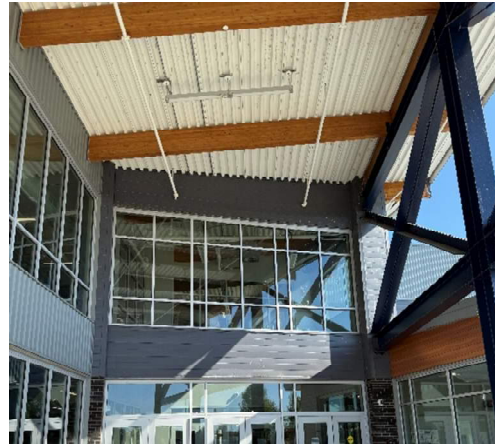
10. New entry. Birds perch on sprinkler lines and land create messes at main entry.
