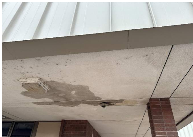
1. Significant water damage to exterior soffit panels.
