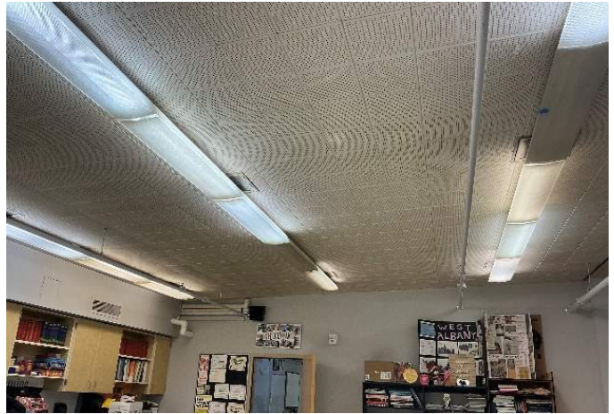
2. Original lighting in various stages of function.
