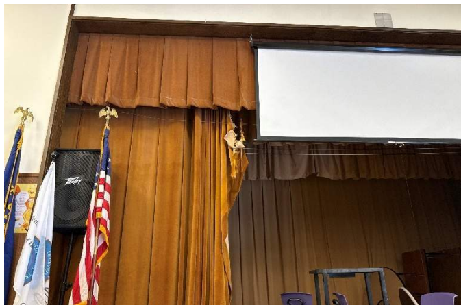
6. Stage curtain damaged, in need of replacement.
