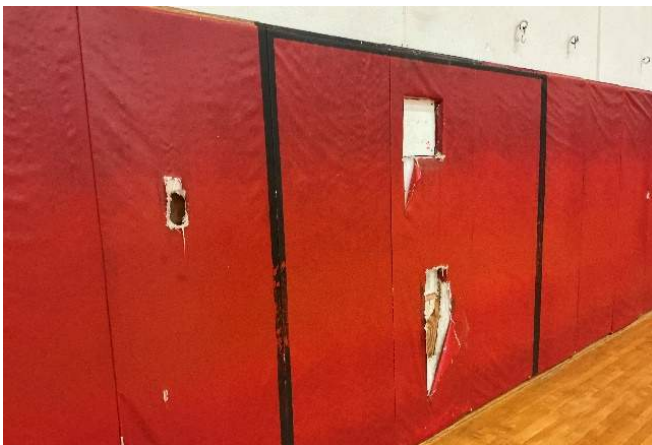
5. Wall mats at gyms to be replaced.
