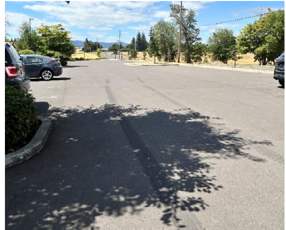
4. Parking areas in need of re-striping.
