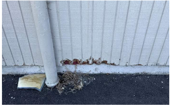
4. Siding damage at exterior.
