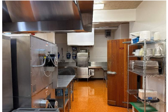
4. Aged kitchen equipment in an undersized space.
