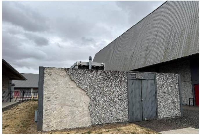
2. Wall at chiller with finish coming off.
