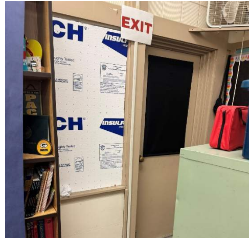
6. Exterior exit in classroom, missing illuminated signage, temporary insulation visible to help regulate temperature in room.
