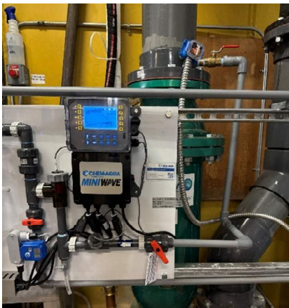
11. Water softener does not work.
