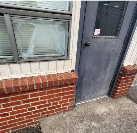
5. Failing window, heavy damage to exterior door and deteriorated siding and trim.
