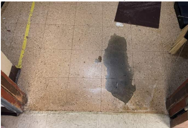
5. Heavy damage to presumed asbestos tile.
