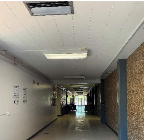
9. Lights in hallway old fluorescent fixtures.
