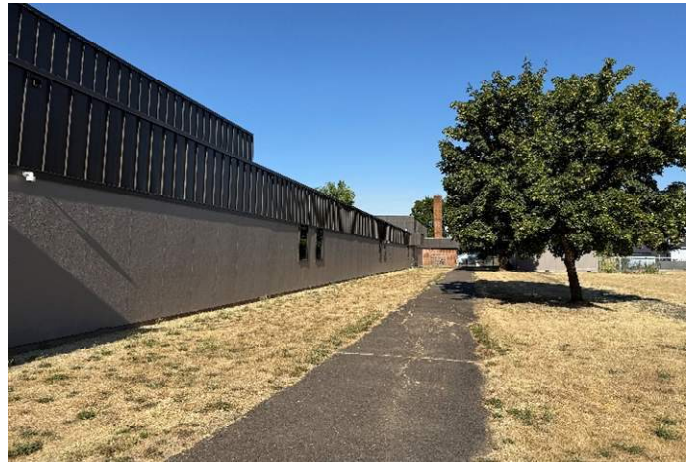
2. Degrading asphalt in site path, decommissioned chimney in background.
