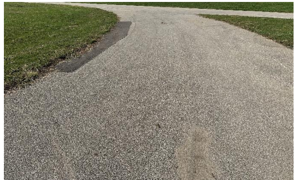
Photo 2: Surface Deformation – North Curve
