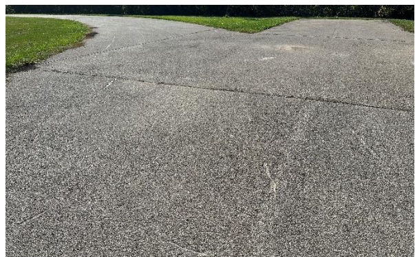
Photo 3: Longitudinal and Transverse Cracking
