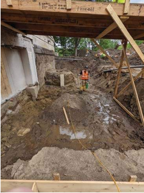
Wet Conditions Area Observed
