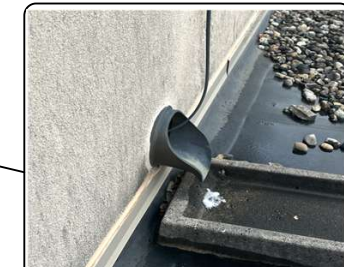
Section G. "Roofing Contractor" to raise existing through-wall downspout nozzle to meet manufacturer's minimum flashing height requirements.
