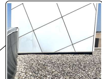
Cut and raise bottom of existing metal wall panels on Section F for new 8" flashing height.
