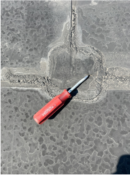
Repair cracked T-Lap flashing.
