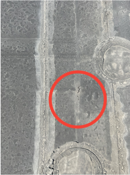
Repair cracked T-Lap flashing.
