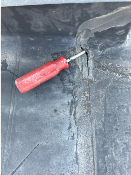
(63) Repair open soil stack flashing.
