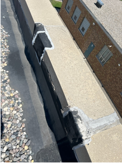
Severely damaged 8"x 4' limestone capstone.
