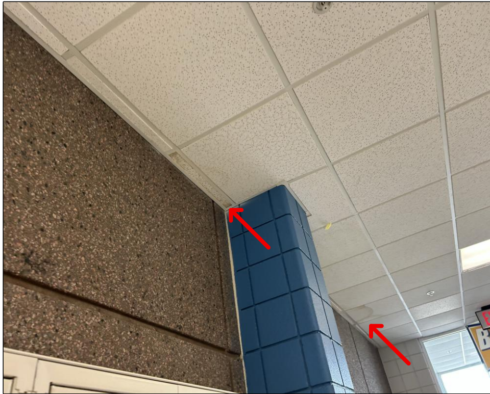
Multiple leak areas where vertical sealant joints are failing.
