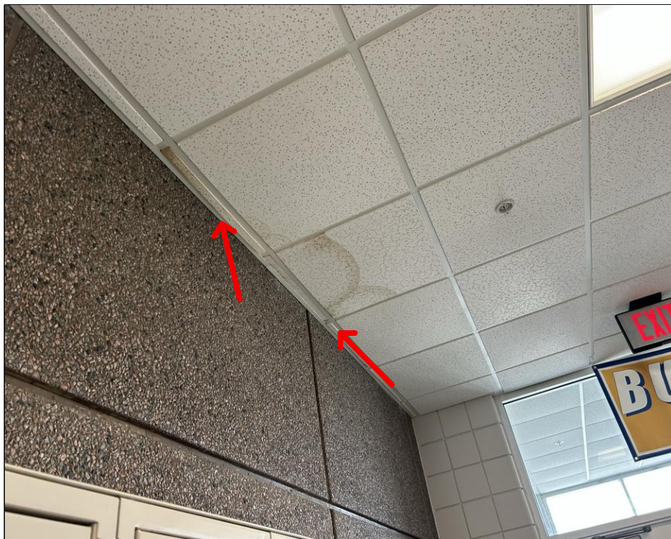
Leak areas where additional vertical sealant joints are failing.
