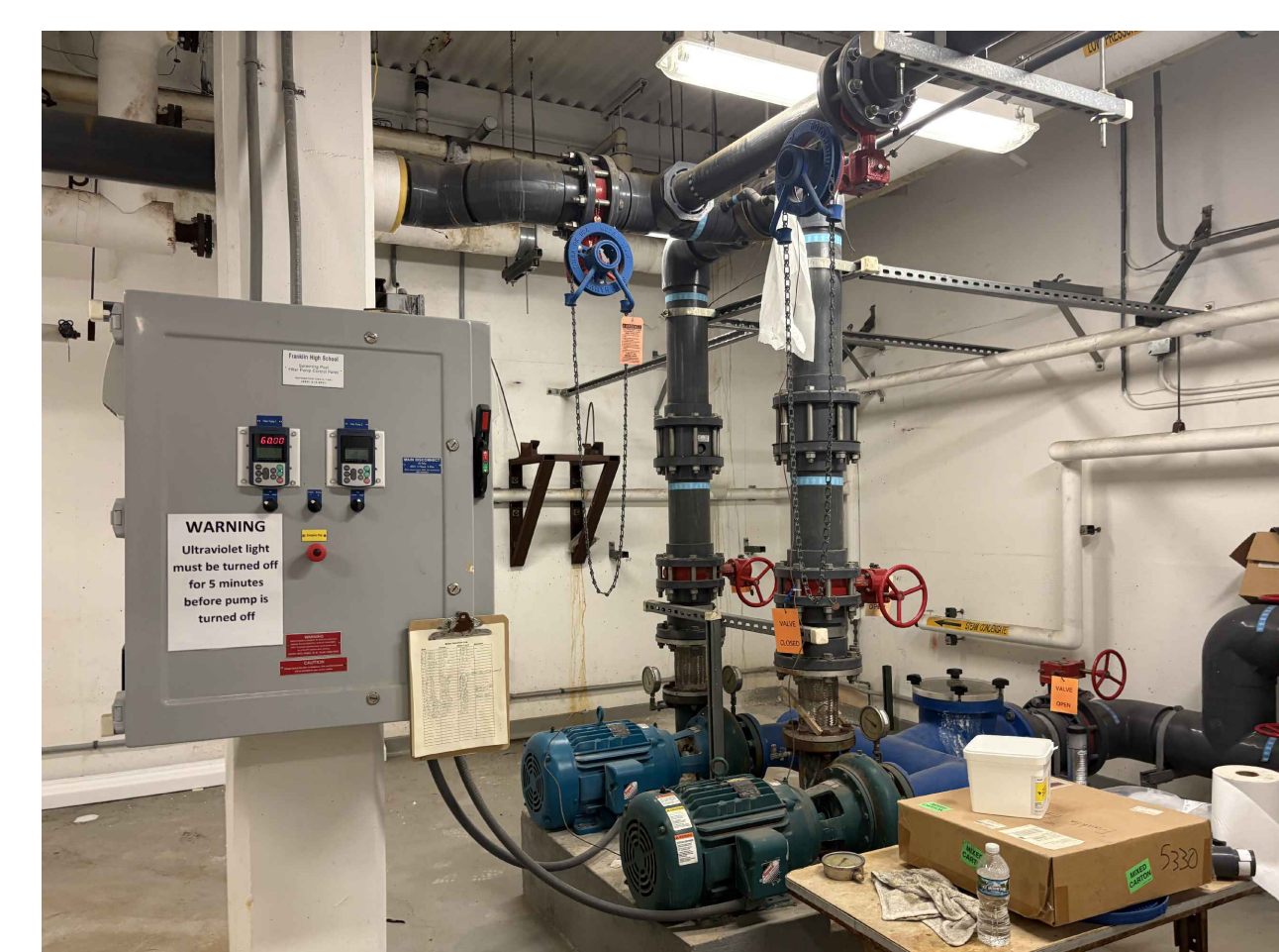
1 EXISTING RECIRCULATION PUMPS & STRAINER AQ0.2 NTS
