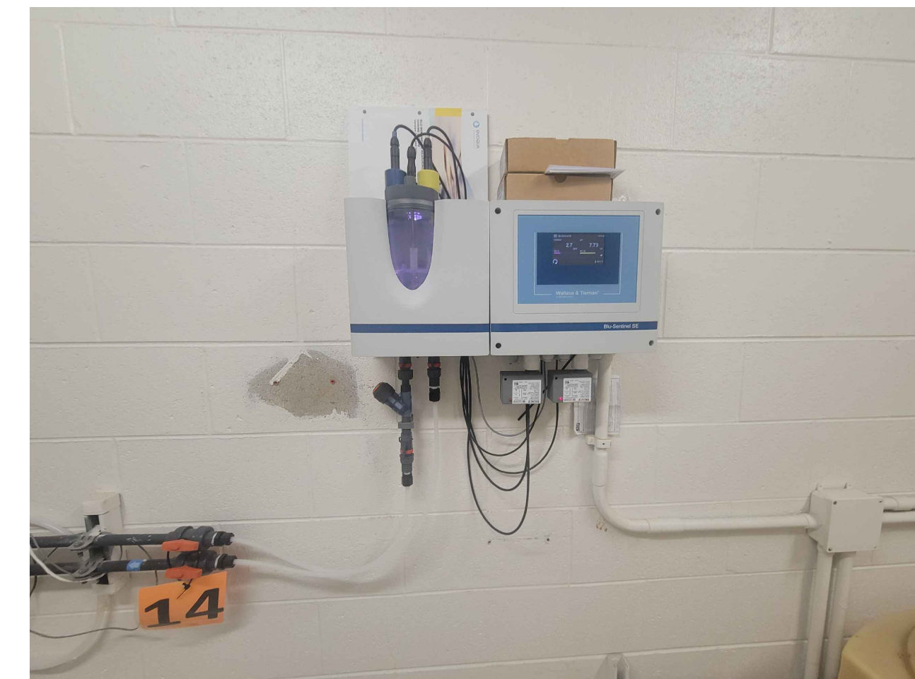
2 AQ0.3 EXISTING CHEMICAL CONTROLLER NTS
