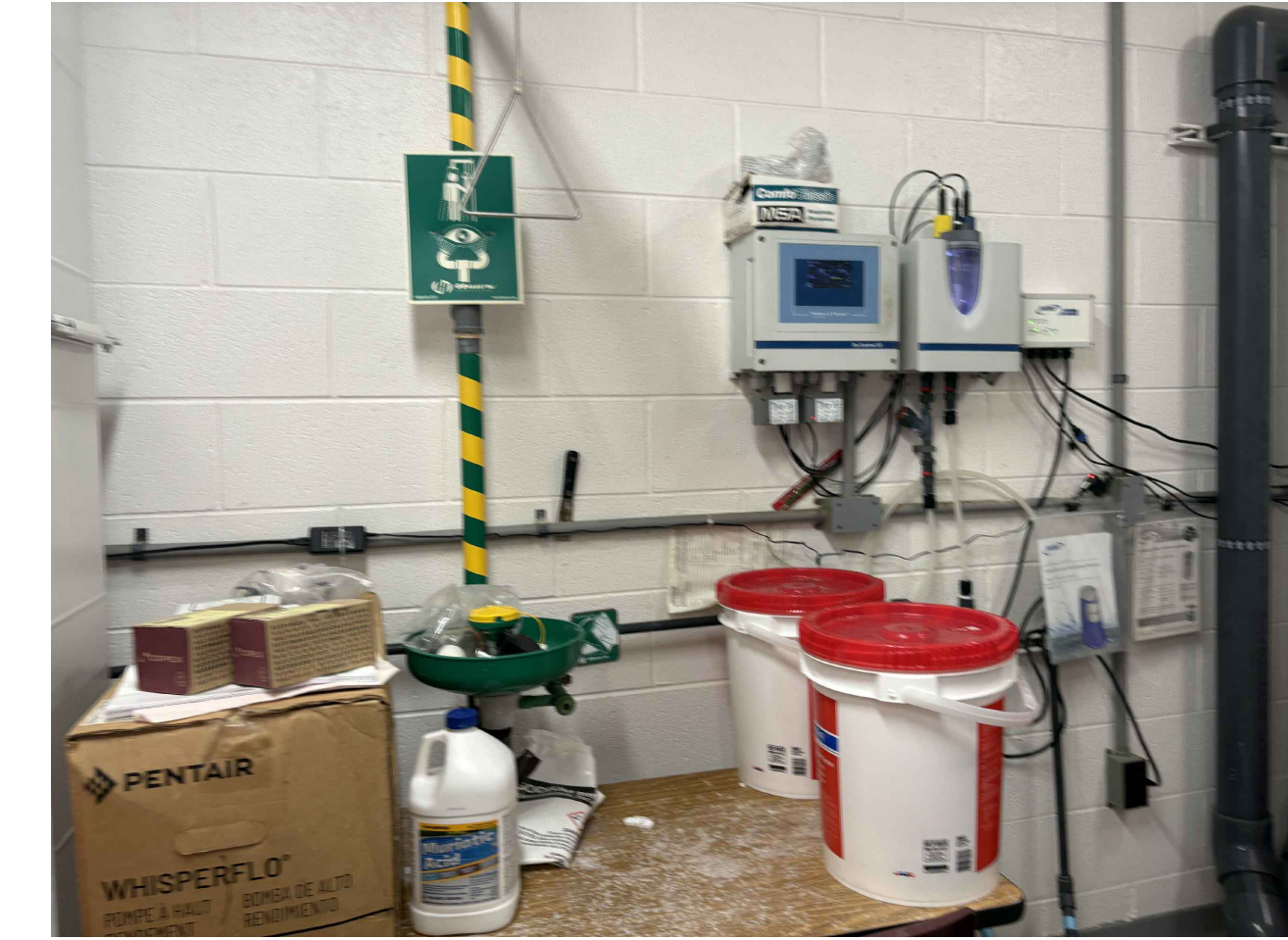
2 AQ0.3 EXISTING CHEMICAL CONTROLLER NTS
