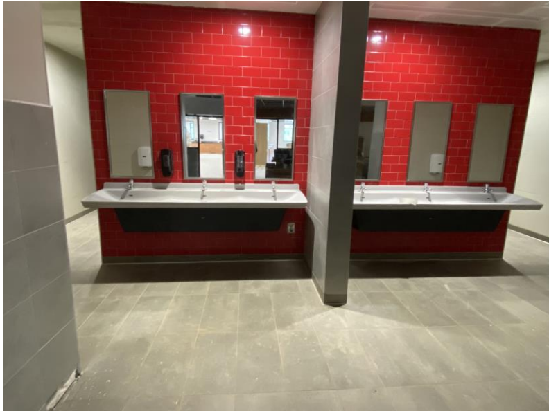
Gang Restroom Sinks in Area 3
