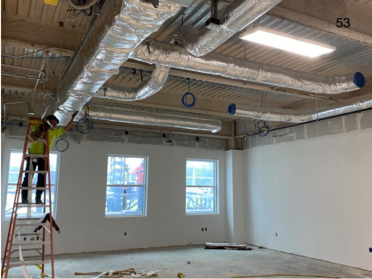
Ductwork Insulation on 2 nd Level
