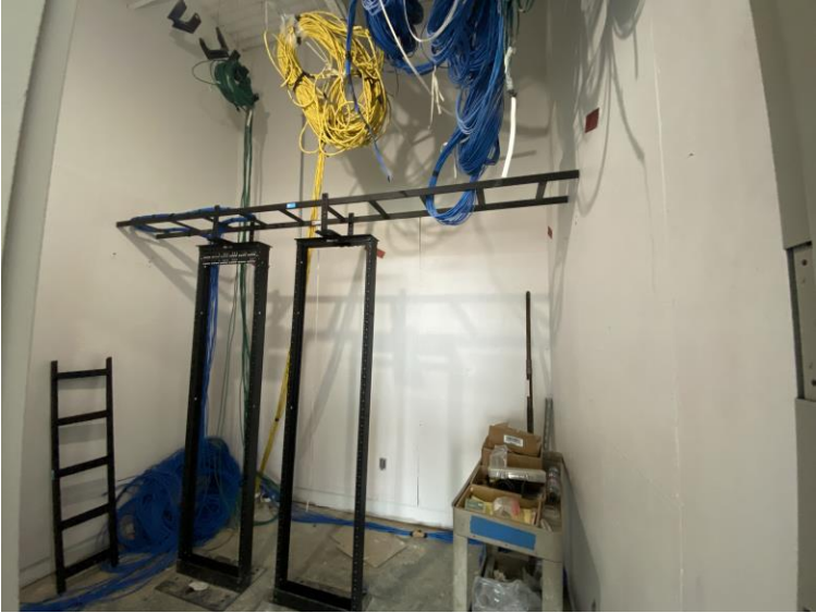
Racks Set in IDF on 2 nd Level
