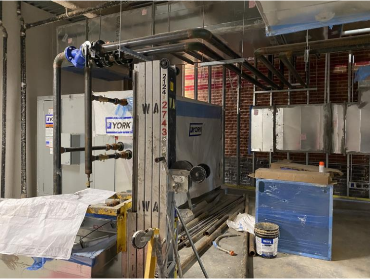
Air Handling Unit on 1 st Level
