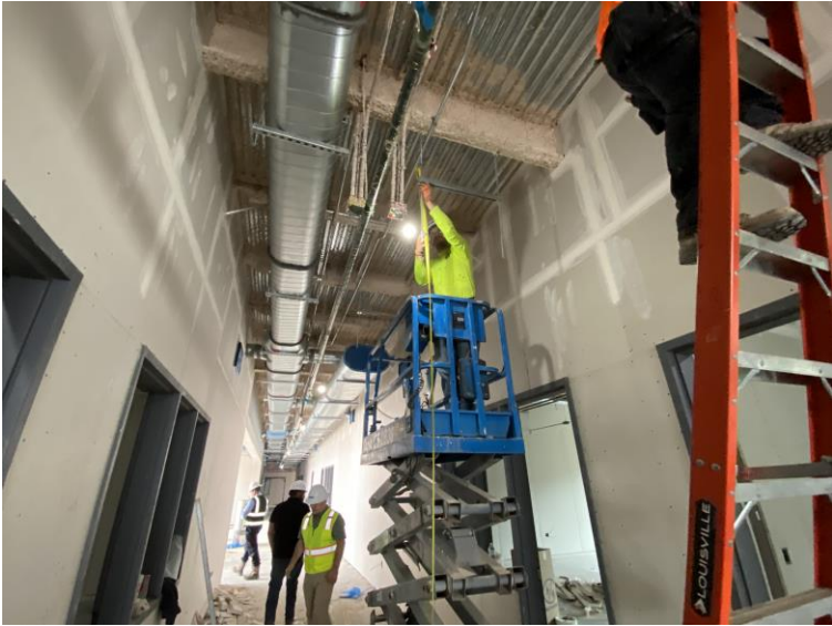
Unistrut for Ductwork on 2 nd Level
