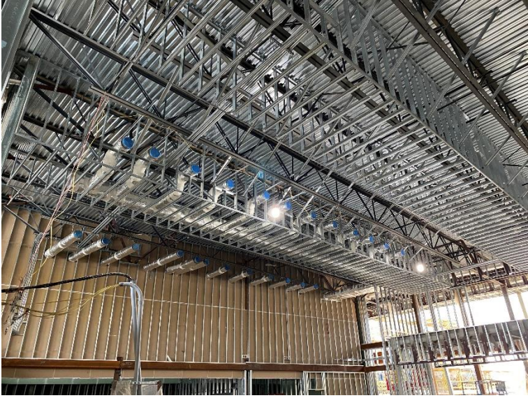
Overhead MEP in Library
