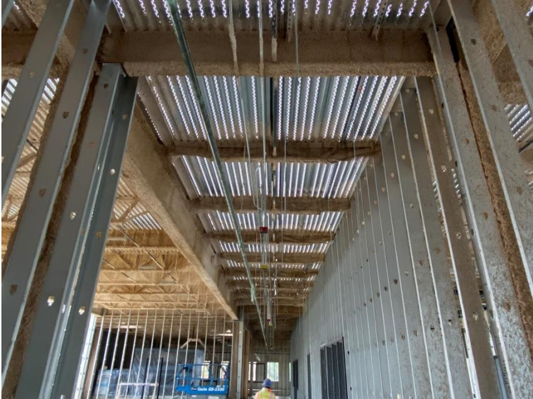
Overhead MEP in Corridor on 2 nd Level
