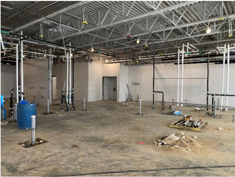
MEP in Serving Area
