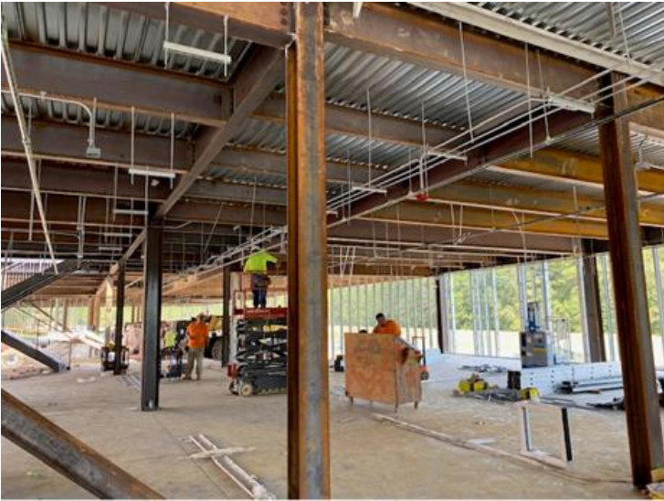
Overhead MEP on the 1 st Level
