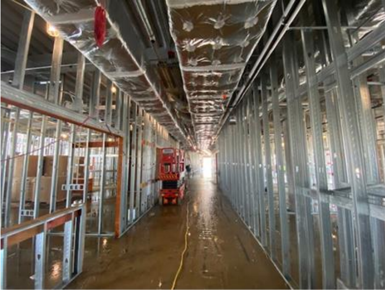
Insulated Overhead Ductwork in Area 2
