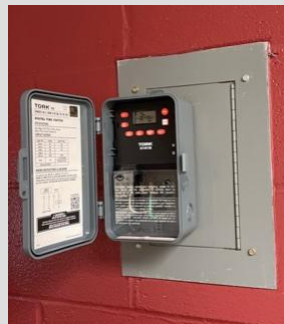
Lighting Time Clock
