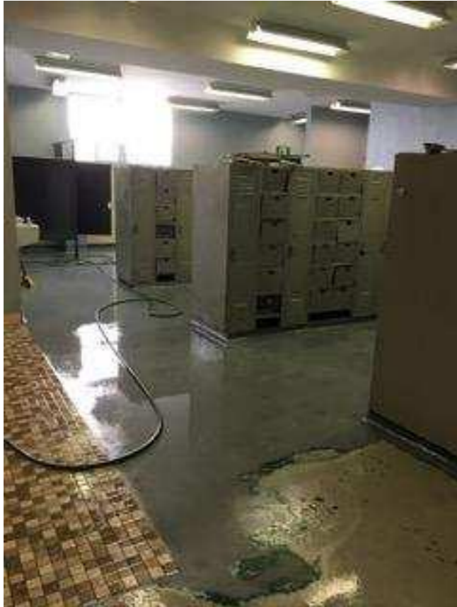
Early stages of floor stripping Note the multiple stacks of center lockers
