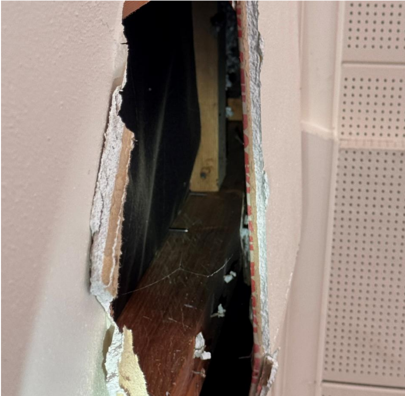
Photo #13 Looking Northeast. Refer to note #10 above. This recent framing is intriguing as it may indicate an intentional repair near the ceiling level.
