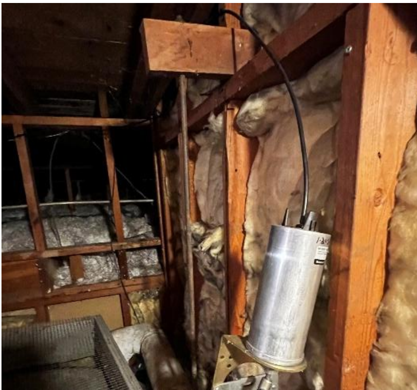
Photo #11,12 Looking Southwest. Indicates the mechanical equipment (lower left) in the mezzanine above the buckle.
