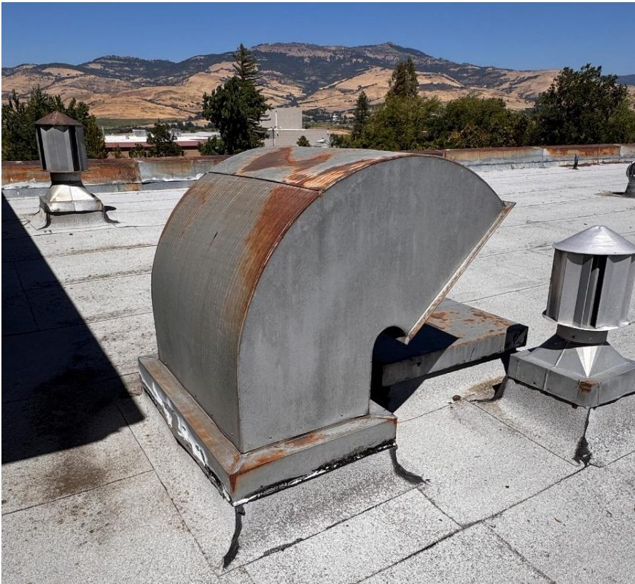
Photo #15. Looking Northeast. Refer to Photos #9 & #10. The corner of the Gymnasium that pops up above the corridor and the east wing is just to the left of this photo.
