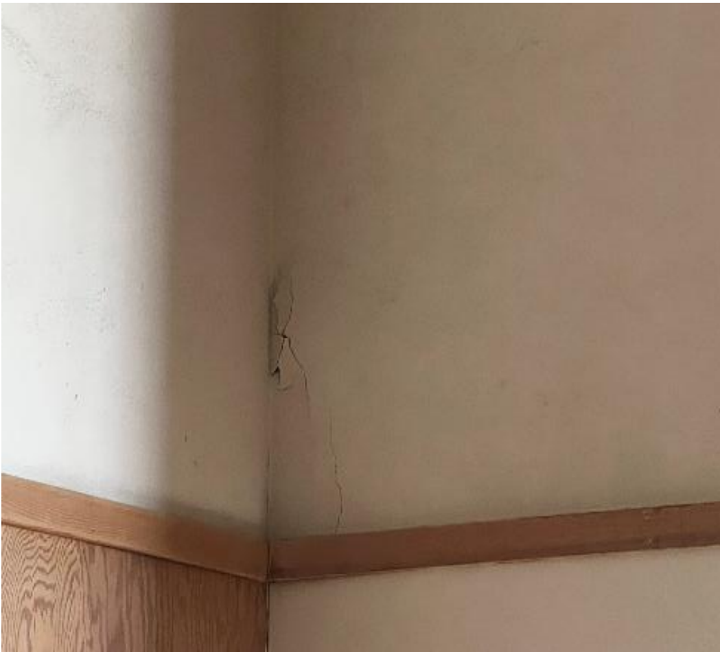
Photo #4 Looking west. This shows a plaster crack indicating minimal building movement.
