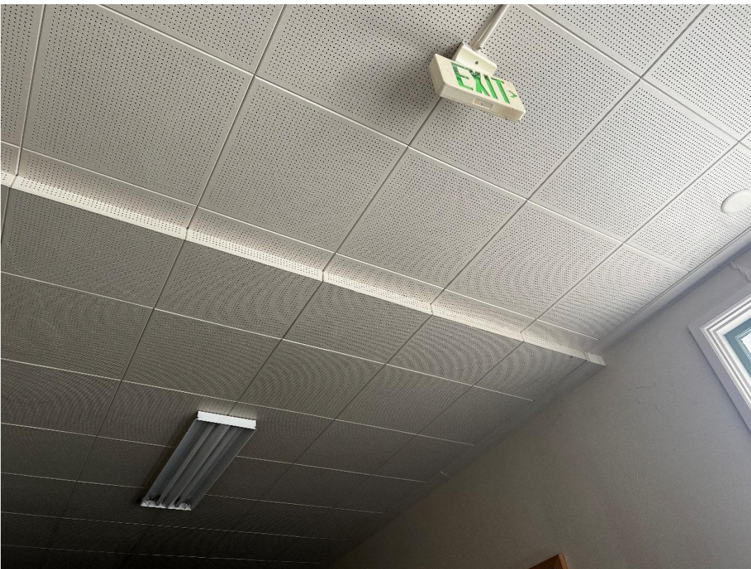
Photo #3 Looking Northwest, across the Corridor from the buckle. It indicates the purposeful change in the ceiling plane spanning the corridor.
