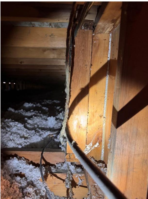
Photo #18. Looking West. This picture indicates a stooled-up frame wall running west the length of the gymnasium. It bears on the ceiling framing and continues up underneath the roof framing.
