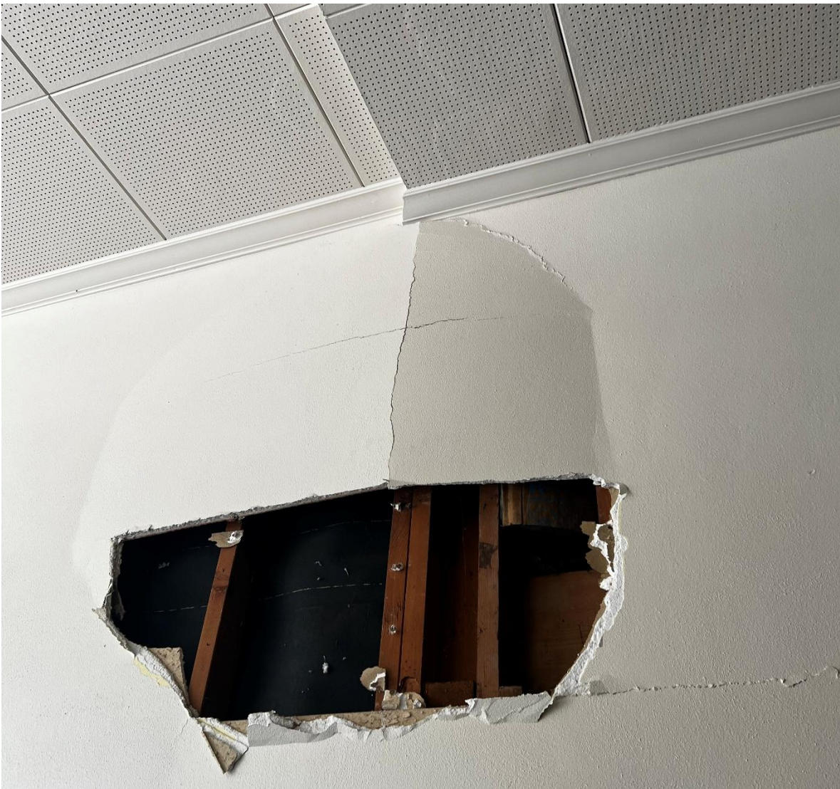
Photo #1 Looking North. Indicates the buckling of the Gypsum Wall Board(24"x36") in the Corridor adjacent to the Stage and the Teacher Work Room (per original blueprint).
