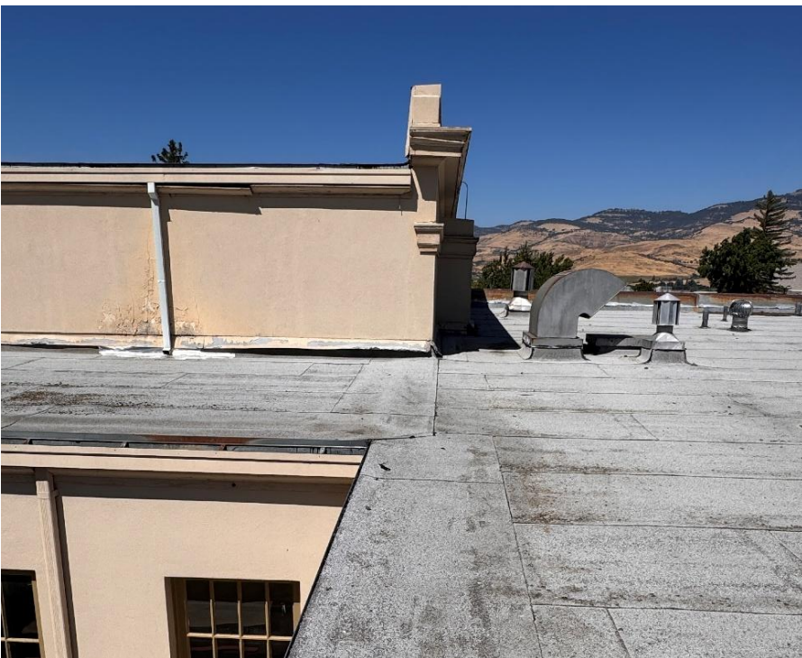
Photo #16. Looking North. Refer to Photos #9 and #10. Note the hump from this lower eave to the corner of the gym indicating movement. The buckle is directly below the corner of the gym.
