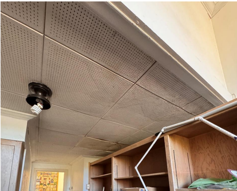
Photo #14 Looking Southwest. The buckle is on the outside of this wall. The water stains at acoustic ceiling may indicate water from outside or from the HVAC equipment in the mezzanine above.
