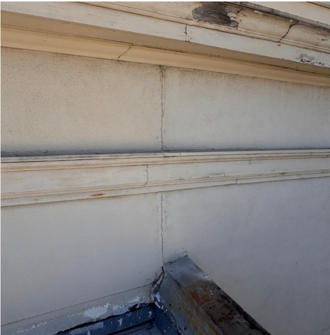
Photo #17. Looking Northwest. Refer Photos #9 and #10. This crack is at a location that is common to buildings indicating expected expansion and contraction.
