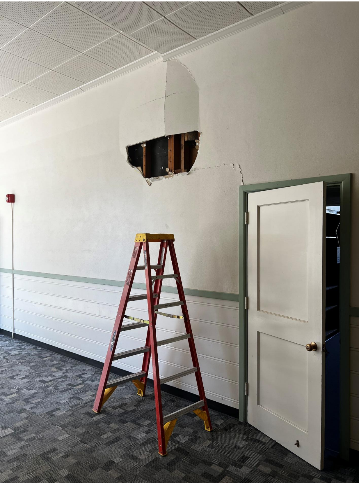
Photo #6 Looking Northeast. Indicates the context of the buckle outside of 'Teachers Break Room'(per original blueprint)
