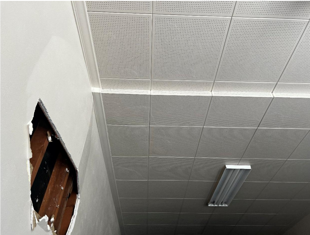
Photo #2 Looking Northeast. Indicates the buckling in the Gypsum Wall Board showing the depth out of plumb.
