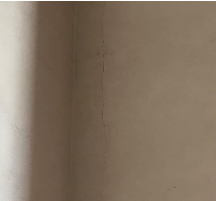
Photo #5 Looking west. This shows a plaster crack indicating minimal building movement.
