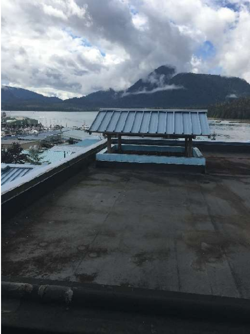
Mechanical ventilation pit
