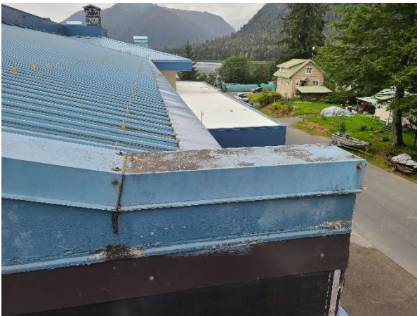
Water pooling on parapet cap
