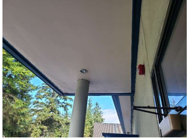
Blistering soffit paint
