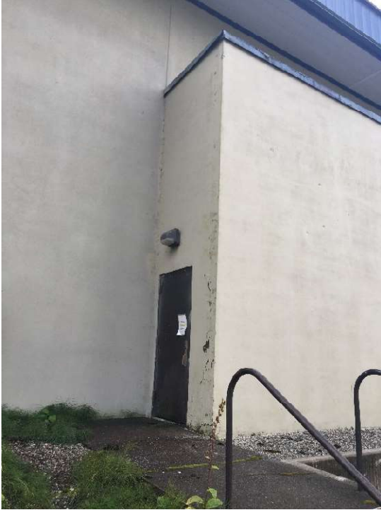
Water damage along the wall
