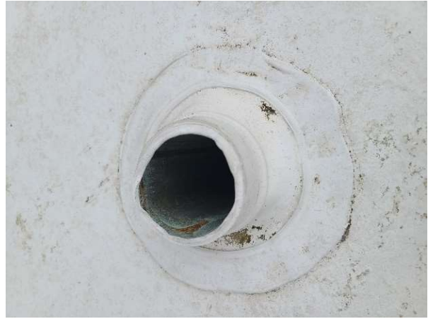
Low VTR serving as overflow drain
