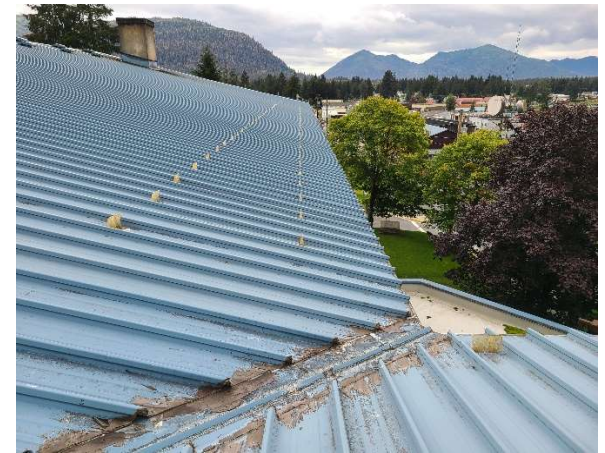
Past attempts to prevent water penetration
