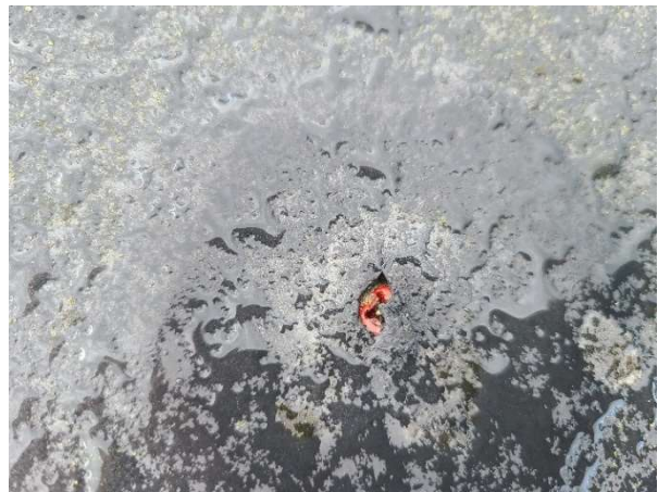
Bird damage at roof insulation fastener
