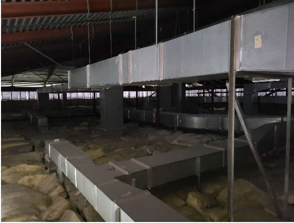
Uninsulated attic ductwork
