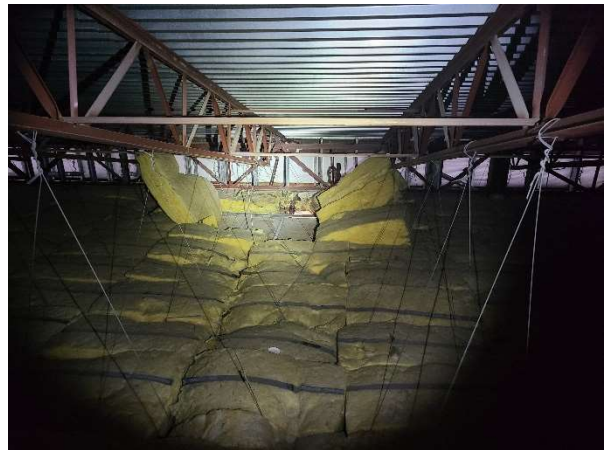
Attic insulation moved for leak repair
