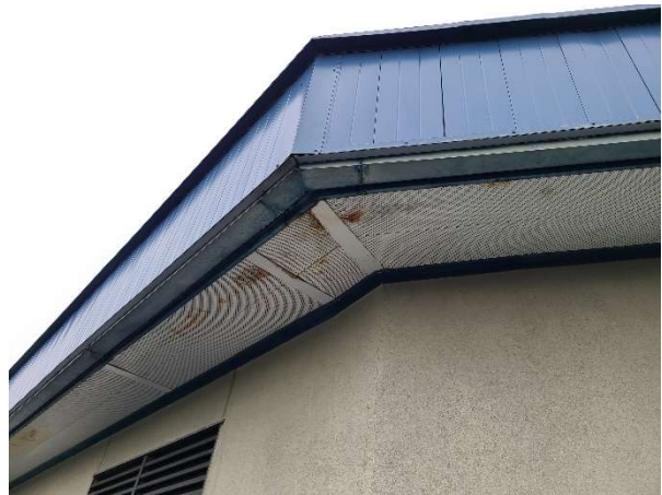
Soffit staining caused by roof leaks
