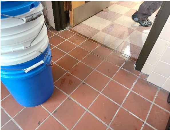
Ongoing roof leak
