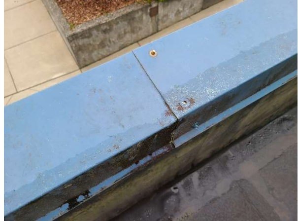
Screws missing from top of parapet cap
