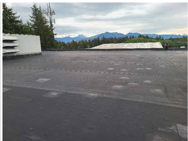
Bird damage patches
