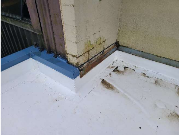
Wall damage due to ice dam
