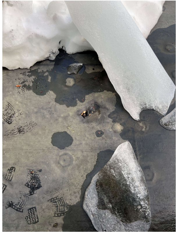
EPDM puncture caused by falling ice
