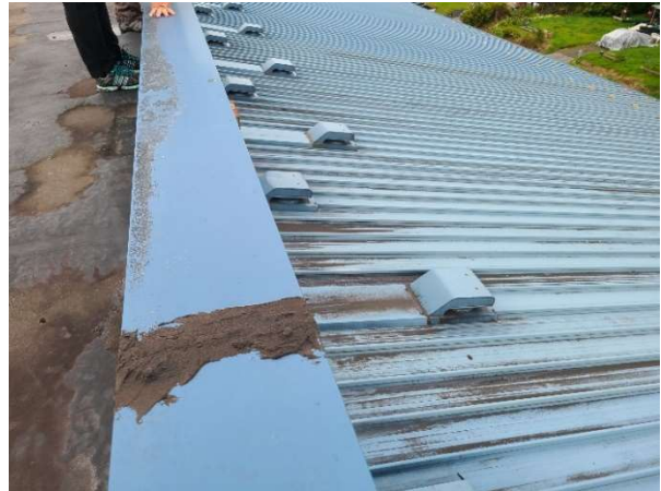
Past attempts at mitigating water penetration
