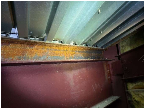
Water damage at roof deck joint
