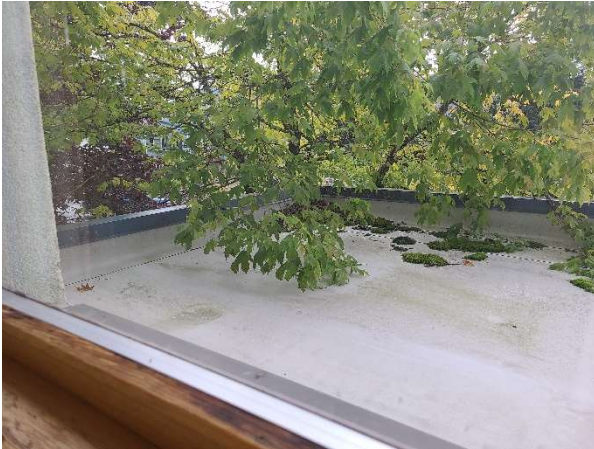
Tree leaning on roof membrane
