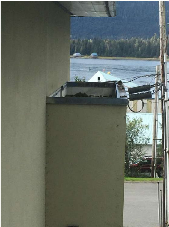
Dented parapet cap
