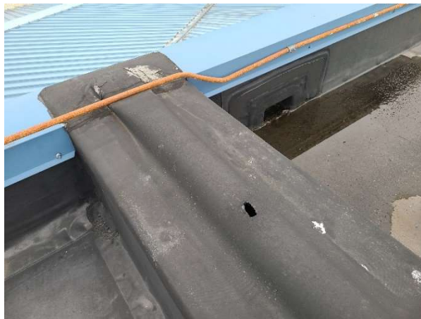
Bird damage at seismic joint
