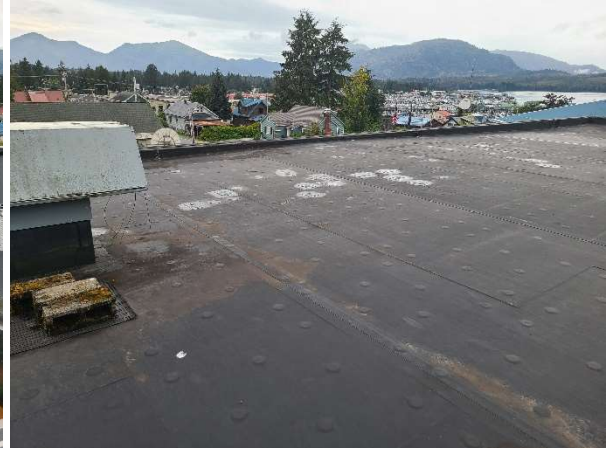
Bird damage patches
