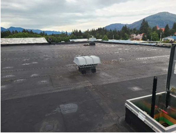
Bird damage patches
