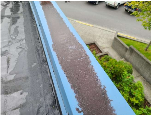
Parapet cap water pooling
