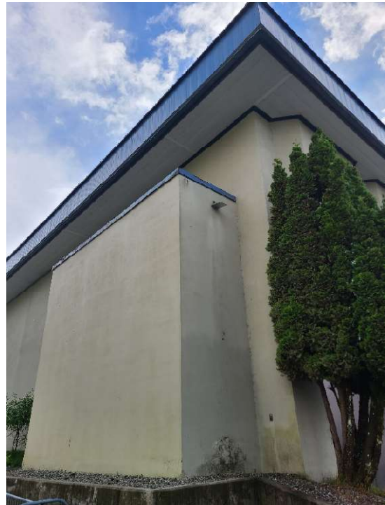
Water damage at scupper discharge
