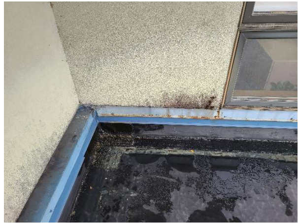
Wall damage due to ice dam
