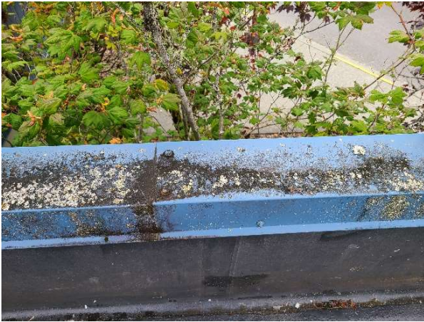
Parapet water pooling
