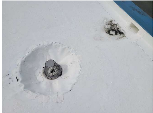
Roof drain and overflow scupper
