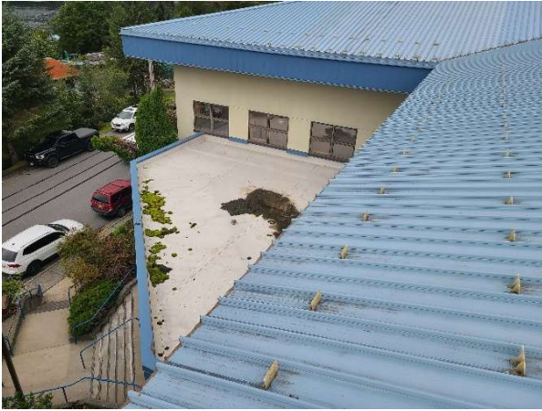
Roof C and D shedding on Roof A
