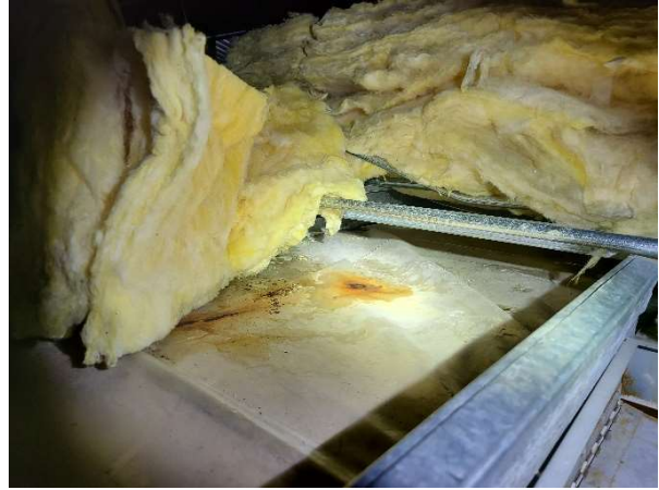
Water pooling on top of vapor barrier
