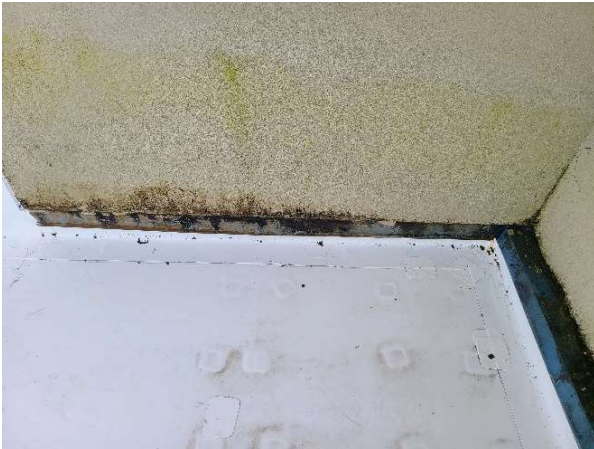
Wall damage due to ice dam
