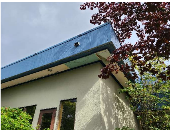
Soffit damage near roof drain
