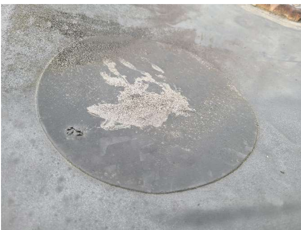
Bird damage in recent patch
