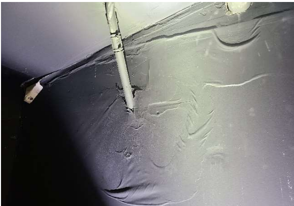
Evidence of past water leaks
