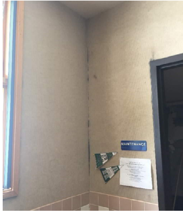
Figure 21- Nook Wall Crack
