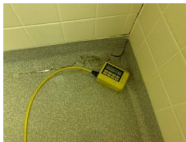
Figure 13- 2020 Boys Bathroom Floor
