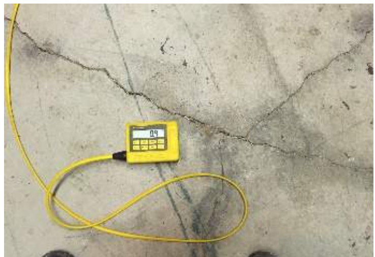
Figure 9- Cracks near Loading Dock Doors
