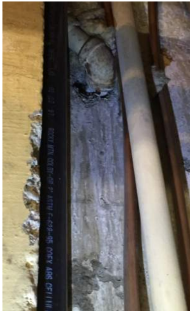
Figure 24- 2018 Water Stain by Pipe Penetration
