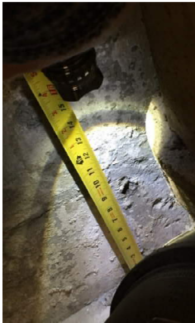
Figure 21- 2018 Hole in Wall
