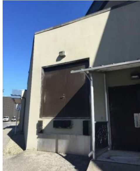
Figure 18- 2018 Northwest Wall of Addition, West Column
