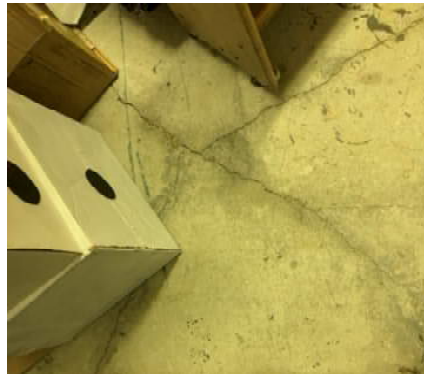
Figure 15- 2020 Storage Room Crack
