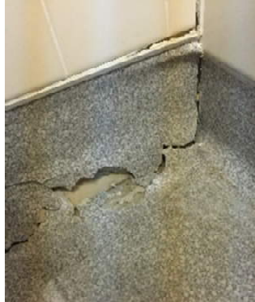
Figure 6- Boys Bathroom Floor
