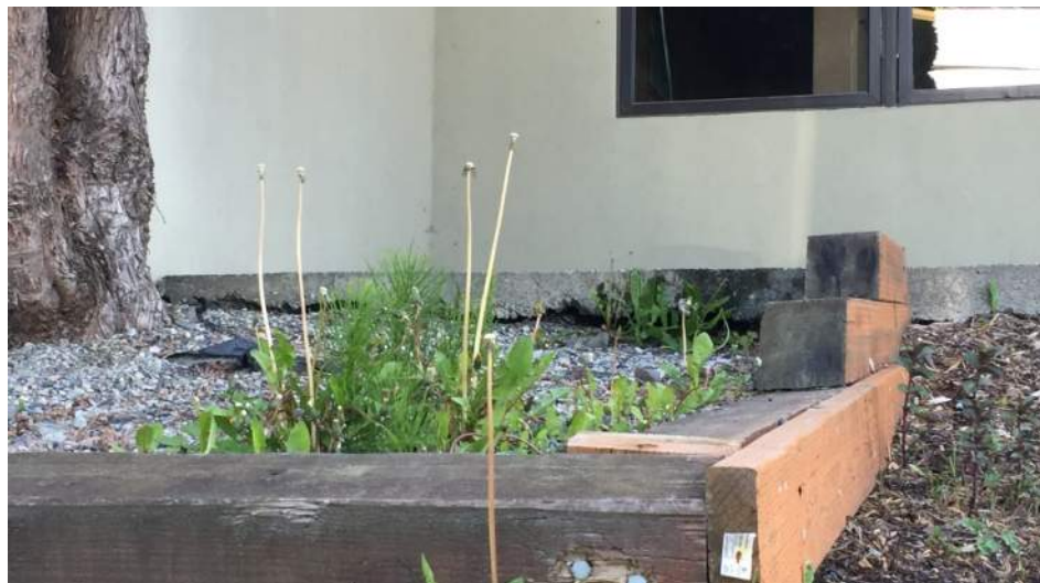
Figure 22- Exterior Slab Undermined
