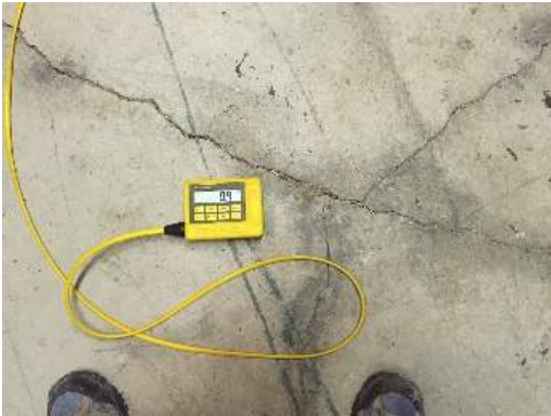
Figure 14- 2018 Storage Room Crack
