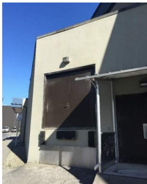
Figure 15- Northwest Wall of Addition, West Post
