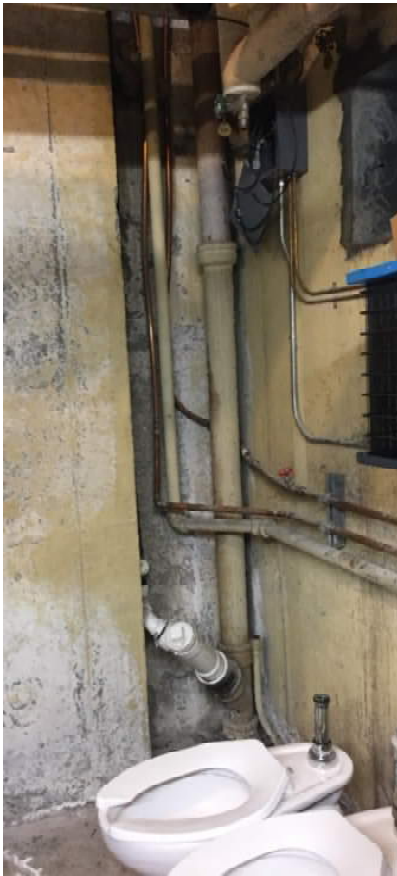
Figure 16- Nook with the Leak
