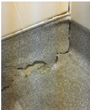
Figure 12- 2018 Boys Bathroom Floor
