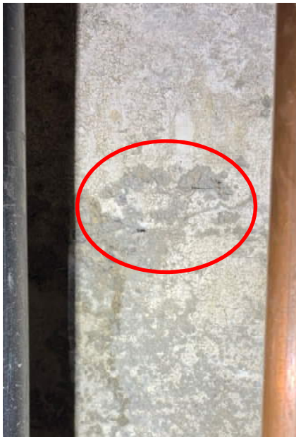
Figure 23- 2020 Damage in Concrete Wall
