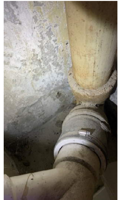
Figure 22- 2020 Hole in Wall
