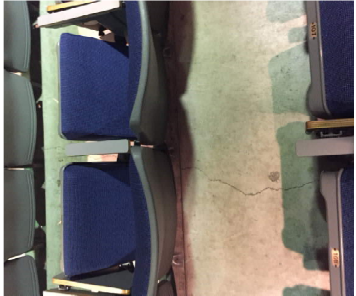
Figure 1- Crack in the Risers
