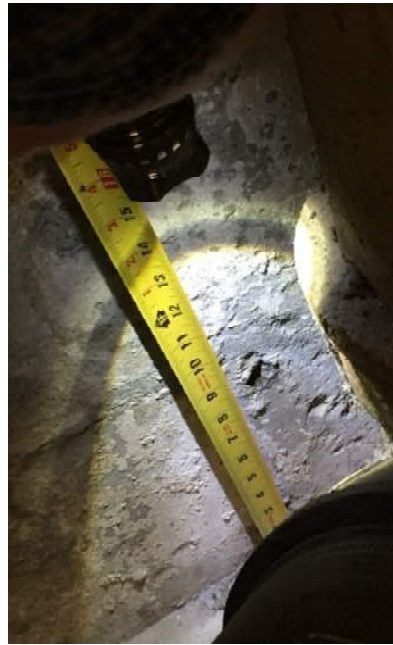
Figure 17- Hole in Wall
