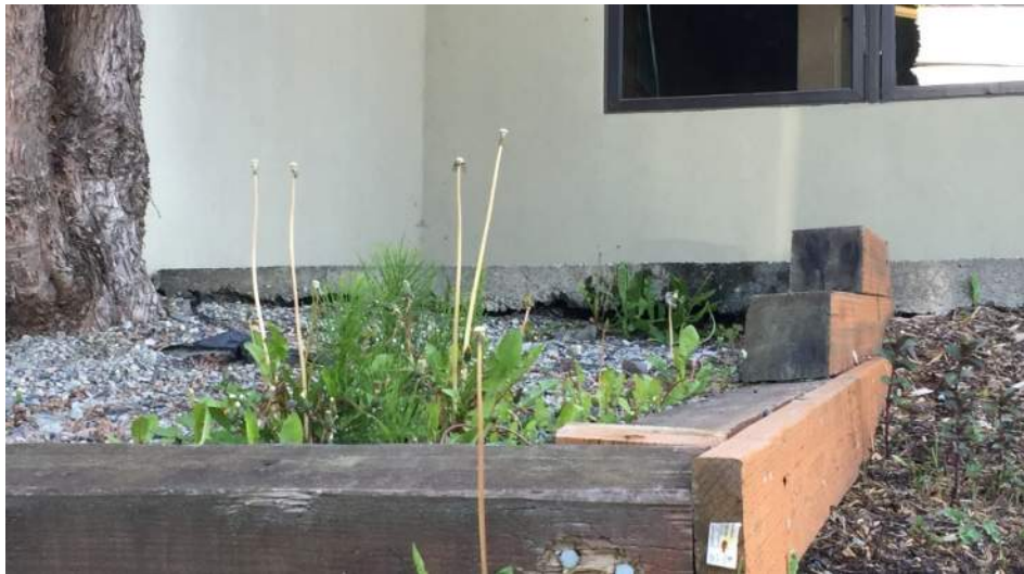
Figure 22- Exterior Slab Undermined
