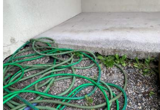
Figure 28- 2020 Exterior Slab Undermined
