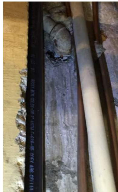
Figure 24- 2018 Water Stain by Pipe Penetration
