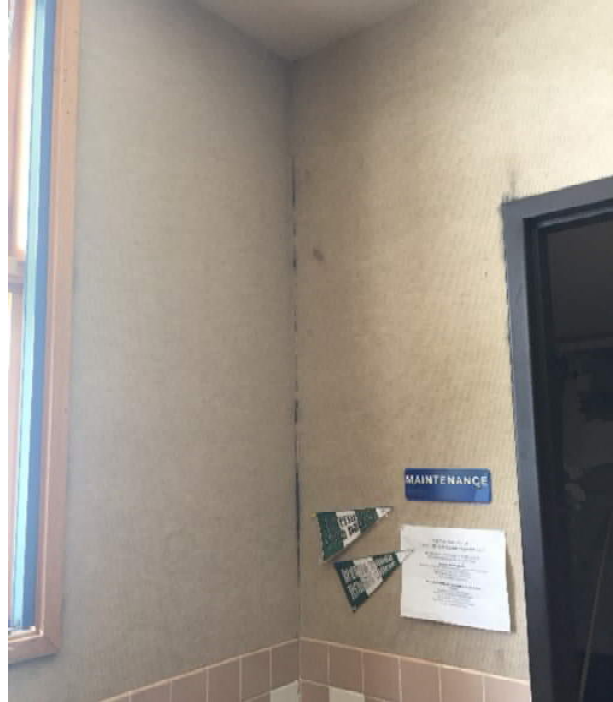
Figure 21- Nook Wall Crack
