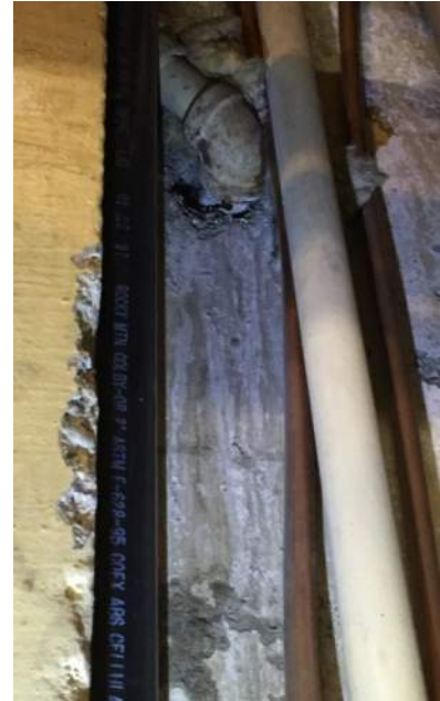
Figure 18- Pipe Hole Leak
