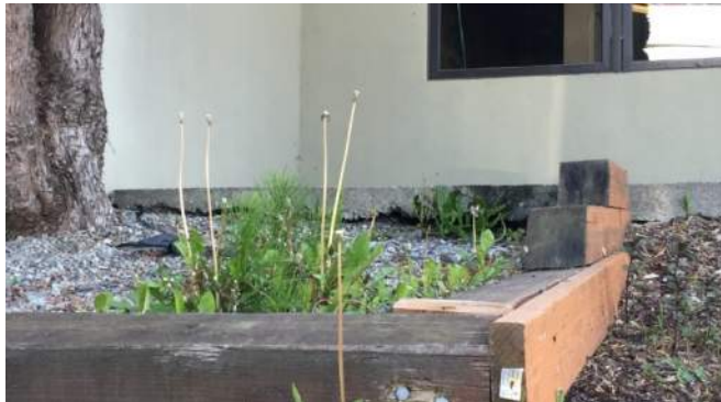
Figure 27- 2018 Exterior Slab Undermined
