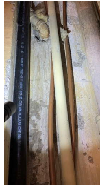
Figure 25- 2020 Water Stain by Pipe Penetration
