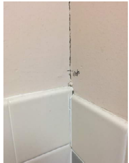
Figure 4- Girls Bathroom Wall
