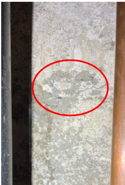
Figure 23- 2020 Damage in Concrete Wall
