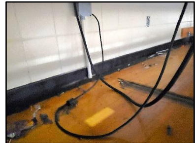
Loose power cables.
