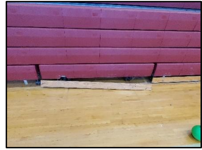
Damaged/loose skirt boards.
