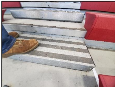
Loose intermediate aisle step.
