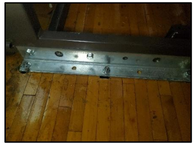
Floor anchor attachment.
