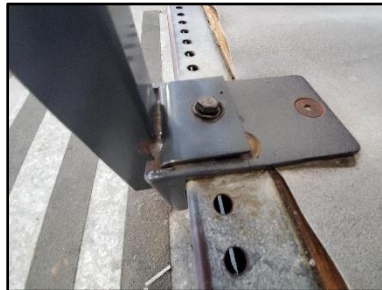
Loose aisle rails.
