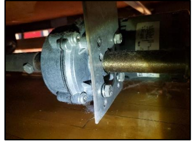
Loose & missing motor mount fasteners.
