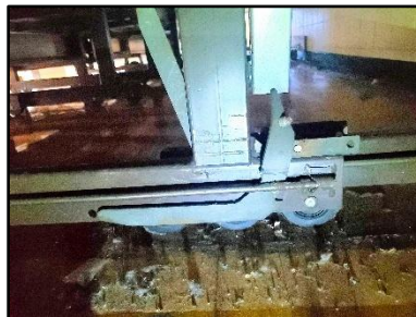
Damaged & non actuating row locks.
