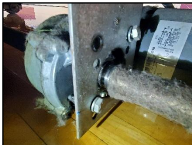
Loose/missing motor mount fasteners.
