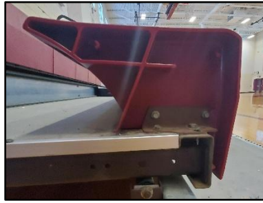
Loose & missing end caps.
