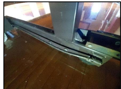
Damaged slide rods.
