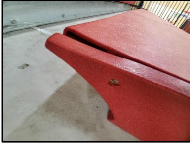
Loose & damaged end cap.
