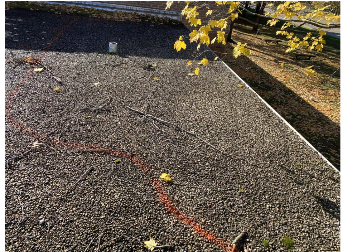
ANOTHER AREA THAT WAS FOUND TO BE WET
