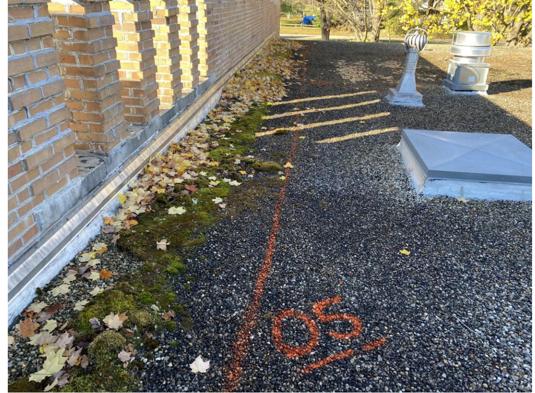
WET AREA THAT WAS IDENTIFIED
