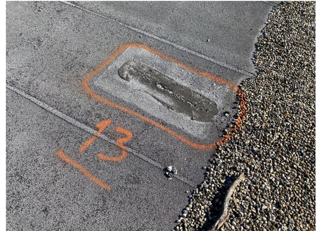
PREVIOUS REPAIR AREA WAS ALSO IDENTIFIED AS WET
