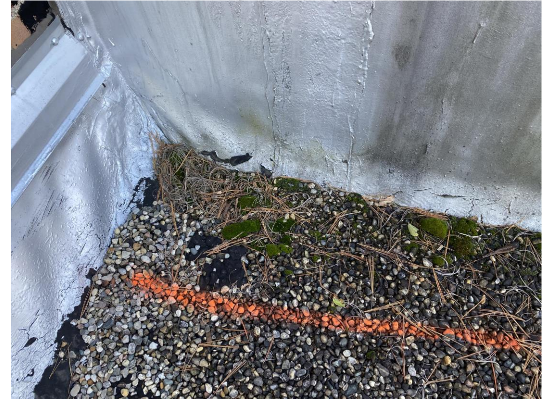
WET INSULATION IDENTIFIED
