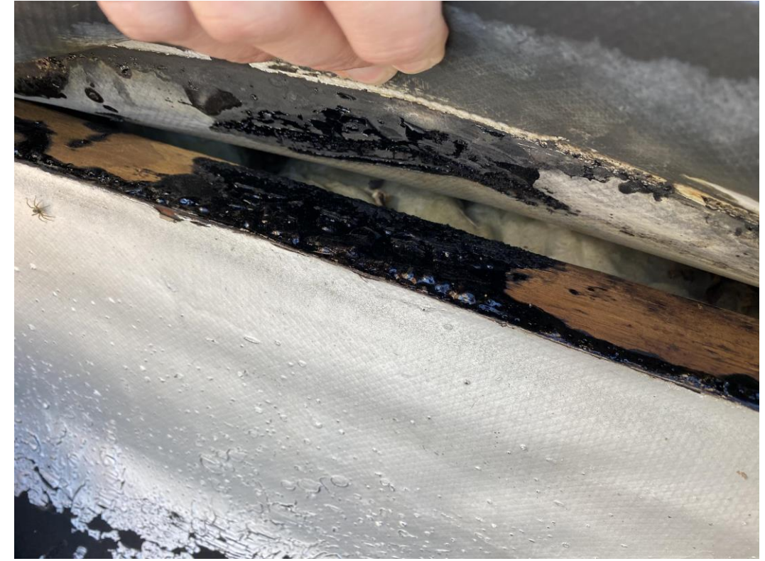
POOR DETAILSHIP ON THE EXPANSION JOINT
