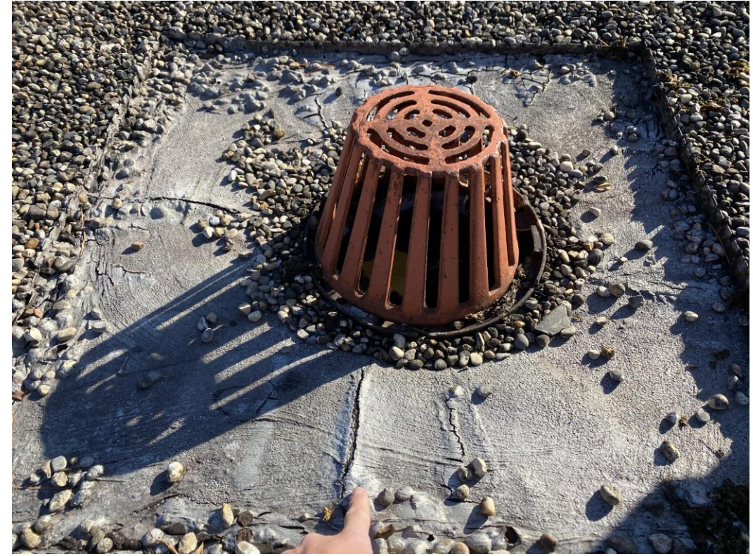
CRACKING IN THE MEMBRANE AROUND THE DRAIN
