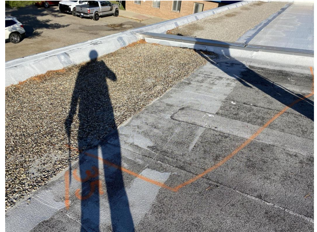
LARGE WET AREA WAS FOUND IN THE VALLEY AREA. THE SATURATION IS STARTING TO MIGRATE UP THE ROOFING SYSTEM
