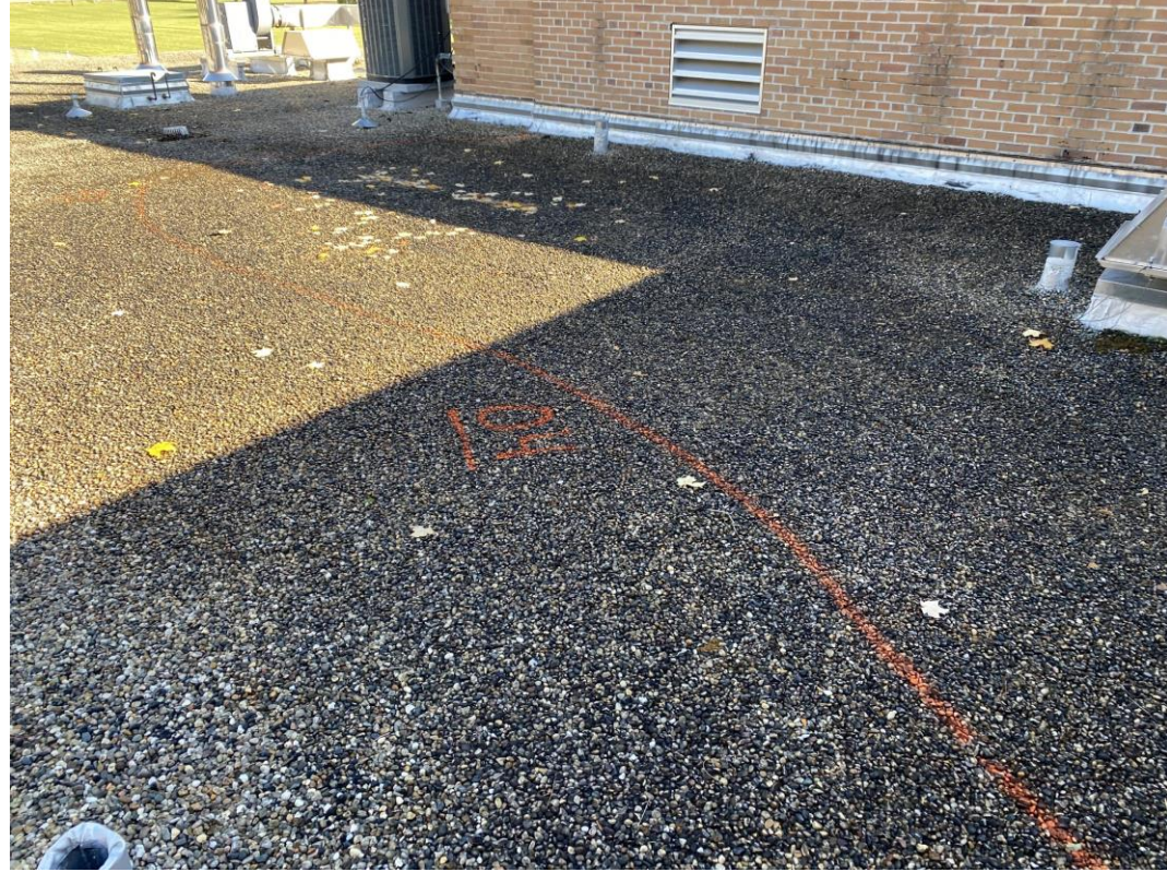
SECTION #13 OVERVIEW AND WET AREA THAT WAS FOUND
