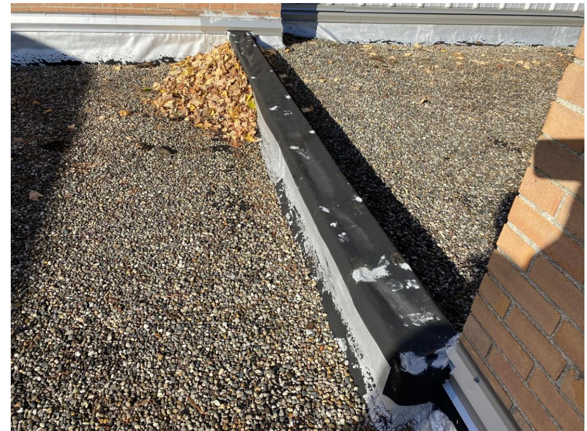
POOR CONTROL JOINT / EXPANSION JOINT DETAIL.
