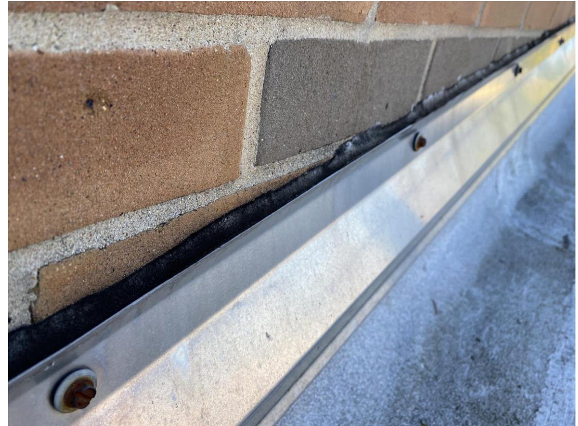
CAULKING ABOVE THE COUNTER-FLASHING IS STARTING TO FAIL IN SOME AREAS
