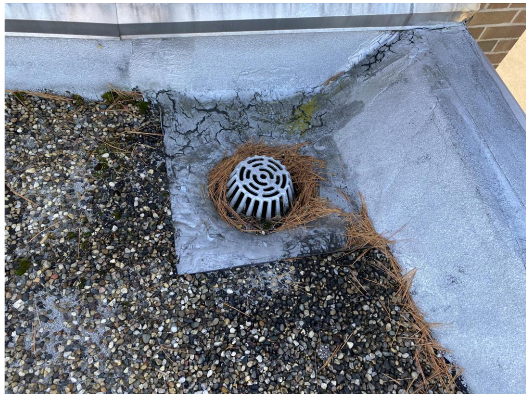
DRAIN OVERVIEW WITH DEBRIS AROUND THE STRAINER.
