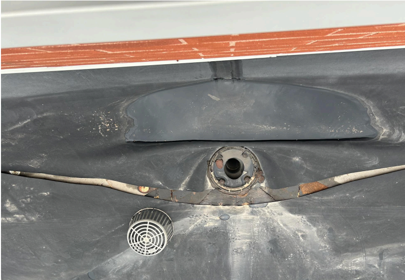
Tears in the rubber membrane throughout parts of the roof.
