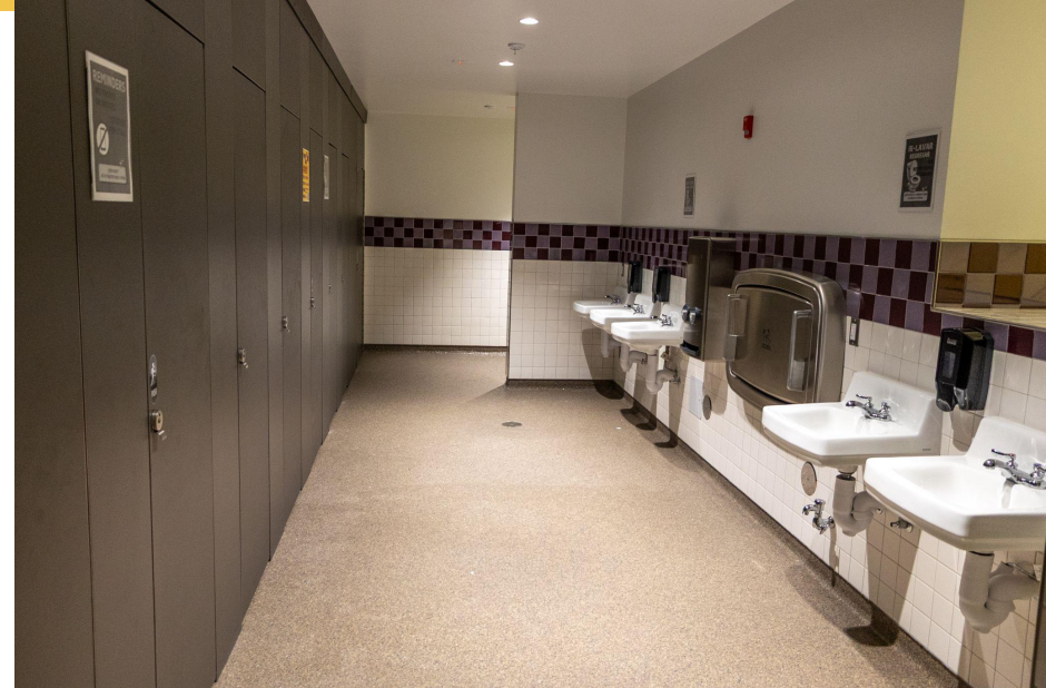
All-user restrooms at Sunset HS (left) and Whitford MS (above). 51
