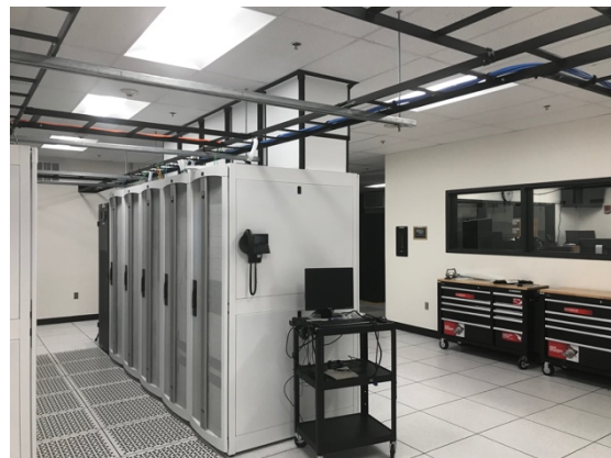
Figure 1: Capital Center Data Center
