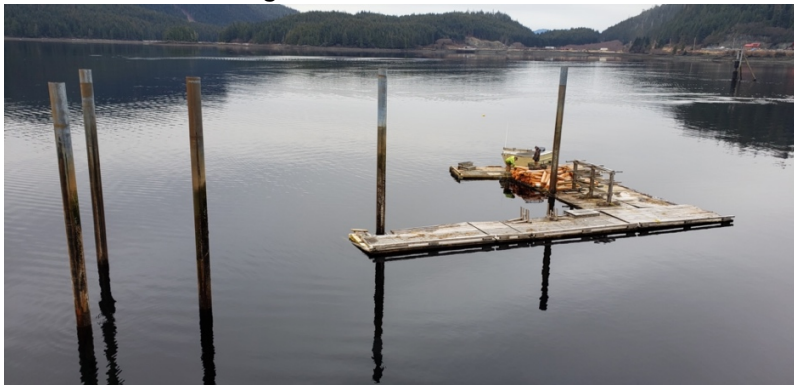
Picture of Metal Pilings and Dock Parts
