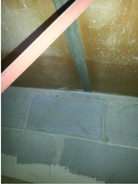
Photo 17 – Lounge: Moisture on Ceiling
