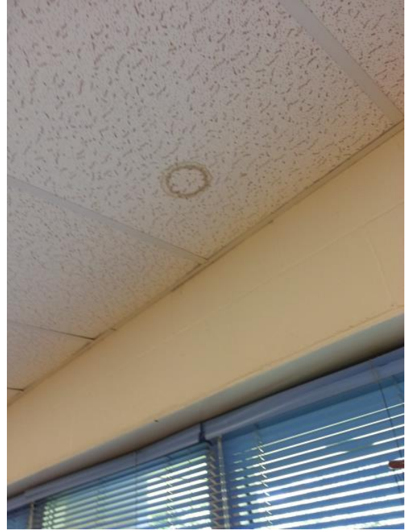
Photo 26 – Room 135 Water stain on ceiling tile
