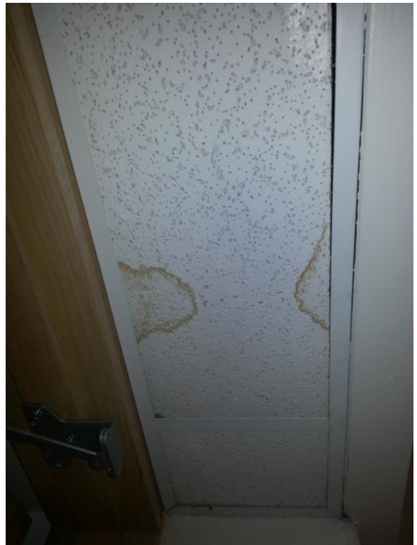
Photo 4 – Room 125 Stained Ceiling Tile
