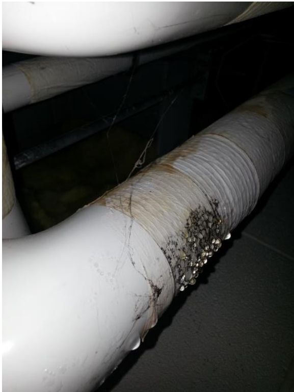
Photo 31 – Room 135 Condensation and water damage on pipe above ceiling
