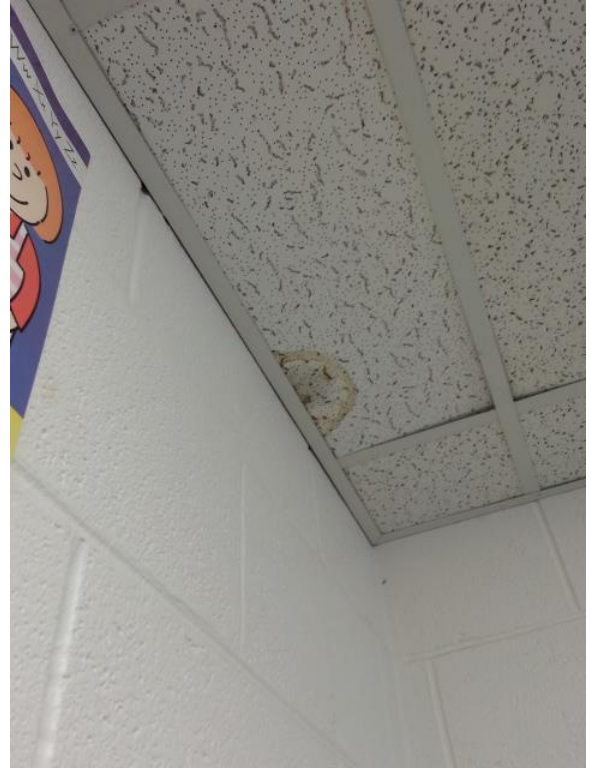
Photo 42 – Room 136 Stained ceiling tile
