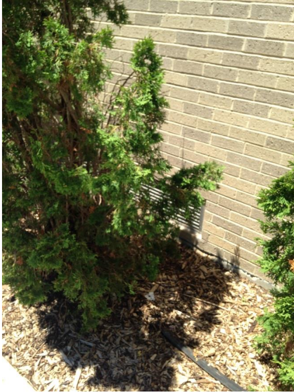
Photo 57 – Outside room 134, partially obstructed exhaust grille
