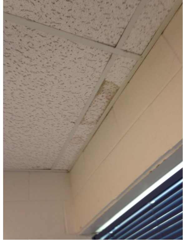
Photo 74 – Room 144, water stained ceiling tile
