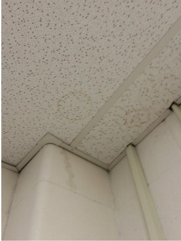
Photo 41 – Room 138 Water stained ceiling tile
