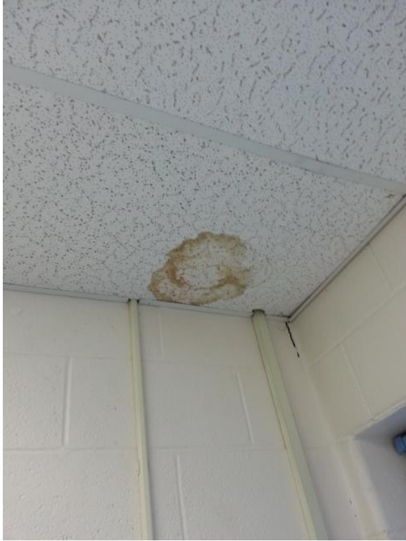
Photo 21 – Room 133 Water Stain on ceiling tile
