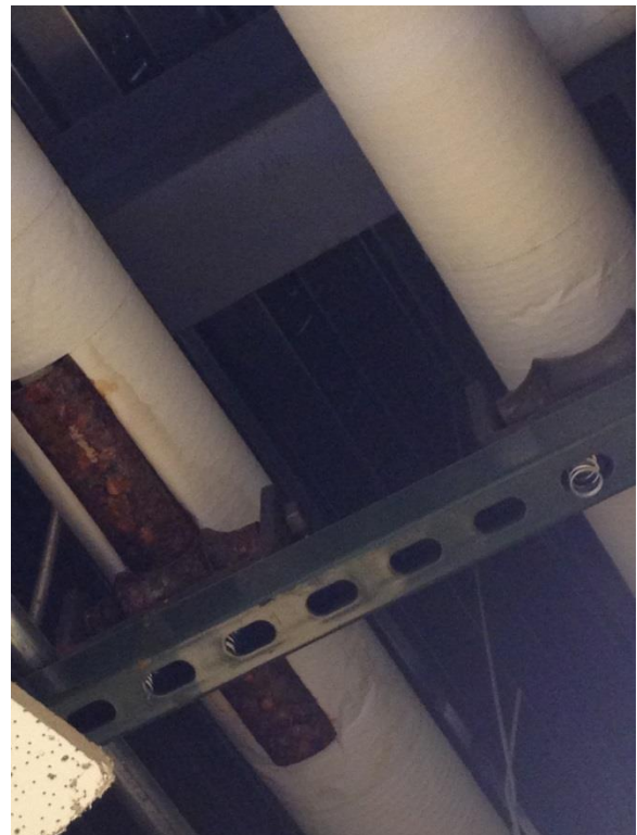
Photo 72 – Room 142, condensation and water damage on pipes
