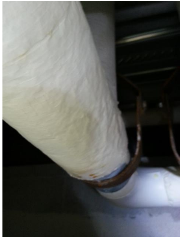
Photo 40 – Room 138 Damaged pipe
