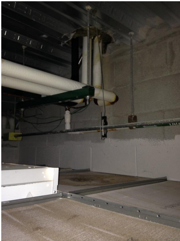
Photo 67 – Room 141, stained/damaged pipe above ceiling tile
