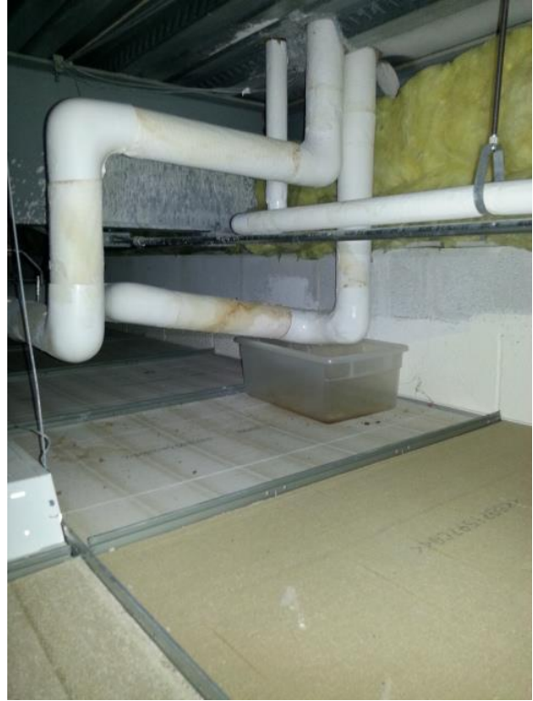
Photo 34 – Room 137 Water damaged pipe
