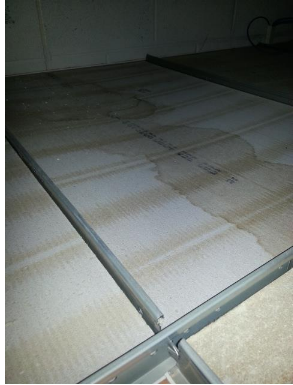
Photo 22 – Room 133 Stain on reverse of ceiling tile
