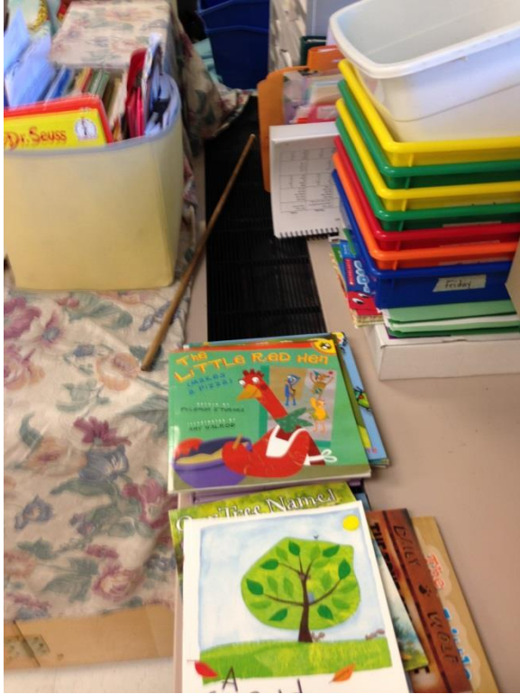
Photo 61 – Room 139 - Obstructed uni-vent
