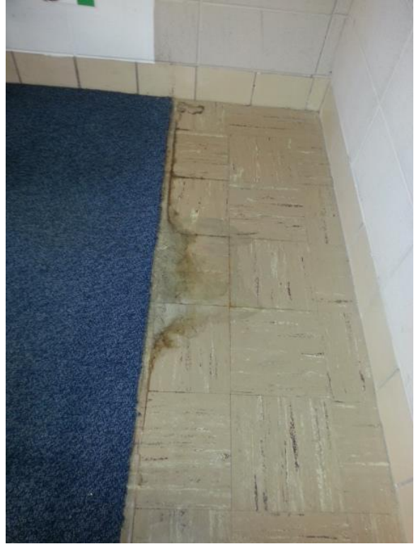
Photo 6 – Room 125 stained tiles under removed cabinets
