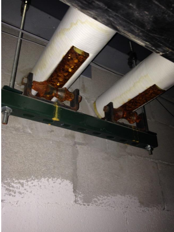
Photo 69 – Zone 5/SW hallway, damaged Pipe/condensation on supports
