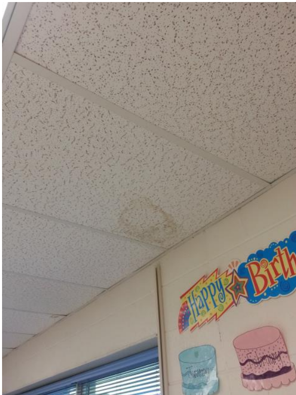
Photo 19 – Room 133 Water Stain on ceiling tile
