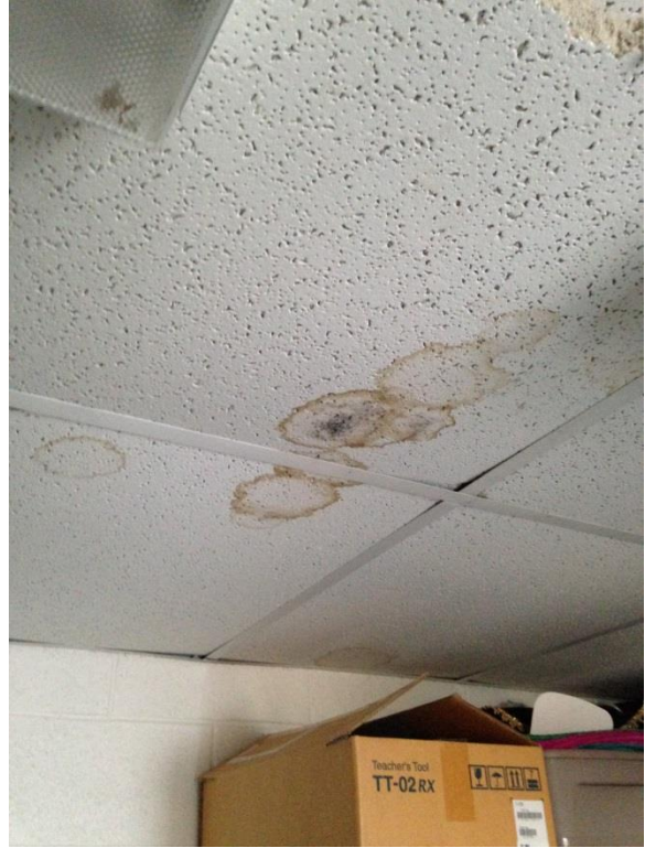
Photo 50 – Library Storage Stain and mold on ceiling tile
