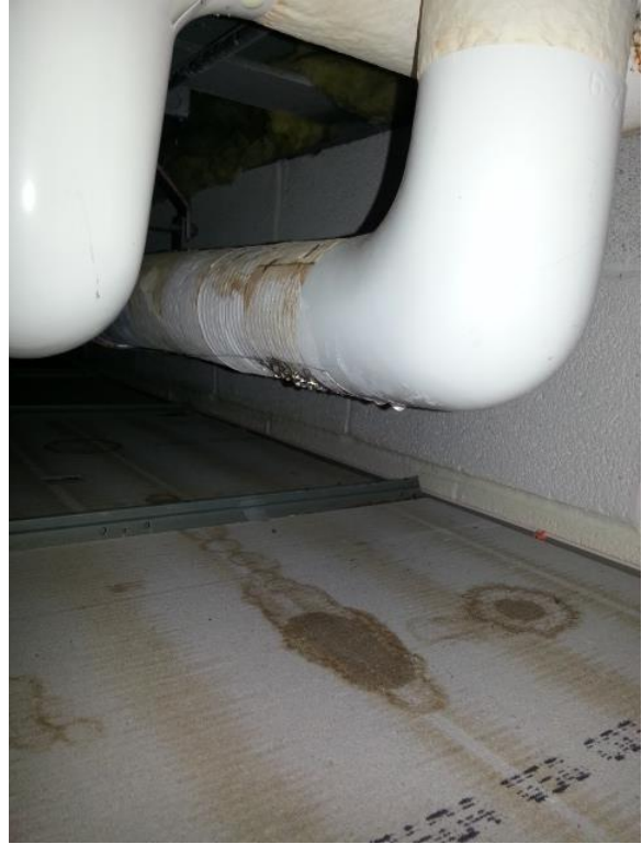
Photo 30 – Room 135 leaking pipes above ceiling
