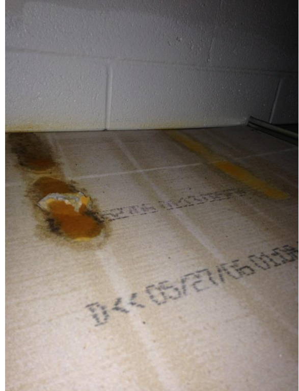
Photo 70 – Zone 5/SW hallway, damage on ceiling tile above supports
