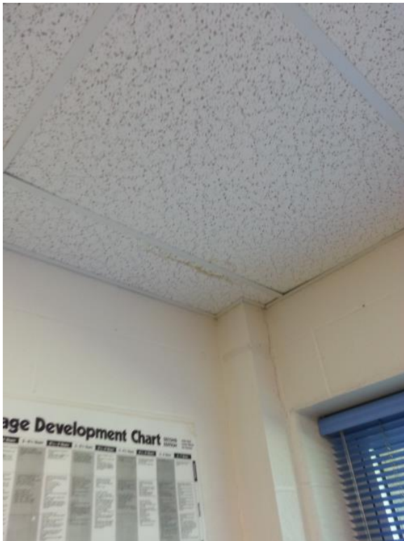
Photo 27 – Water stain on ceiling tile
