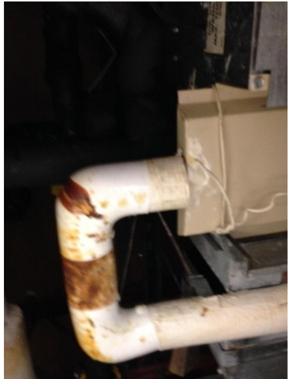
Photo 52 – Library Storage, damaged pipe above ceiling tile
