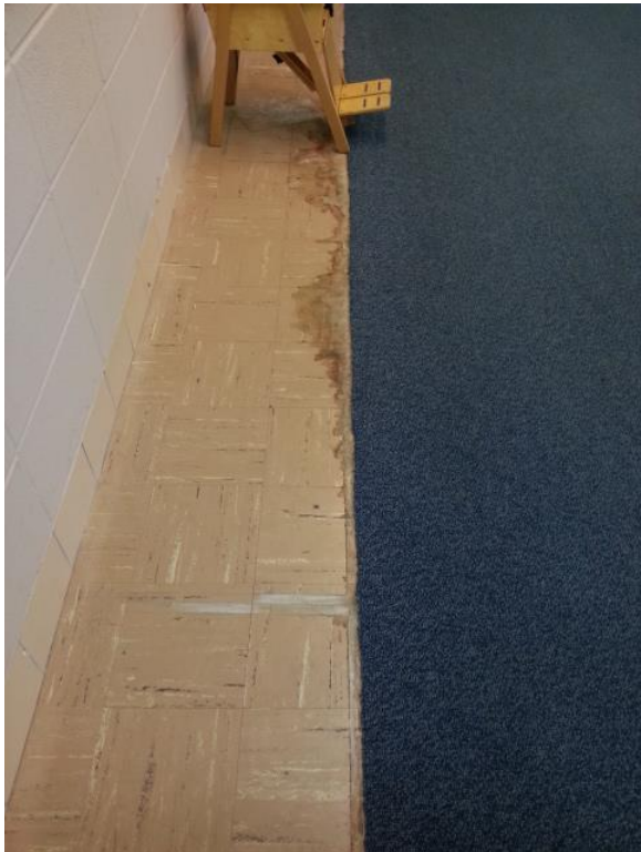
Photo 7 – Room 125 stained tiles under removed cabinets
