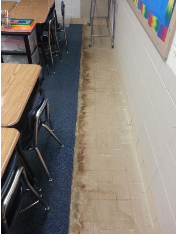
Photo 13 – Room 122 stains under removed cabinets
