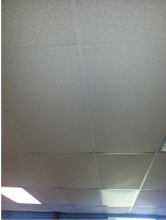
Photo 5 – Room 125 Bowed Ceiling Tiles
