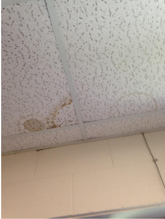
Photo 73 – Room 144, Water stained ceiling tile
