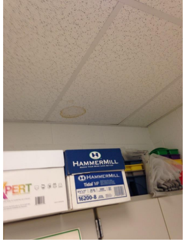
Photo 62 – Room 139, stain on ceiling tile
