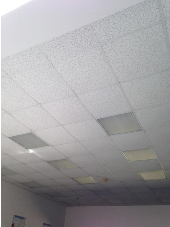
Photo 49 – Library ceiling, slightly bowed ceiling tiles
