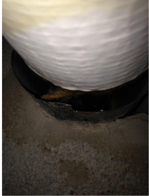
Photo 46 – Room 134 above ceiling, gap in insulation, moisture
