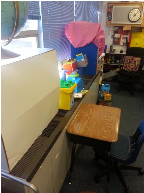
Photo 11 – Room 122 Obstructed uni-vent
