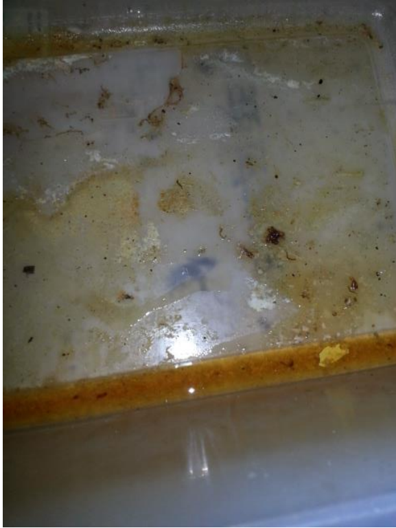
Photo 37 – Room 137 Interior of water collection tub underneath pipe
