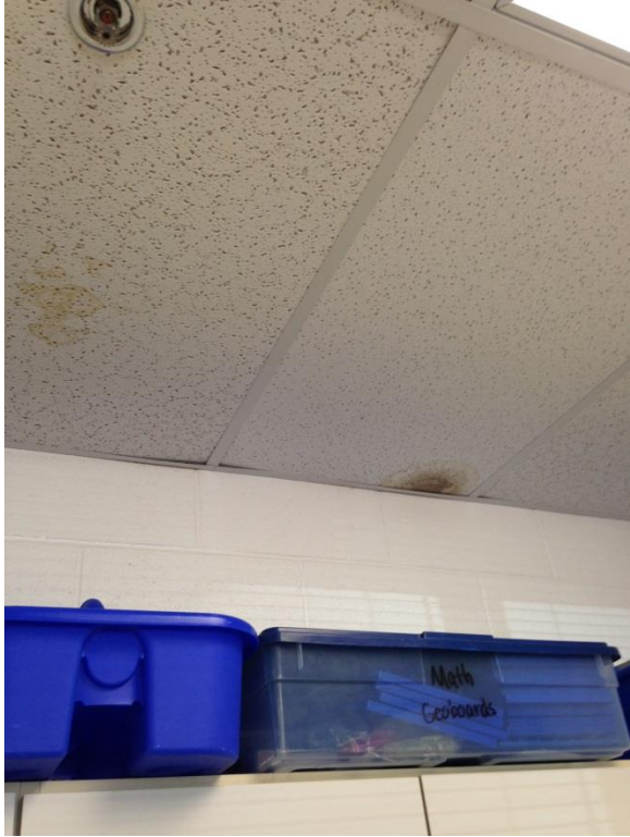
Photo 45 – Room 134 Water stain on ceiling tile
