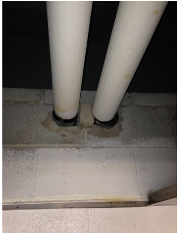
Photo 48 – Room 134 gap in insulation, moisture
