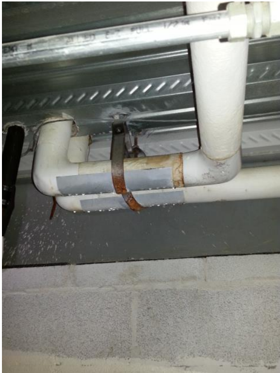
Photo 39 – Room 138 Damaged pipe with condensation
