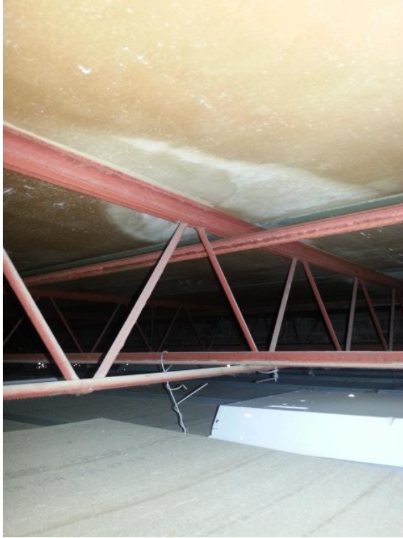
Photo 9 – Room 125 above drop ceiling – discoloration on gypsum board decking
