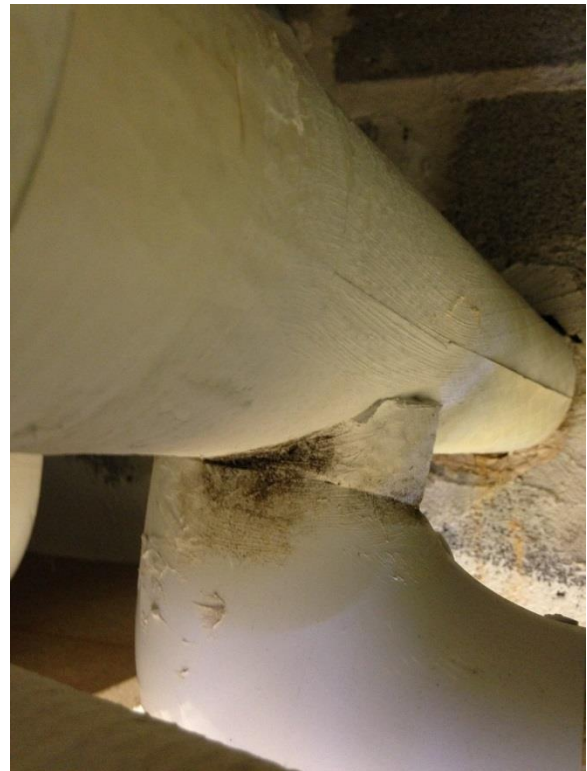
Photo 64 – Room 139 suspect growth on pipe above ceiling tile
