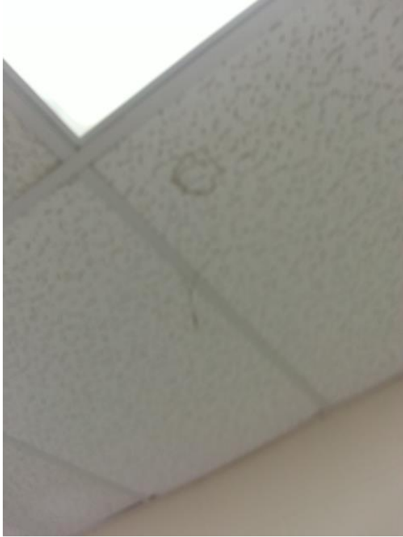
Photo 33 – Room 137 Stained ceiling tile
