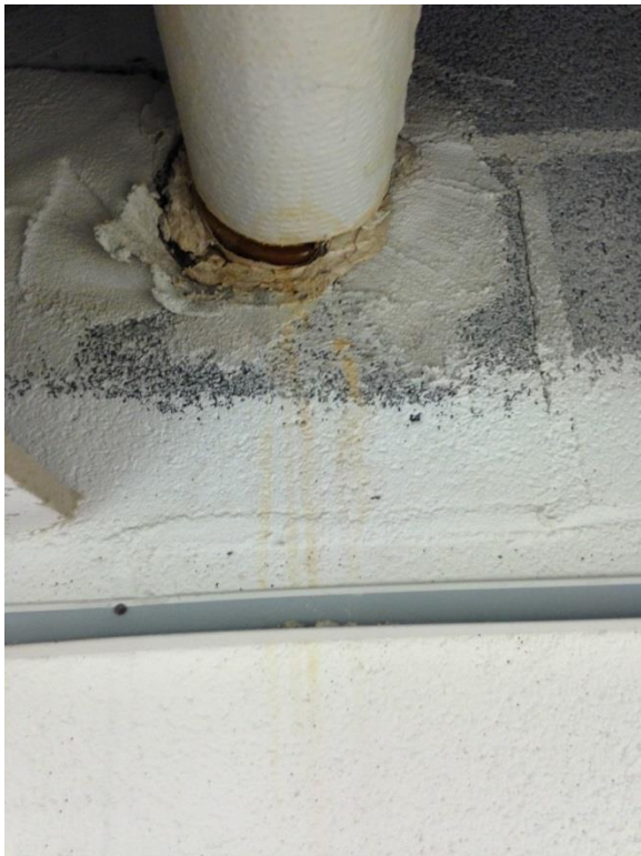
Photo 63 – Room 139, stains and gap in insulation
