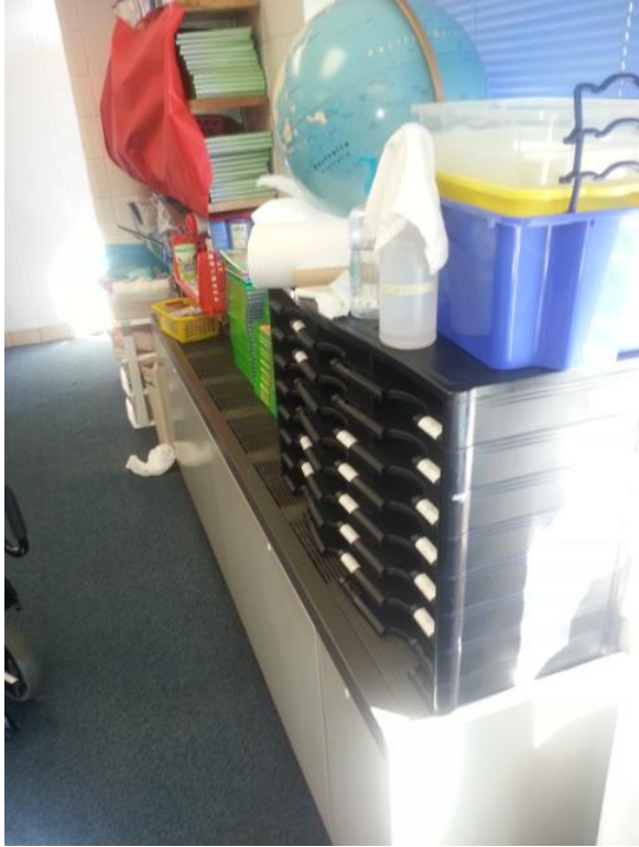
Photo 1 – Room 124 Obstructed uni-vent
