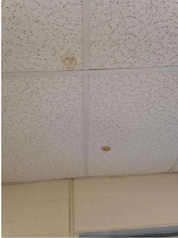
Photo 65 – Room 140, stained ceiling tile
