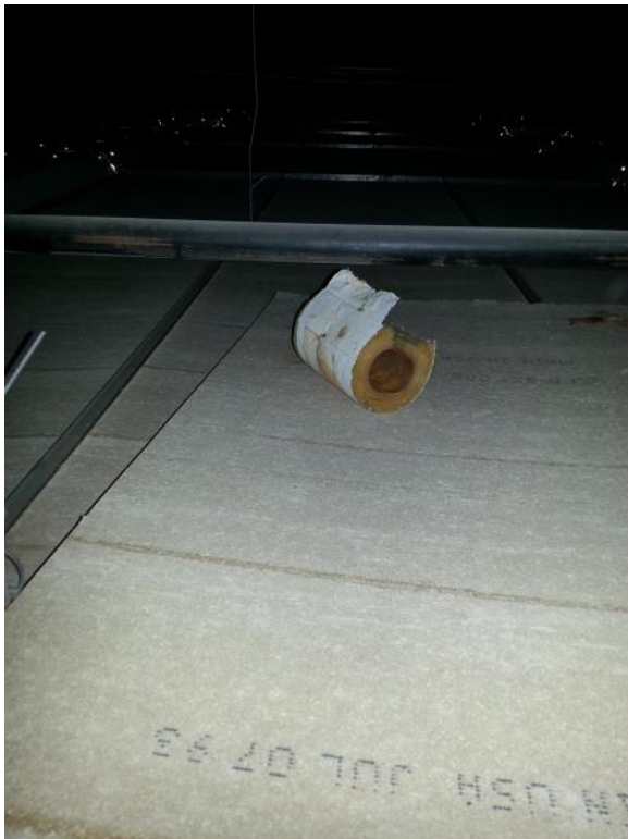
Photo 35 – Room 137 damaged pipe wrap
