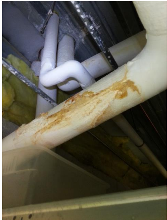
Photo 36 – Room 137 damaged pipe
