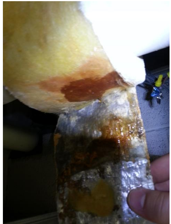
Photo 44 – Room 136 actively wet pipe covering
