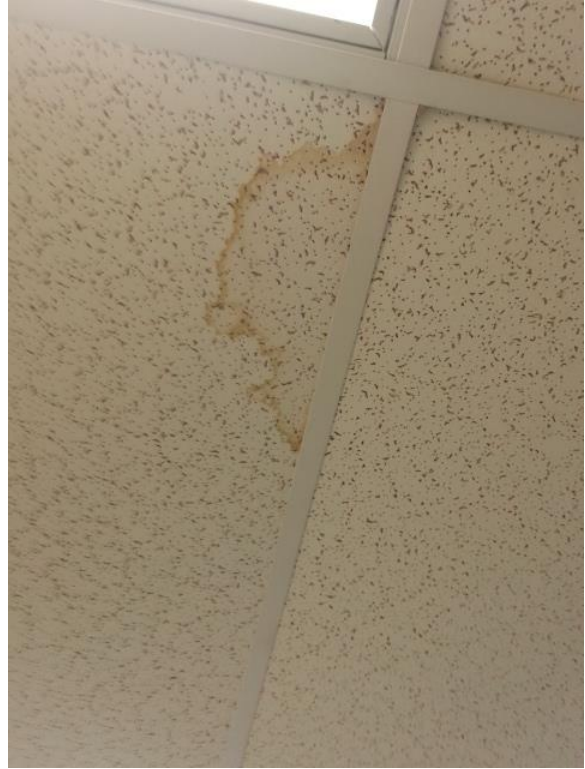
Photo 14 – Room 120 Stained Ceiling tile
