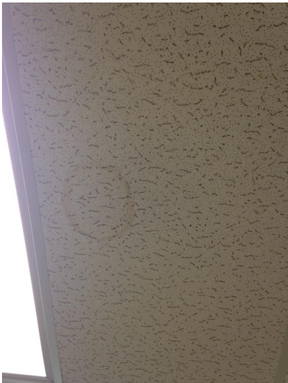
Photo 71 – Room 142, water stained ceiling tile
