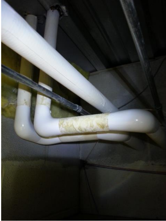
Photo 25 – Room 133 Stained Pipe Cover
