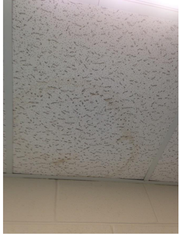
Photo 66 – Room 141, stained ceiling tile
