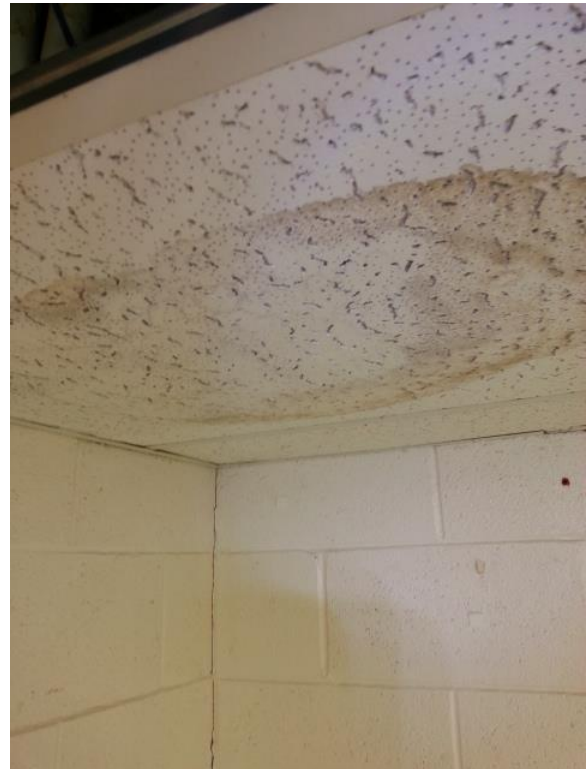
Photo 24 – Room 133 Stained ceiling tile
