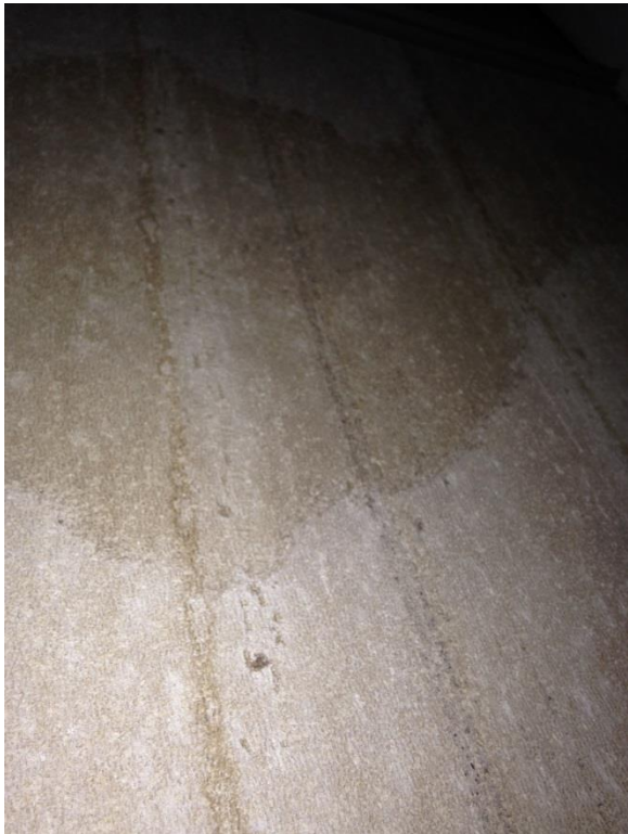
Photo 47 – Room 134 water stained ceiling tile
