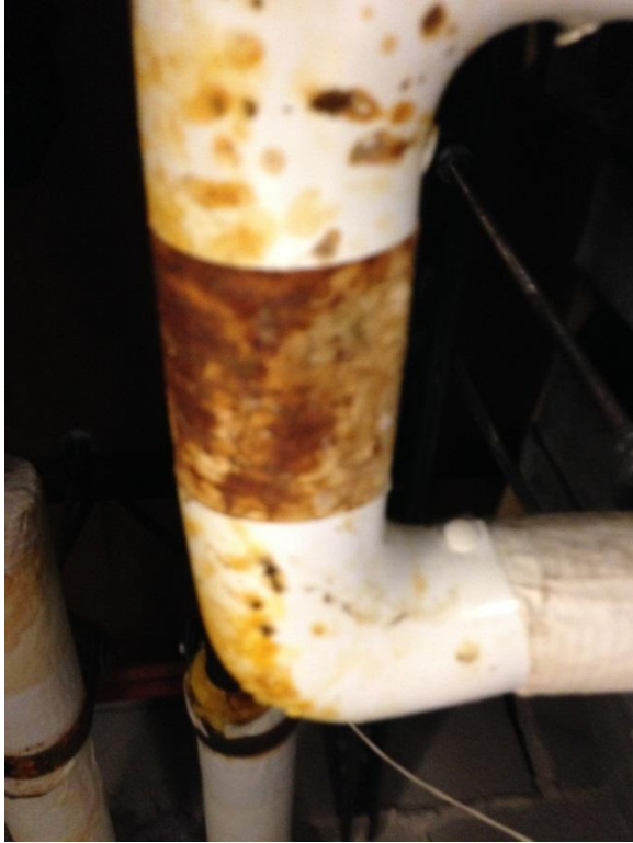
Photo 53 – Library Storage damaged pipe above ceiling tile
