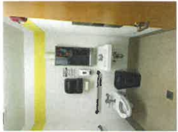
TYPICAL STAFF TOILET ROOM (MODULE B: T1 & T2)
