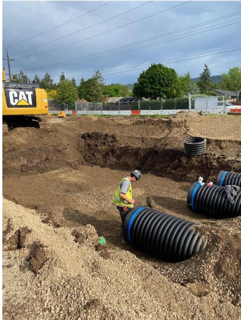
Underground Water Detention
