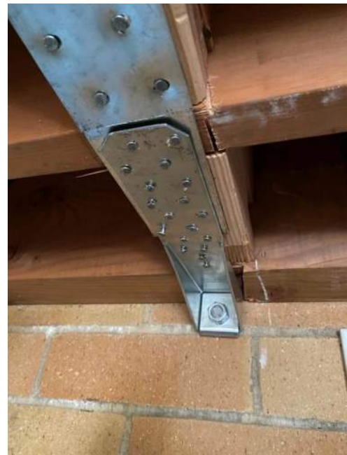
Library seismic strapping
