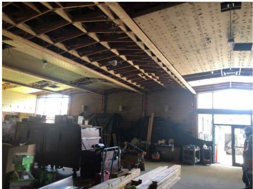
Library- all materials staged in library to minimize construction impacts on students and staff.
