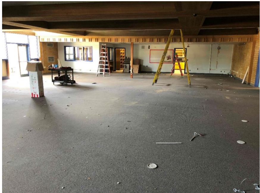
Library completely cleared
