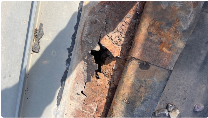
Photo showing metal roof deteriorating.
