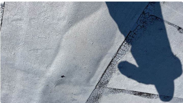
Photo showing additional blister.
