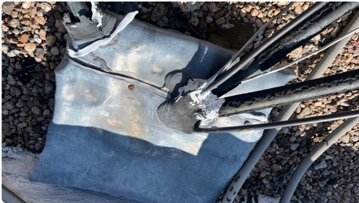
Photo showing lead around pitch pan with screws going into the portable sealer causing leaks to occur.
