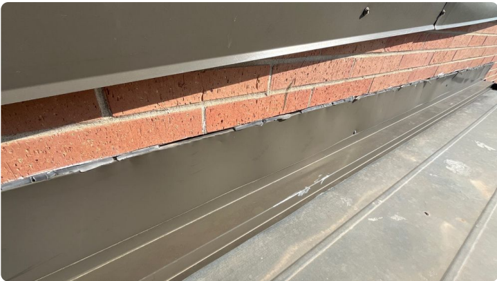
Photo showing sealant starting to deteriorate along the wall metal counter flashings.
