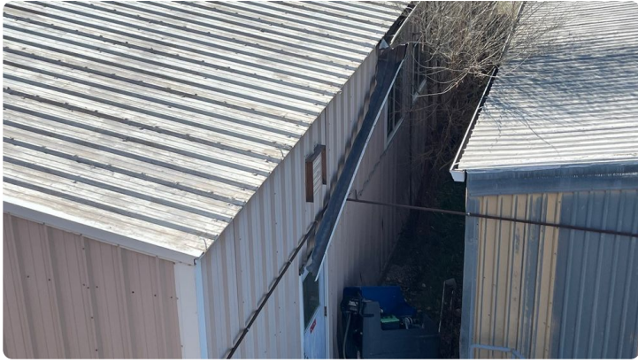
Photo showing additional overview of the detached gutter.
