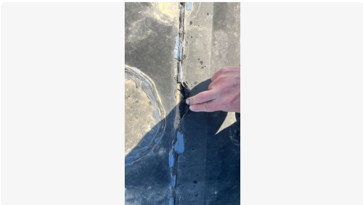
Photo showing field seam deteriorating and pulling loose.
