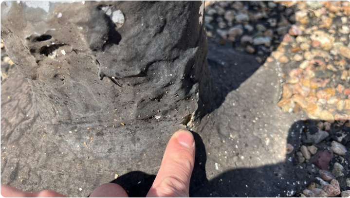
Photo showing a hole through the mastic and lead around soil stack.
