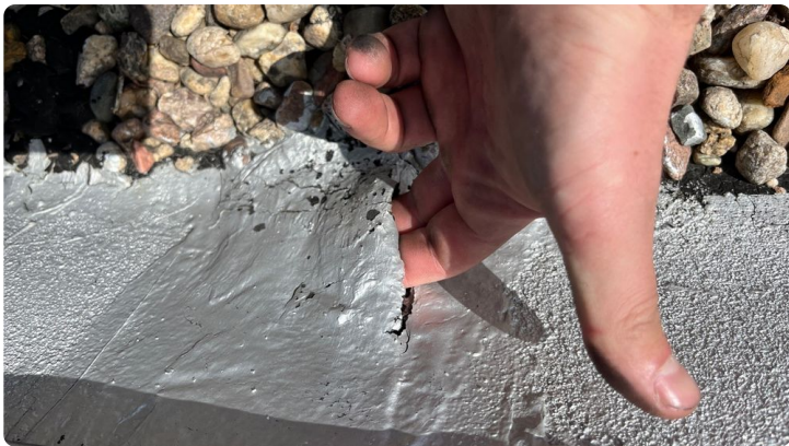
Photo showing vertical seam pulling loose.
