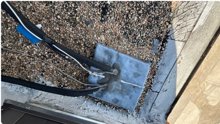
Photo showing lead covering pitch pan with screws going into the portable sealer.
