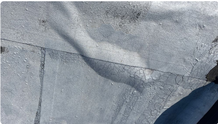
Photo showing blister in the membrane.
