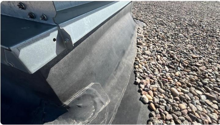
Photo showing tenting a long the projection flashings.
