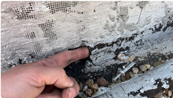
Photo showing vertical seam flashing opening up. Mesh is showing through all a long the perimeter without any mastic.
