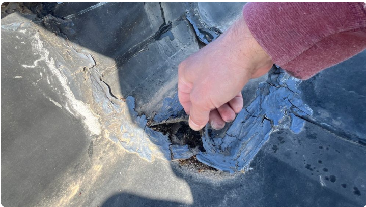
Photo showing vertical seam reinforcement patch pulling loose.
