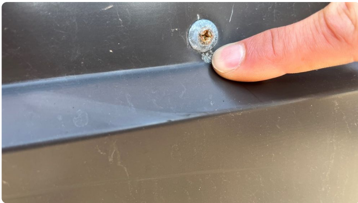
Photo showing a hole in the metal counter flashing causing a leak outside of the gym hallway.
