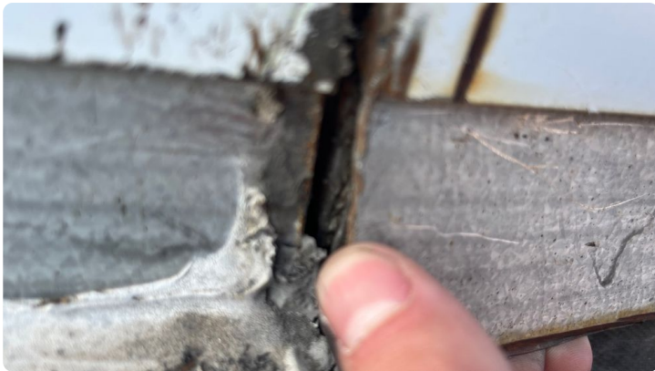
Photo showing poor counter flash detail a long wall where the end cut went through the EPDM flashings and left exposed.
