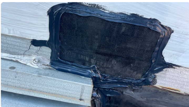
Photo showing repaired made to the counter flashings leak.
