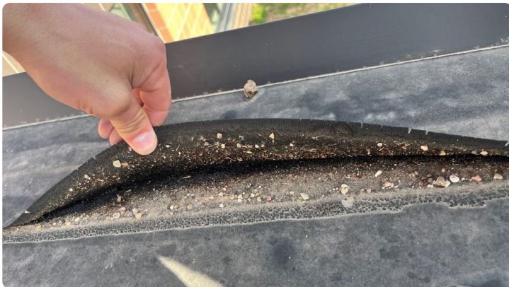
Photo showing form flashing pulling up.
