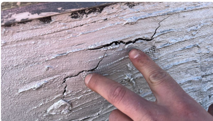
Photo showing a split in the perimeter flashings that appear to be through the coating and membrane.
